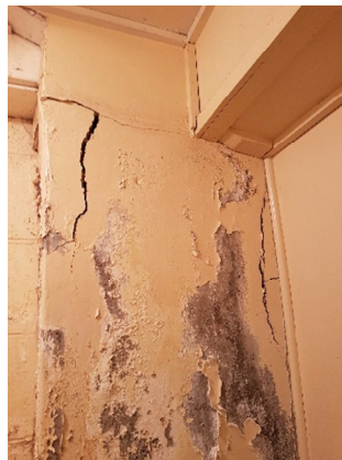
Photo 2: Cracking to Concrete Encasement
