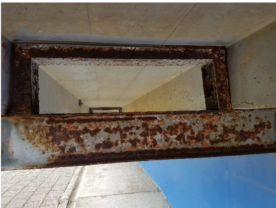
Photo 1: Corroded Steel Section
