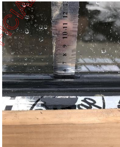
Figure 6 – Pane 1, Interior Glazing Seal
