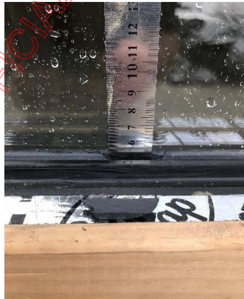
Figure 6 – Pane 1, Interior Glazing Seal
