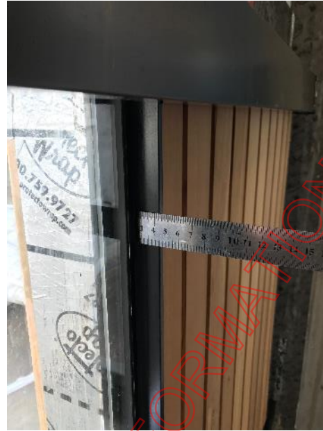
Figure 4 – Pane 1, Right Jamb Seal
