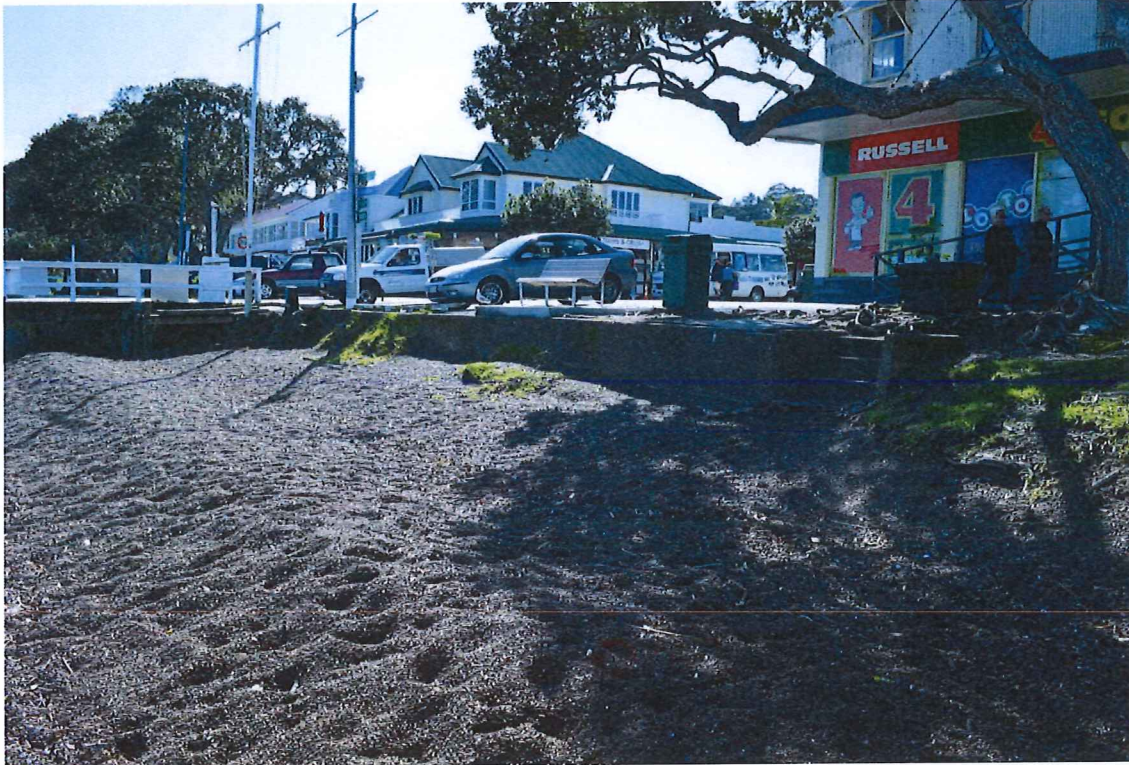
Plate 13: The current concrete retaining wall located to the immediate south of the Russell wharf
