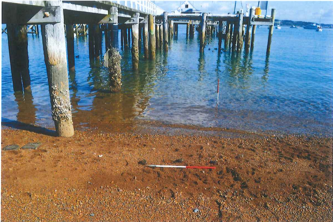
Plate 14: The small timber piles located at the low tide mark to the north of the current Russell wharf
