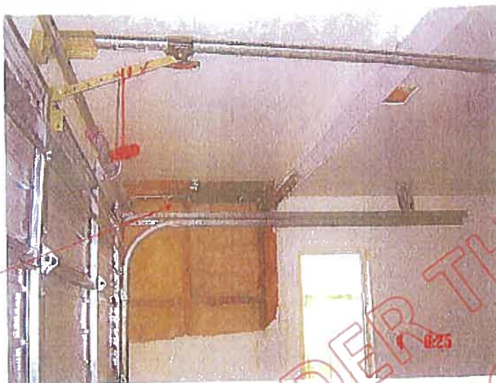
Location of cut out showing decayed metal
