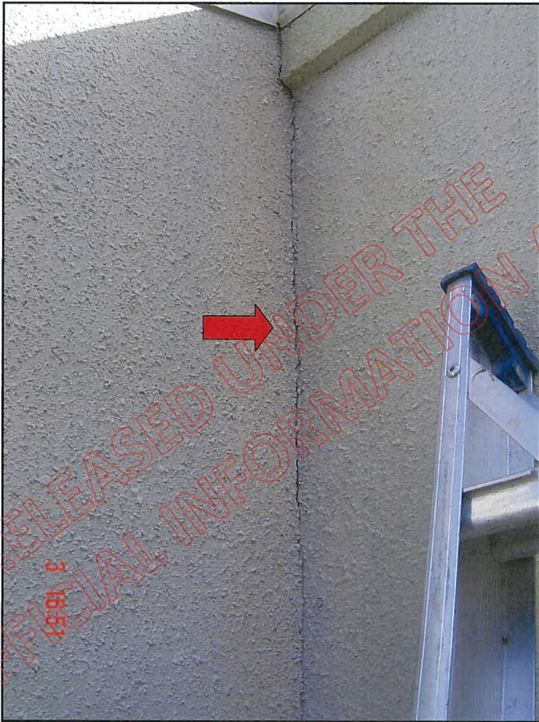
Vertical cracking at east wall / wing wall junction; allows moisture ingress
