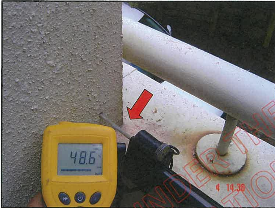
Very high probe moisture reading above balcony capping – wing wall junction; note no saddle flashing at this junction, note incorrect installation of hand rail stanchion
