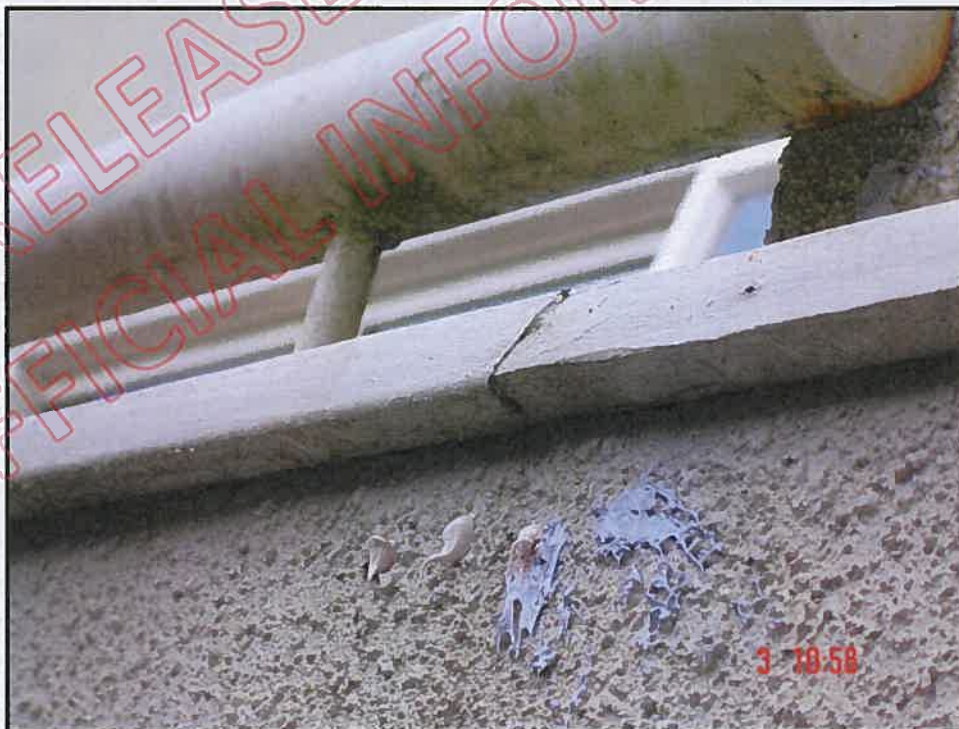
Open and unprotected spliced joint in timber capping
