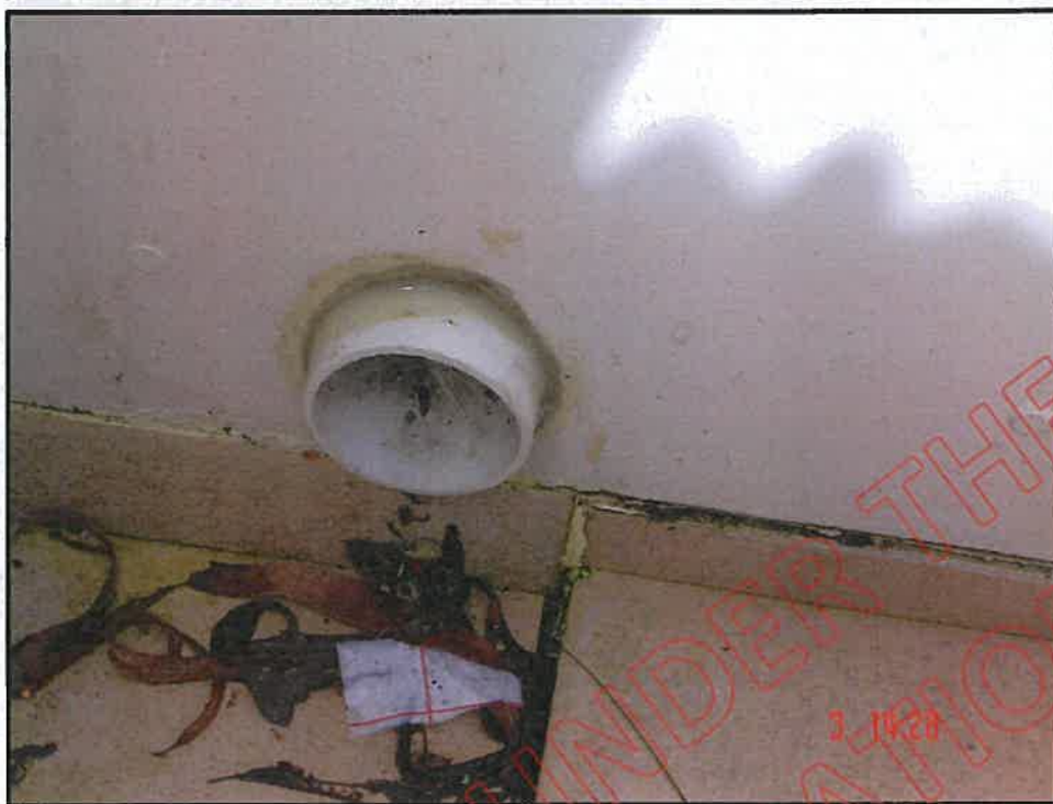
Inadequately designed and fitted balcony drainage overflow
