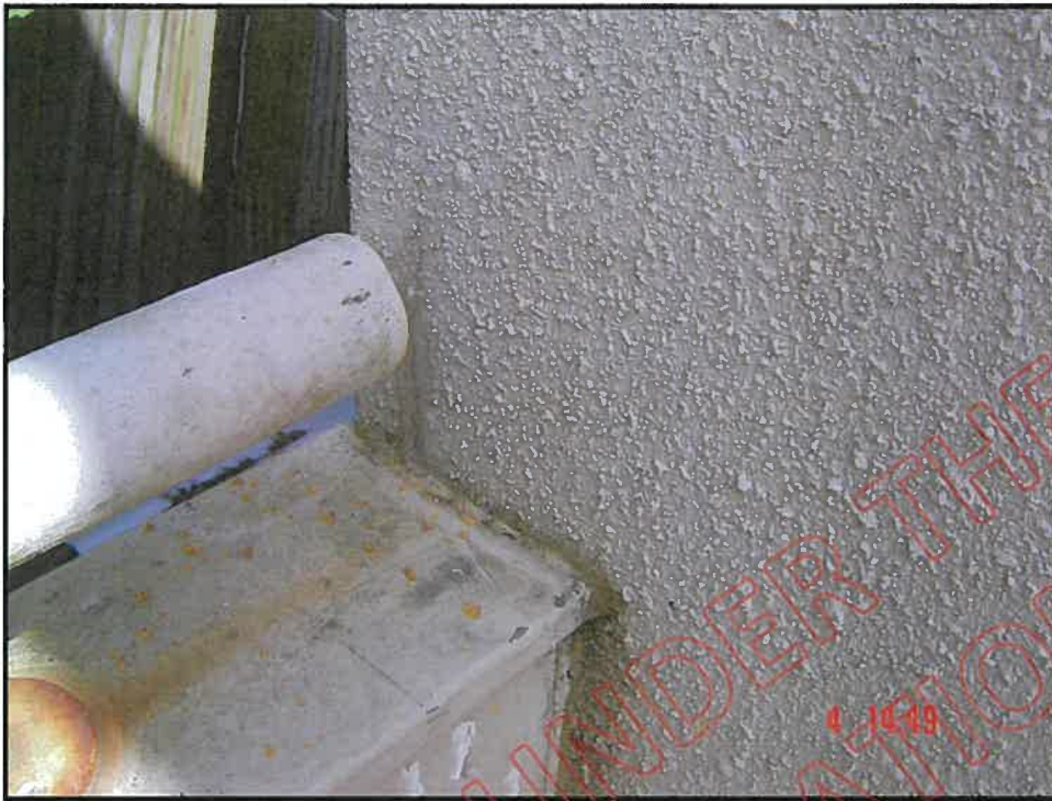
North wall – balcony wall junction (note: no saddle flashing at junction).
