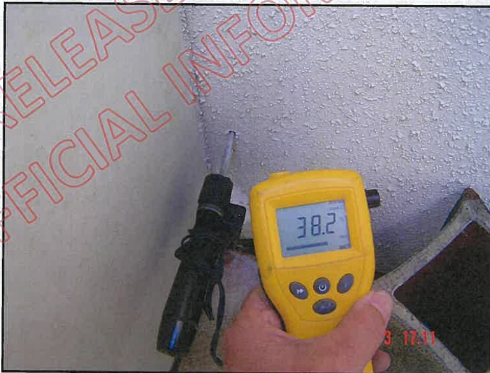
High probe moisture reading at base of wing wall/balcony junction
