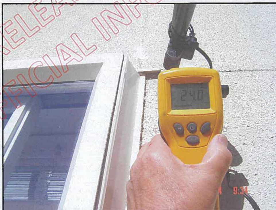
High probe moisture reading at right side of balcony sliding door head flashing; refer photograph 1d 21
