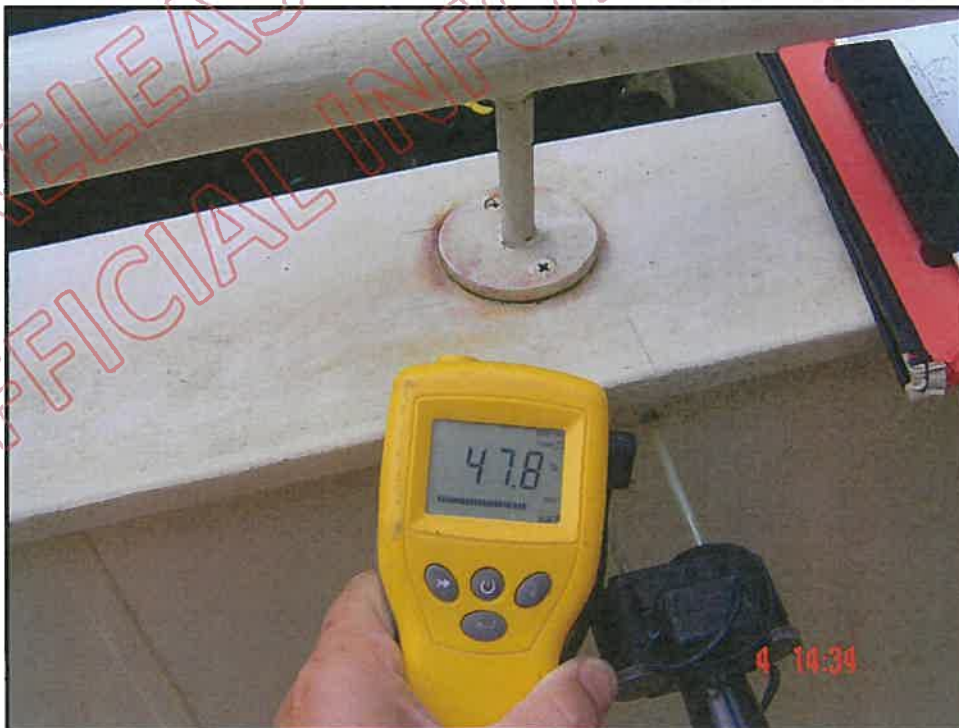
Very high probe moisture reading at centre of eastern balcony wall; note incorrect installation of hand rail stanchion
