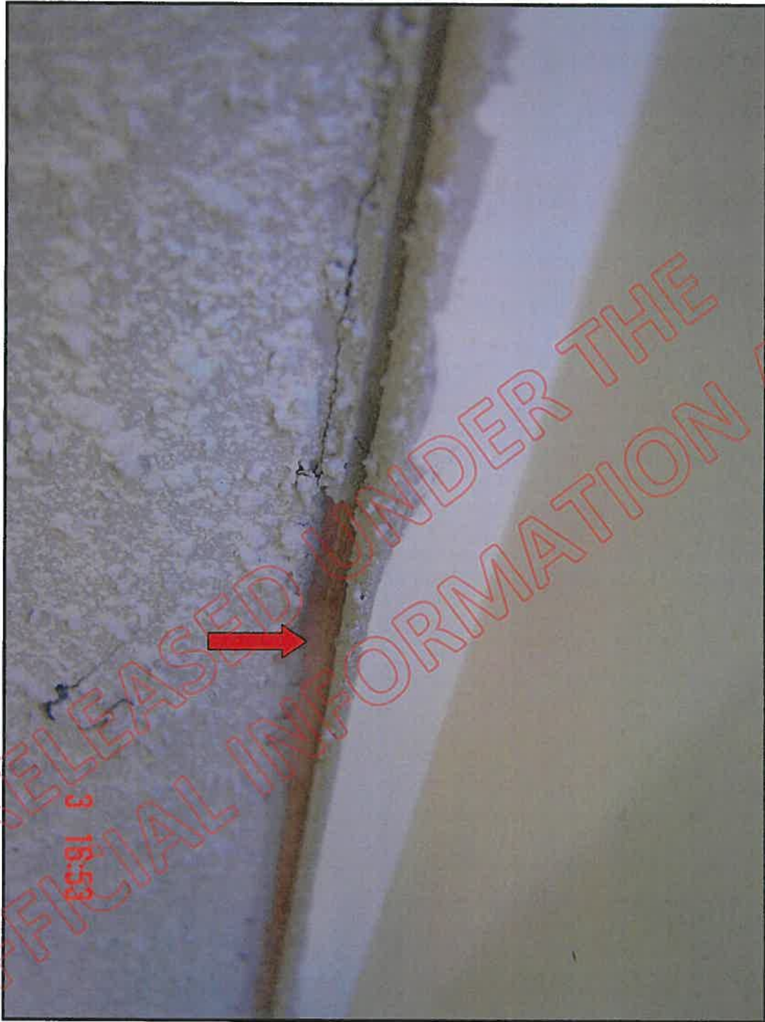
Total joint failure at balcony door jamb, left hand side; note no flashings, seals and raw Harditex
