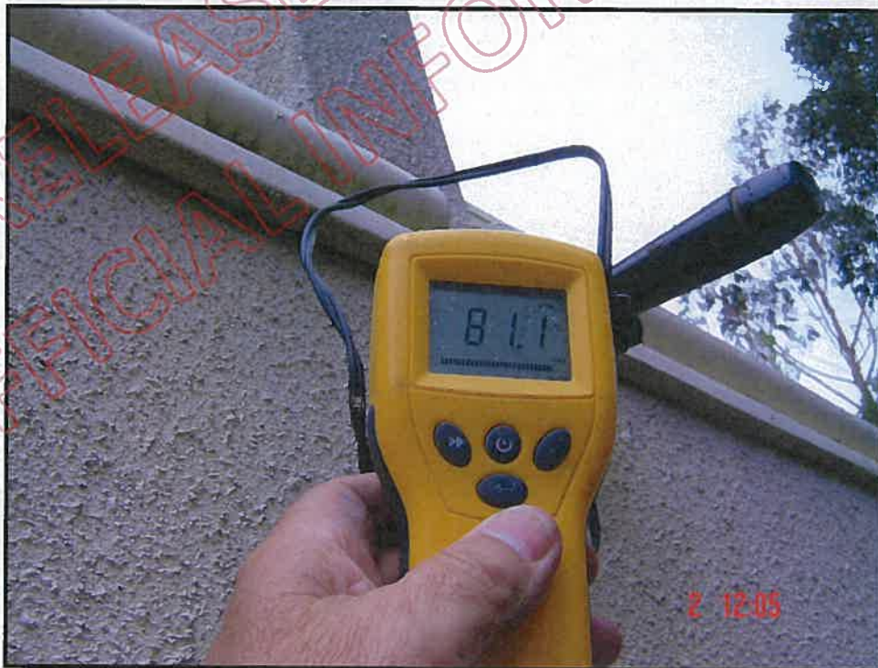
Very high probe moisture reading at eastern face of balcony wall at wing wall
