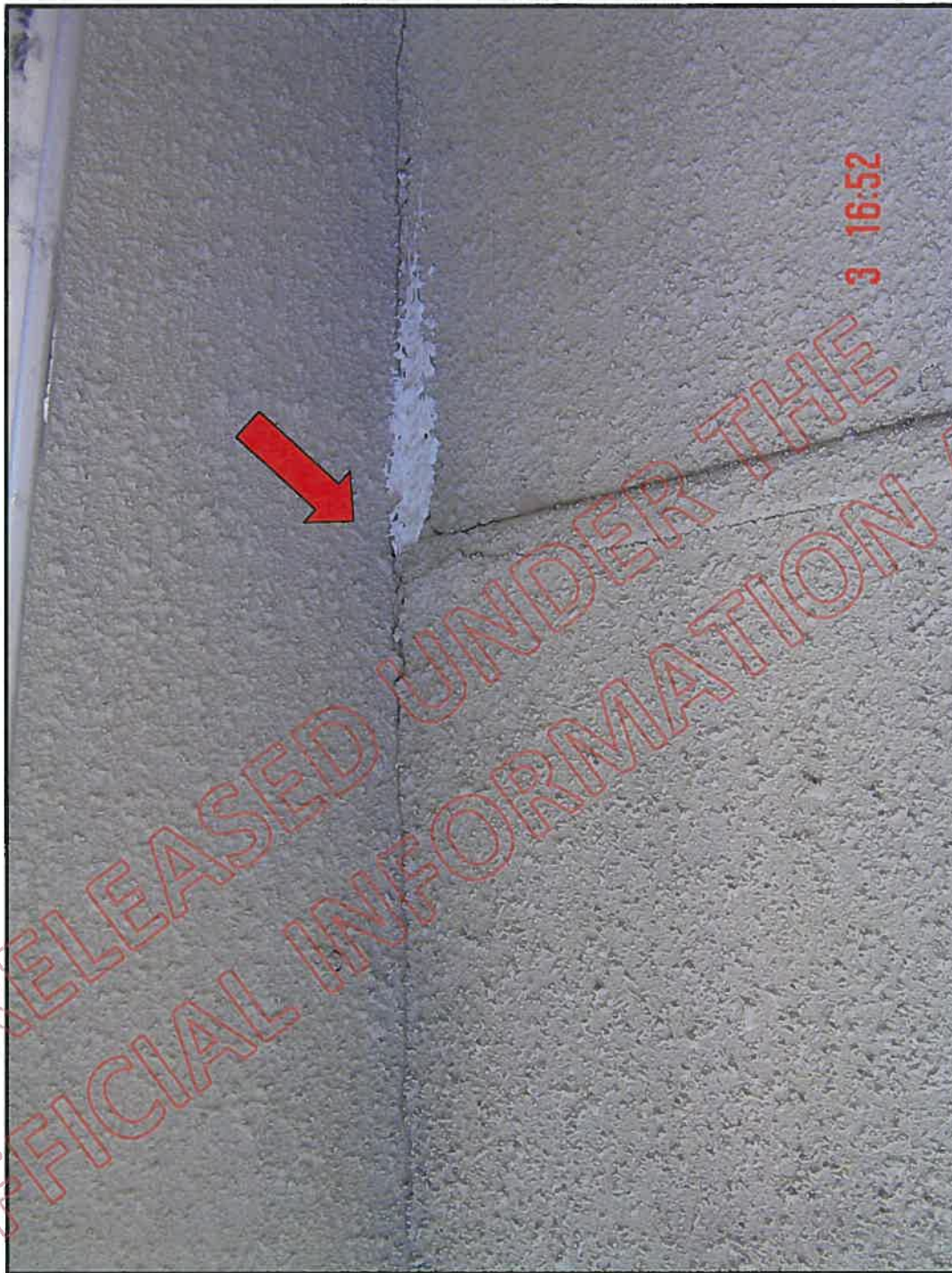
Vertical cracking at east wall / wing wall junction: note inter-storey joint terminates at wing wall face, allows moisture ingress
