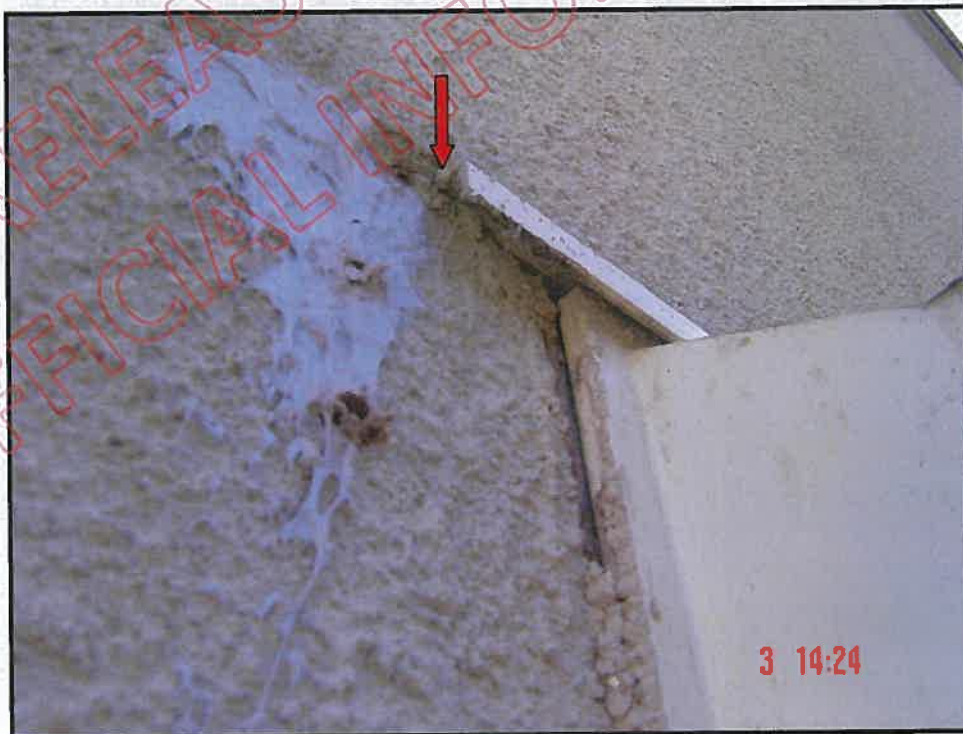
Inter-storey joint butts up to balcony door head flashing left hand side; Open joint is allowing moisture ingress
