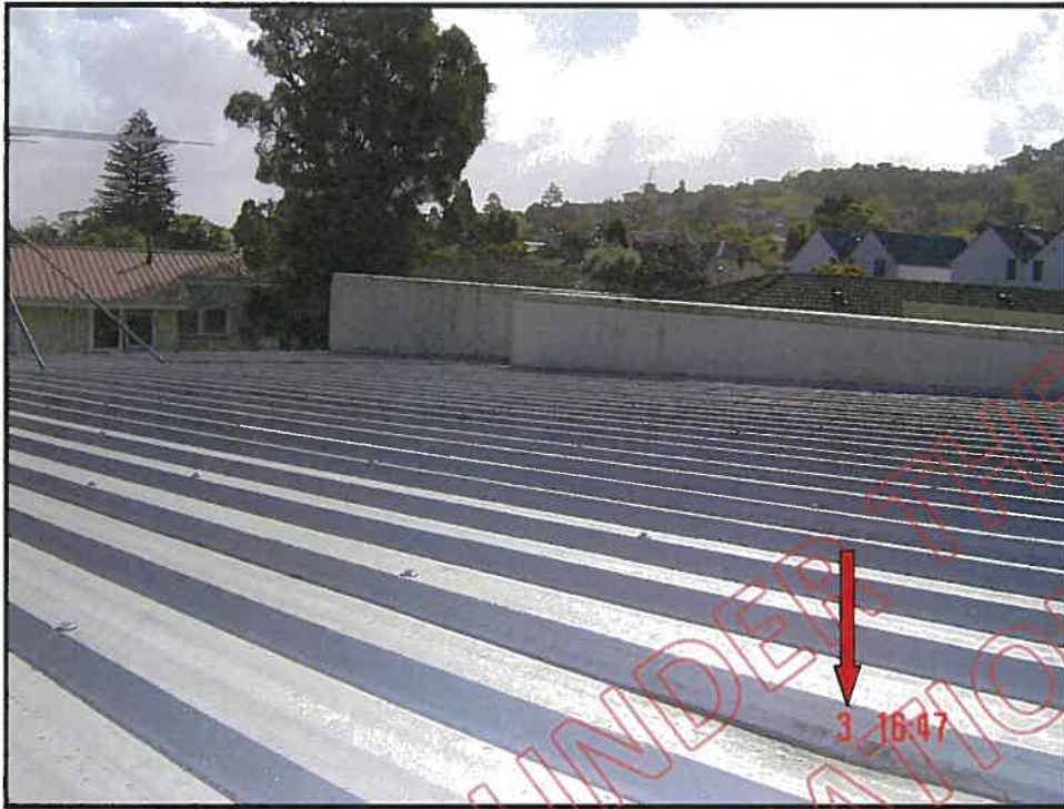
General view of roof units D and E showing damage to the profile due possibly to incorrect walking
