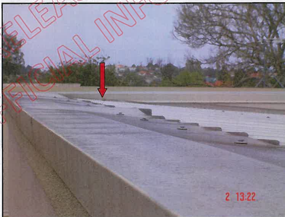
General view of unit C roof showing insufficient height to east and side parapet walls
