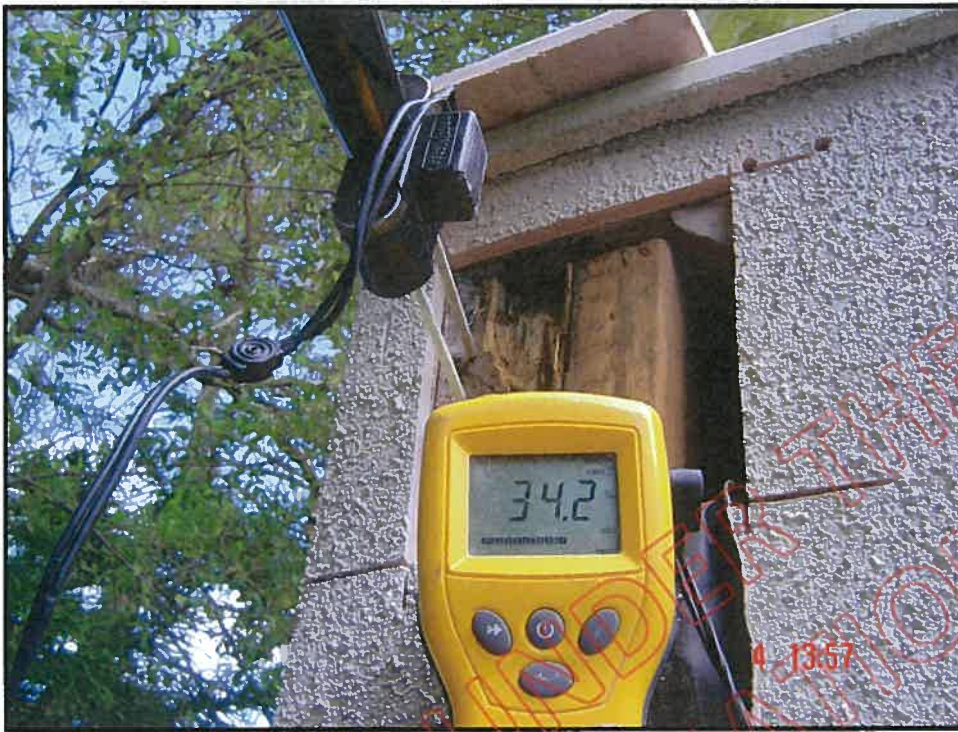
Cut out and probe reading at south east corner of balcony wall (Laboratory sample 9)
