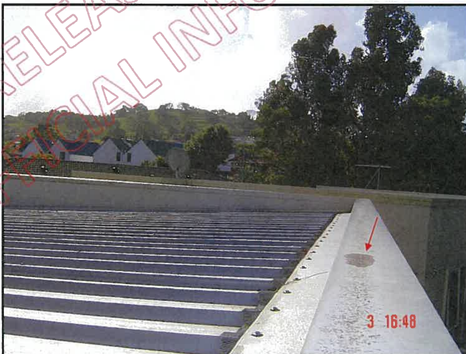
General view of roof unit D: note water ponding on flat cap flashing
