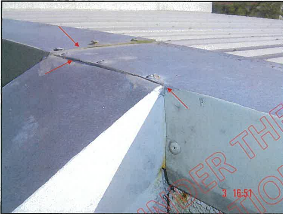
Badly designed cap flashing / wing wall flashing: note corrosion at and below vertical joint
