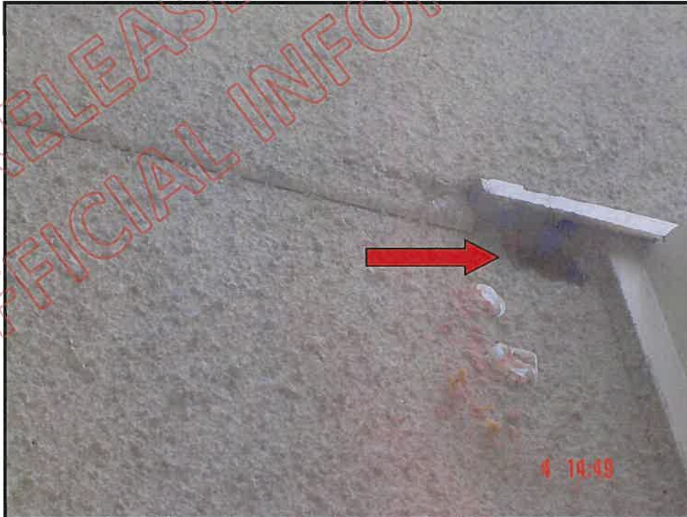
Incorrectly placed inter-storey joint butting into balcony door head flashing; note gap at join and hole with bare harditex under head flashing
