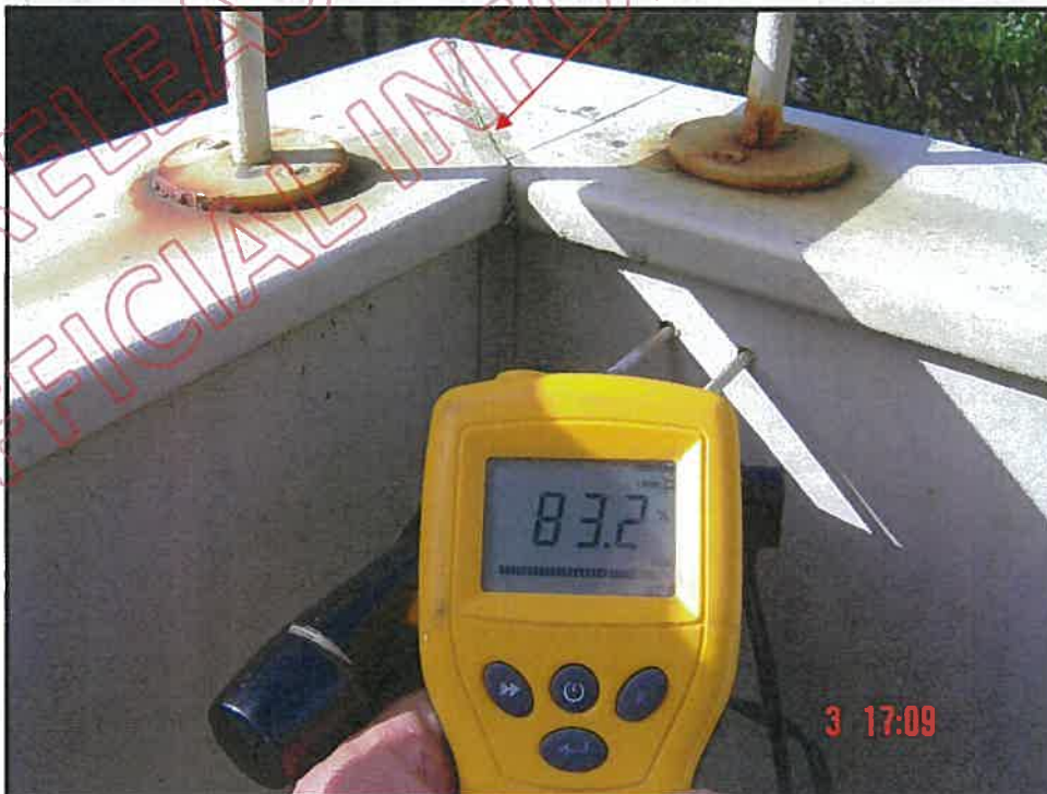
Very high probe moisture reading at north east corner balcony wall junction (note: open and unprotected mitre joint); note also corroded handrail stanchion and incorrect application
