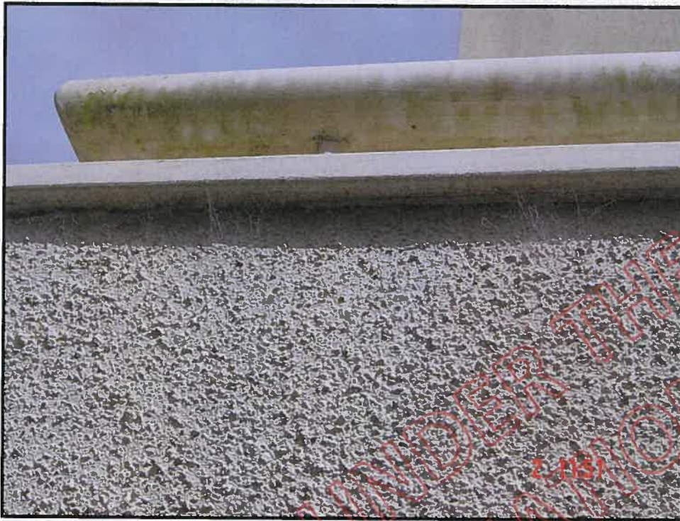
Looking up under timber balcony wall cap: note junction not sealed
