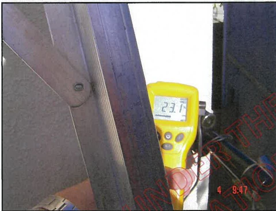
High probe moisture reading at north end of east wall 200mm below fascia
