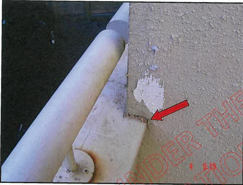
Close up of wing wall balcony wall cap junction showing point of water entry
