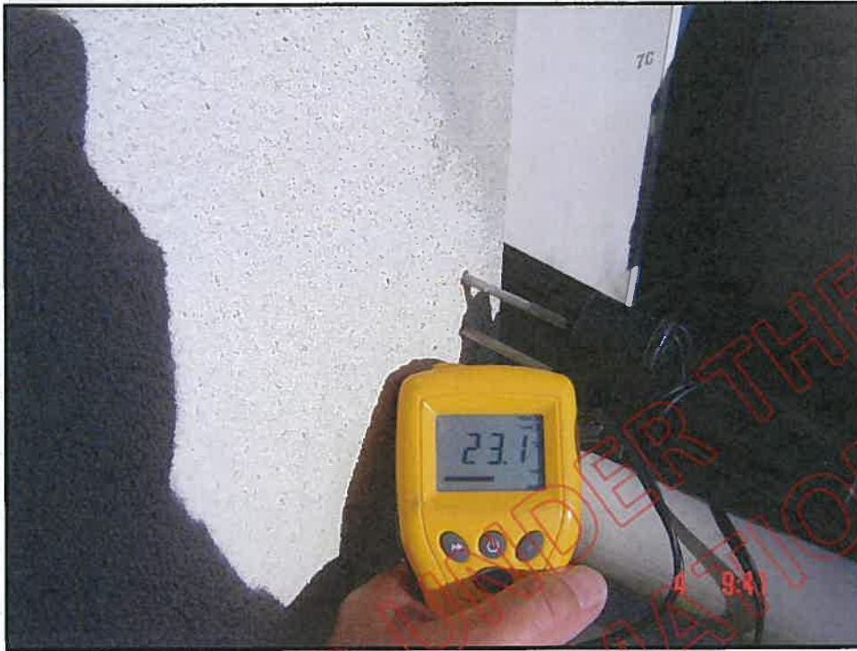
High probe moisture reading at north end of east wall above balcony wall hand rail
