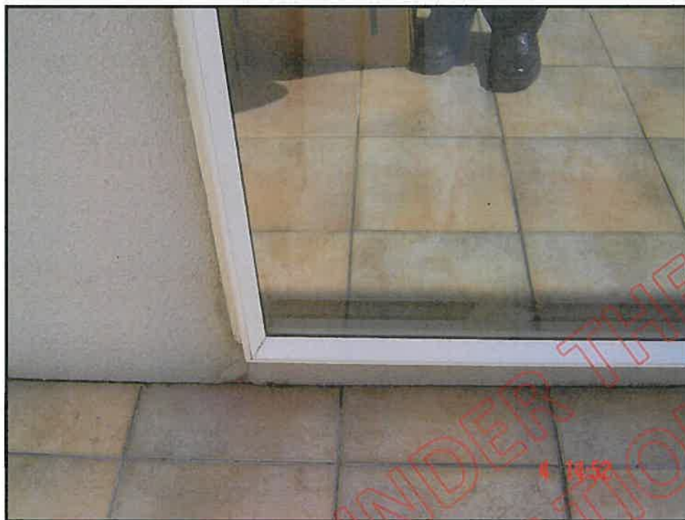
East wall shows cladding finishing hard down onto tiled balcony floor
