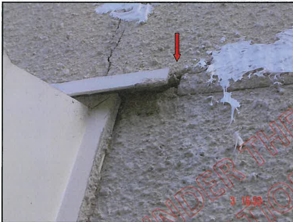
Inter-storey joint butts up to balcony door head flashing right hand side; Open joint is allowing moisture ingress
