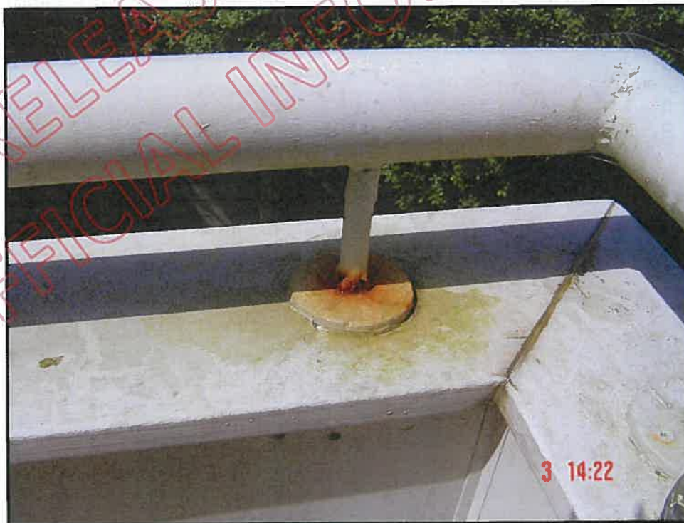
Close up of open and unprotected mitre joint at south east corner of balcony wall); note also corroded handrail stanchion and incorrect application
