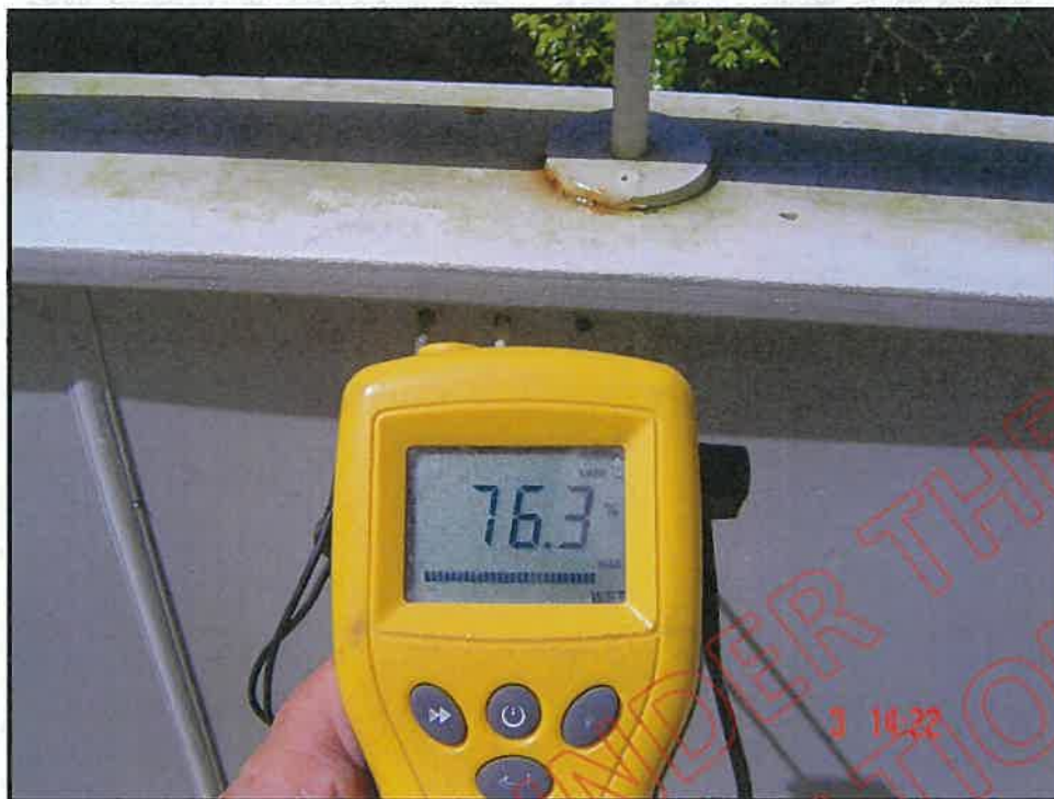
Very high probe moisture reading at centre of balcony wall
