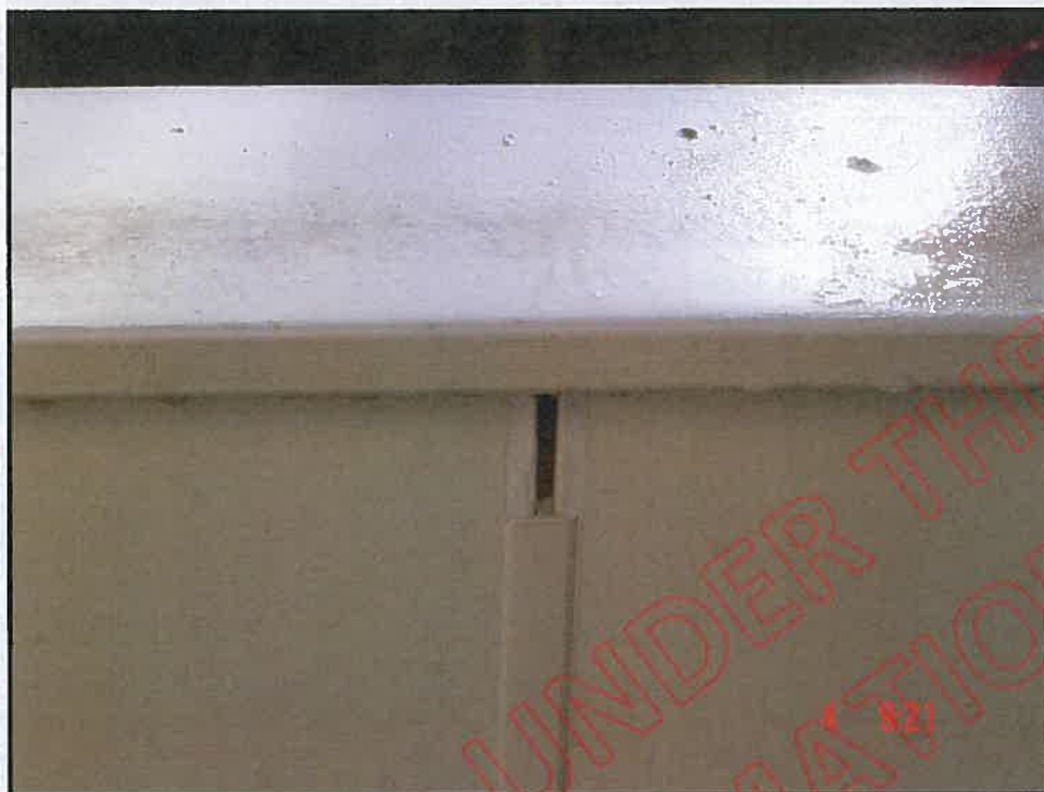
Photograph showing poorly fixed jointer, jointer has dropped and allowing moisture ingress
