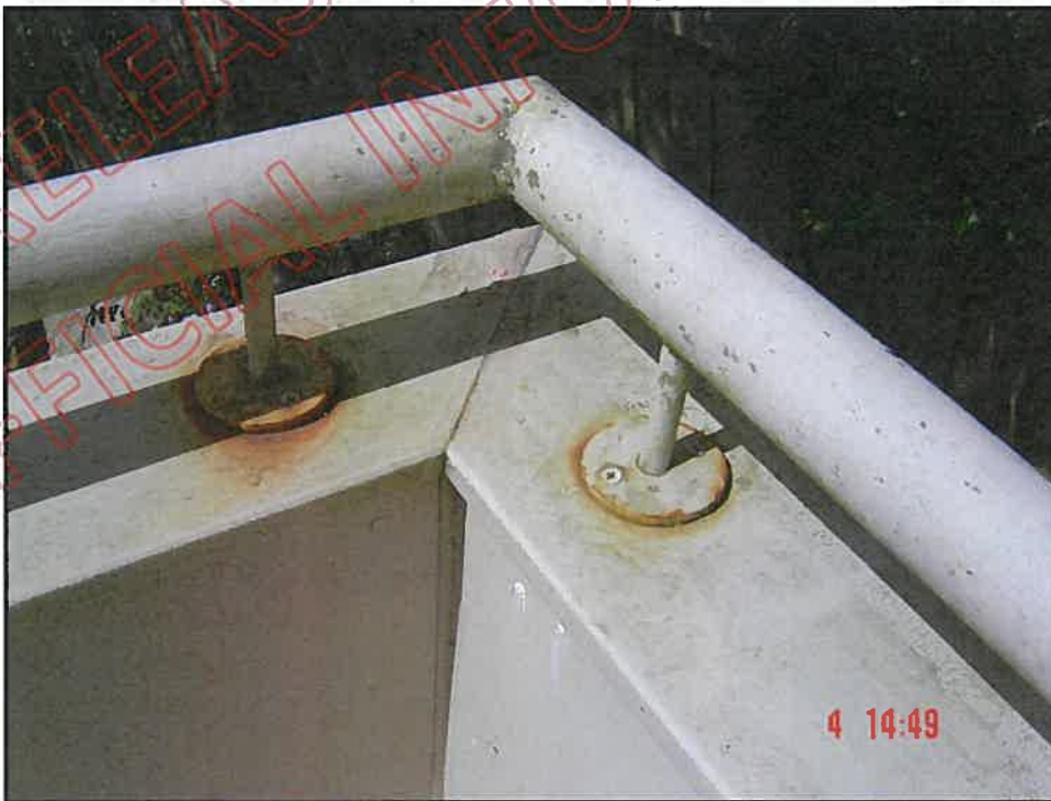
Top of balcony wall at south east corner; note corroded hand rail stanchions and open mitre to timber capping, mitre has no weather protection
