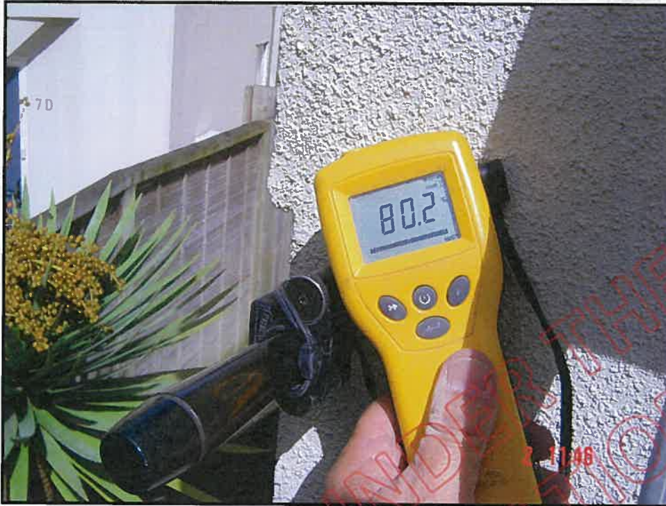
Very high probe moisture reading at north east corner balcony wall adjacent to garage door head, right hand side
