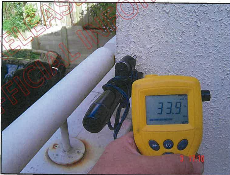
Very high probe moisture reading above wing wall balcony wall junction
