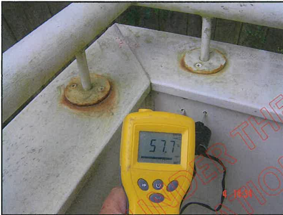
Very high probe moisture reading at south east corner of balcony wall
