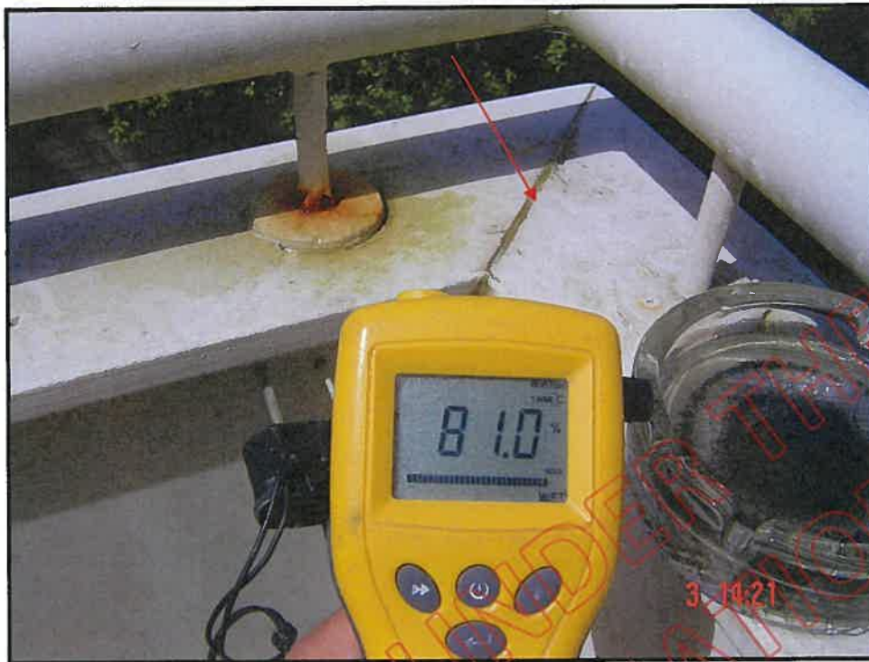
Very high probe moisture reading at south east corner balcony wall junction (note: open and unprotected mitre joint); note also corroded handrail stanchion and incorrect application
