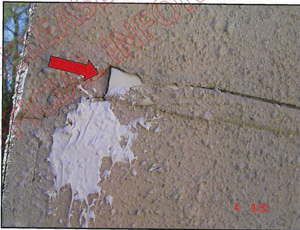
Close up of wing wall balcony showing inter-storey moulding open end, point of water entry; note joint failure below inter-storey; refer photograph (d27)
