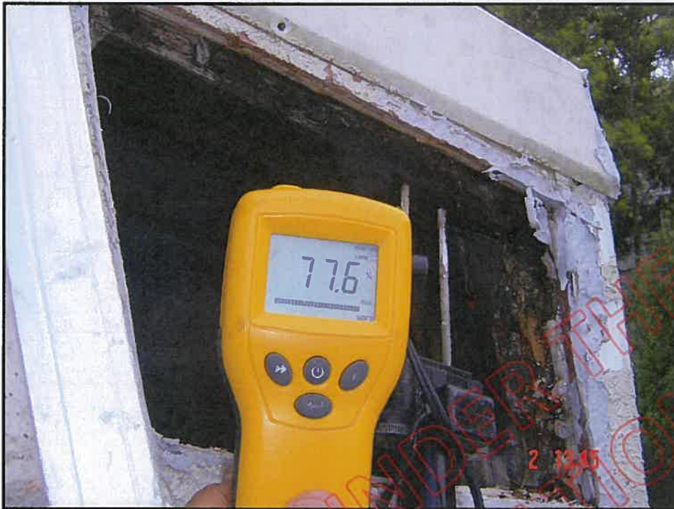
Cut out and very high probe moisture reading at top front corner of wing wall showing advanced decay; point of water entry is poorly designed and fitted wing wall cap flashing
