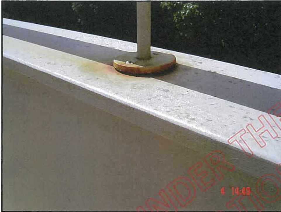
Eastern balcony wall showing incorrectly installed corroded hand rail stanchions
