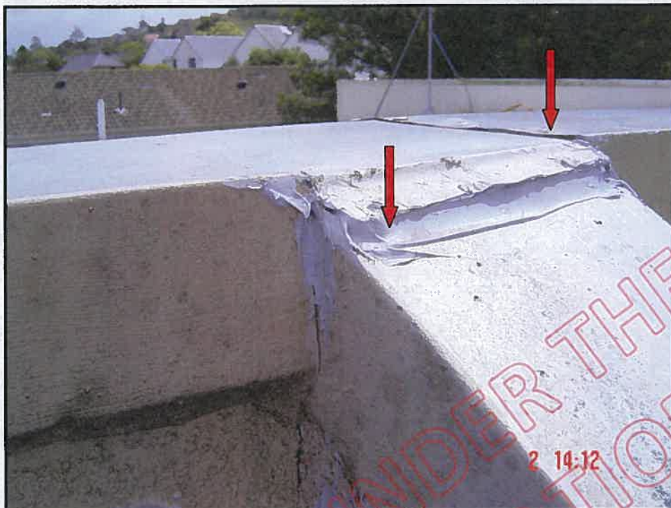
Badly designed cap flashing / wing wall flashing: note copious amount of exposed sealant applied in an attempt to achieve weathertightness, note also open lap joint
