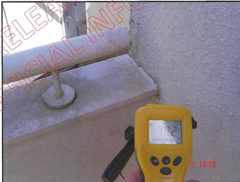
Very high probe moisture reading at balcony wall / wing wall junction: note no saddle flashing at balcony / wing wall junction
