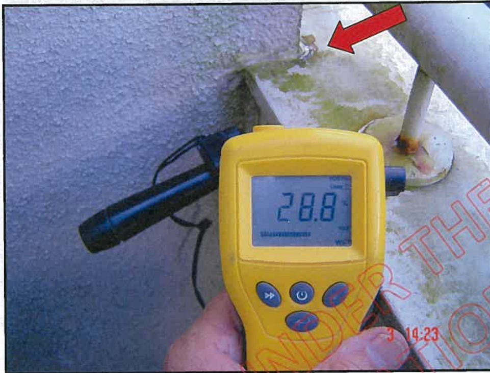
Very high probe moisture reading top of balcony wall adjacent to the wing wall; note no saddle flashing at balcony / wing wall junction
