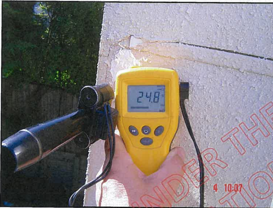
High probe moisture reading below inter-storey at front face of wing wall: note inter-storey joint terminates at mid sheet: end of mould is open allowing moisture ingress
