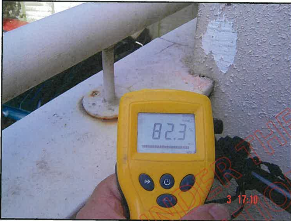
Very high probe moisture reading at wing wall balcony wall junction (note: no saddle flashing at junction); note also corroded handrail stanchion and incorrect application
