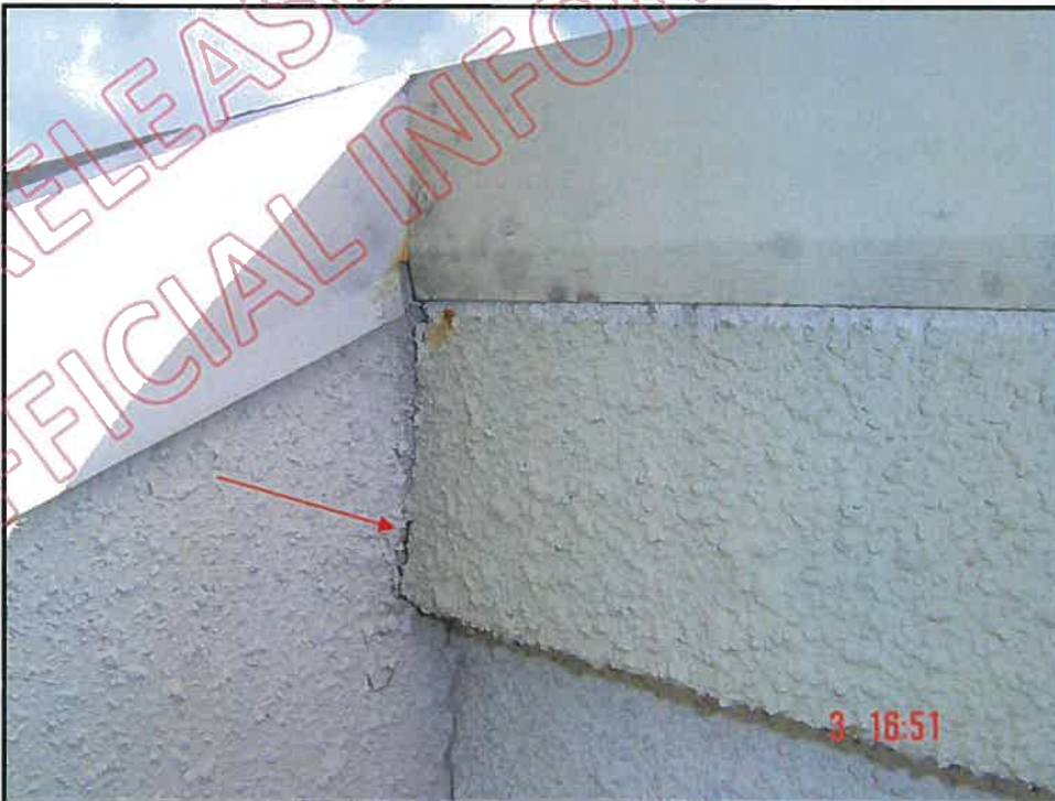
Open joint where timber fascia abuts wing wall cladding
