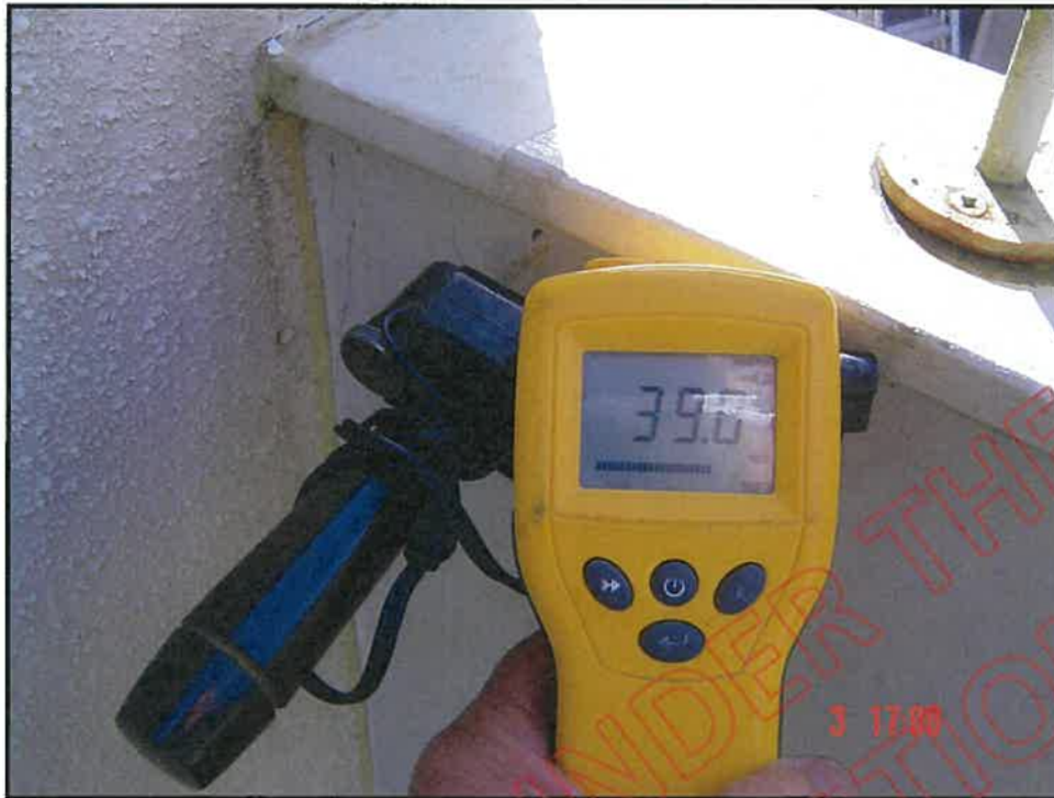
Very high probe moisture reading at east wall balcony wall junction (note: no saddle flashing at junction); note also corroded handrail stanchion incorrect application
