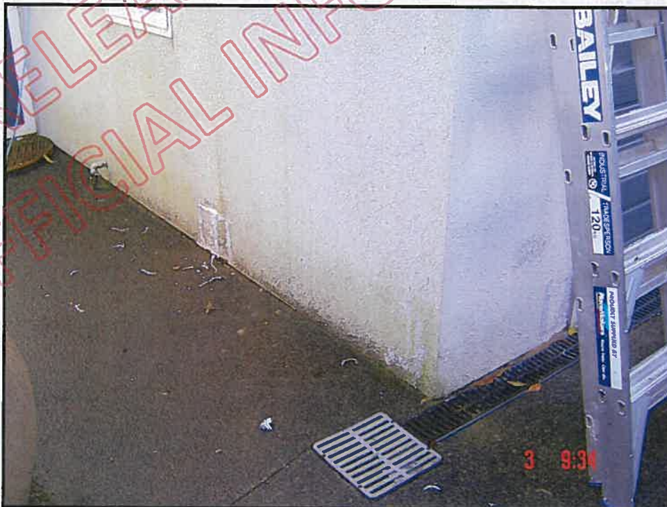
Photograph showing cladding extending to paving; should have minimum of 100mm clearance
