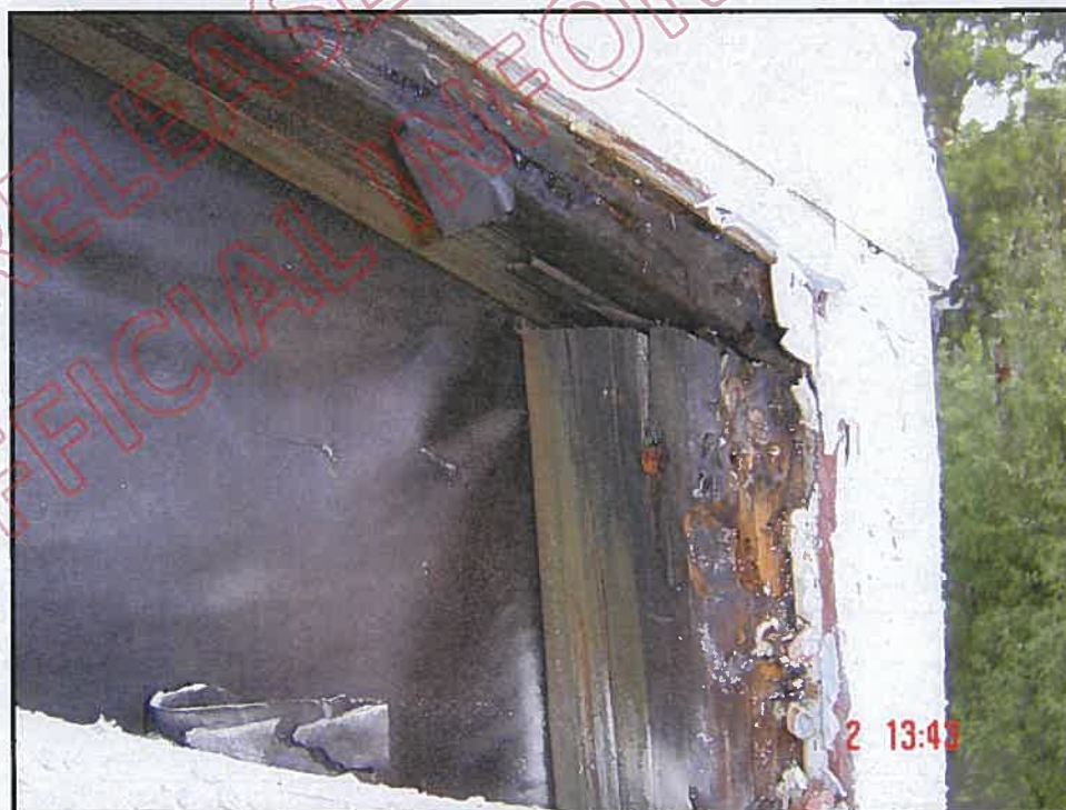
Cut out at top front corner of wing wall showing advanced decay; refer laboratory sample (3)
