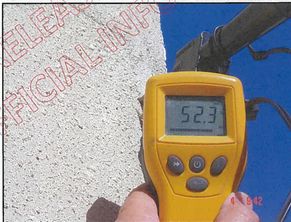
Very high probe moisture reading at north end of east wall 600mm below fascia
