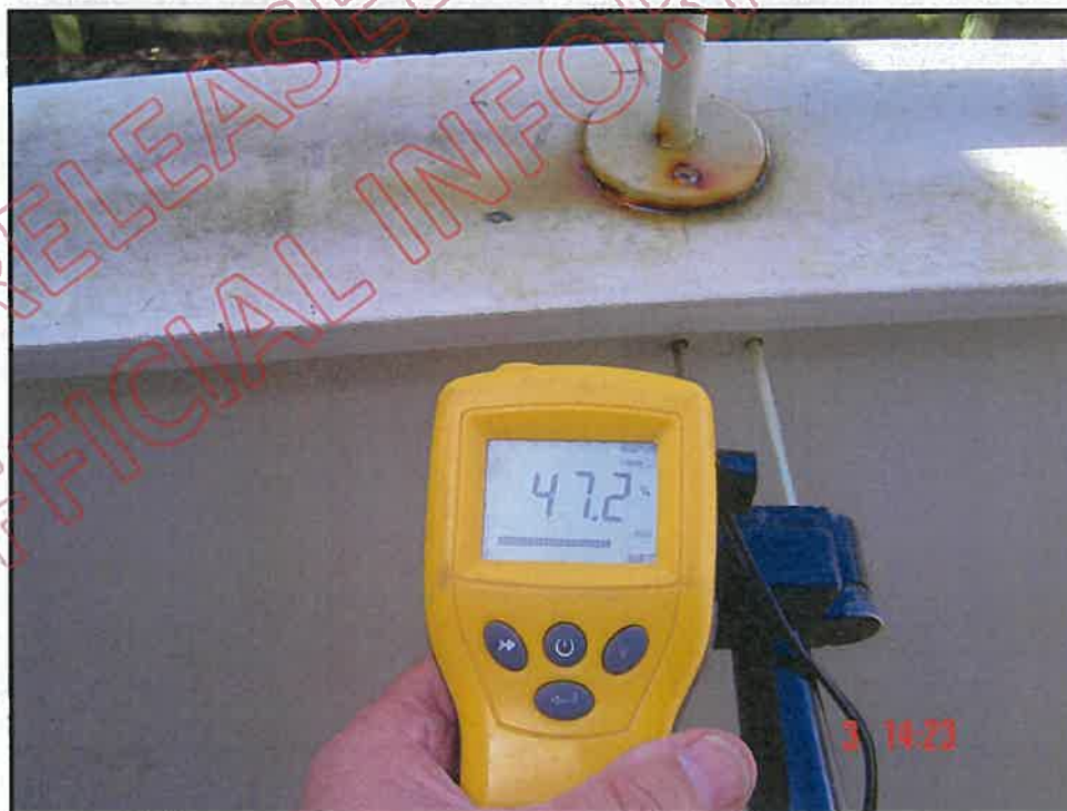
Very high probe moisture reading near to the centre of balcony wall
