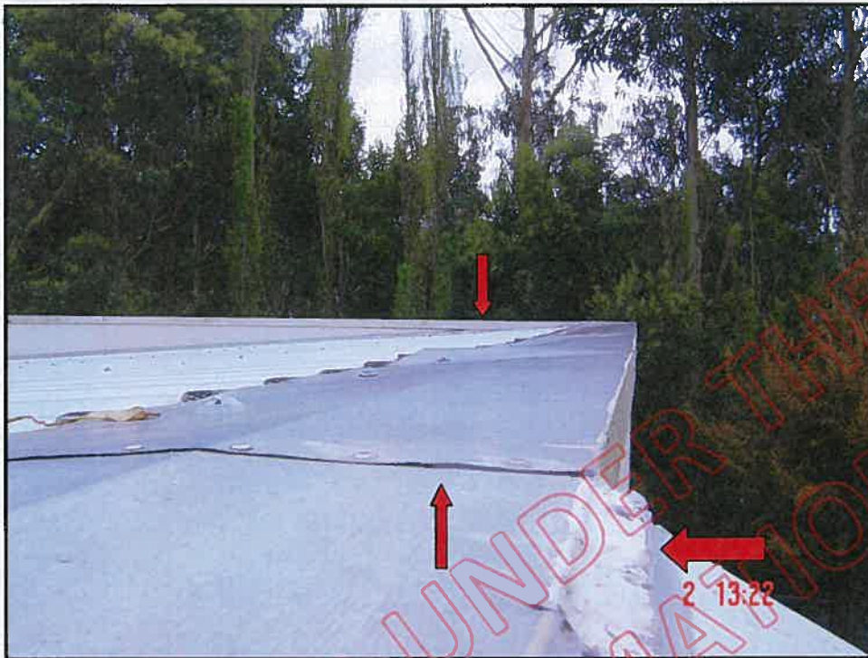
General view of unit B roof showing insufficient height to east and side parapet walls; note also poor cap joints
