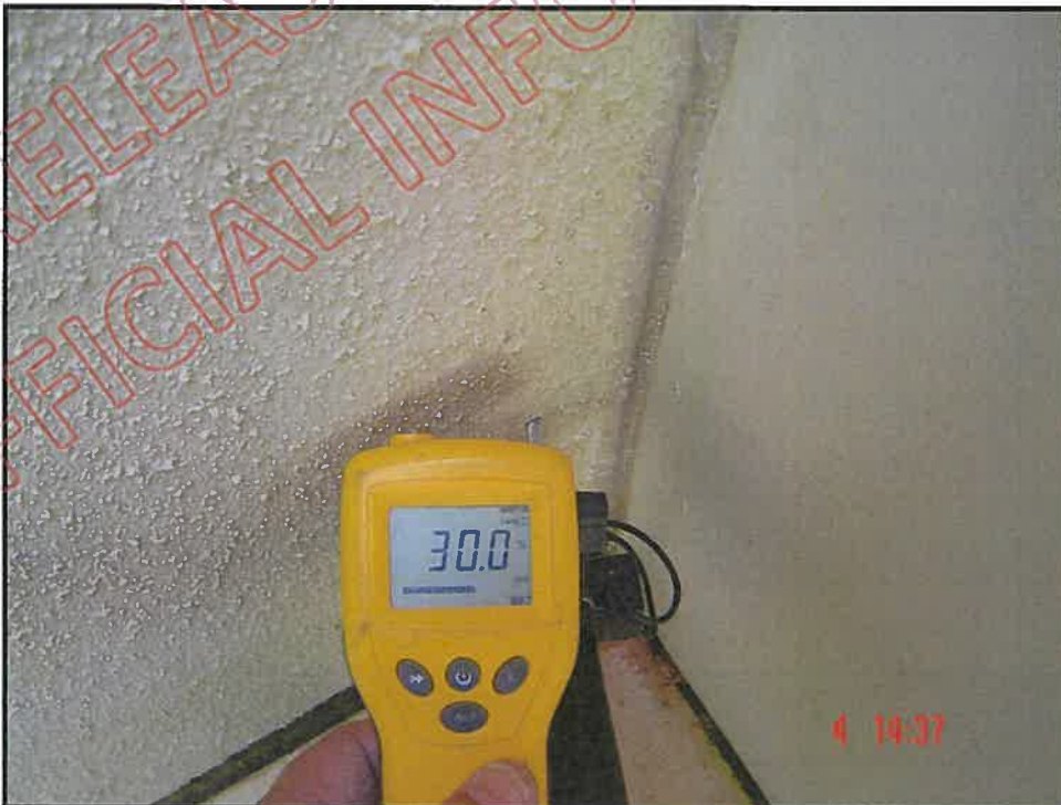
Very high probe moisture reading at base of wing wall; note cladding has insufficient clearance above tiled balcony floor
