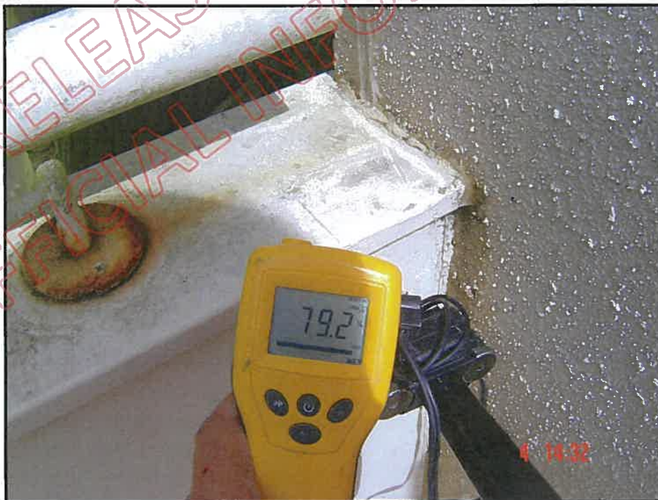
Very high probe moisture reading at east wall balcony wall junction (note: no saddle flashing at junction); note also corroded handrail stanchion incorrect application
