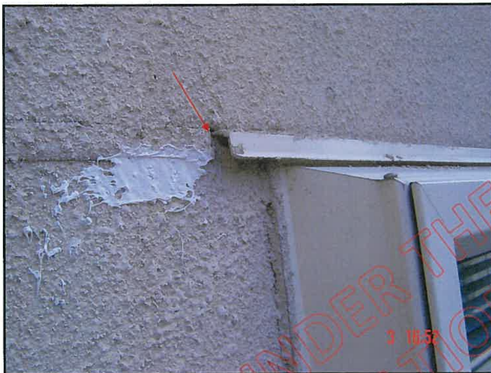
Inter-storey joint butts up to balcony door head flashing left hand side. Open joint is allowing moisture ingress
