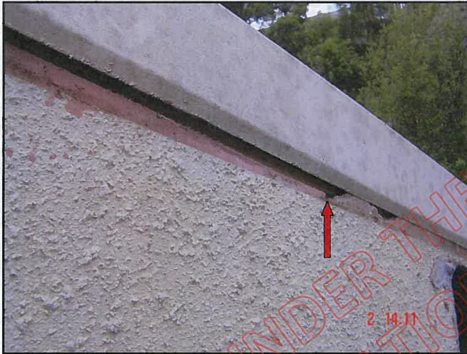
Wing wall cap flashing showing cap barely covering Harditex; note wall should be textured prior to fitting cap flashing, Harditex not sealed at sheet edges as required
