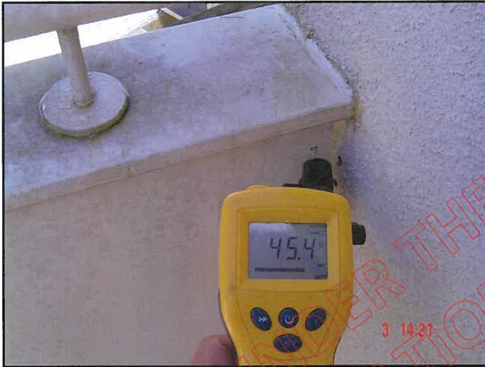
Very high probe moisture reading at east wall / wing wall junction: note no saddle flashing at balcony / wing wall junction
