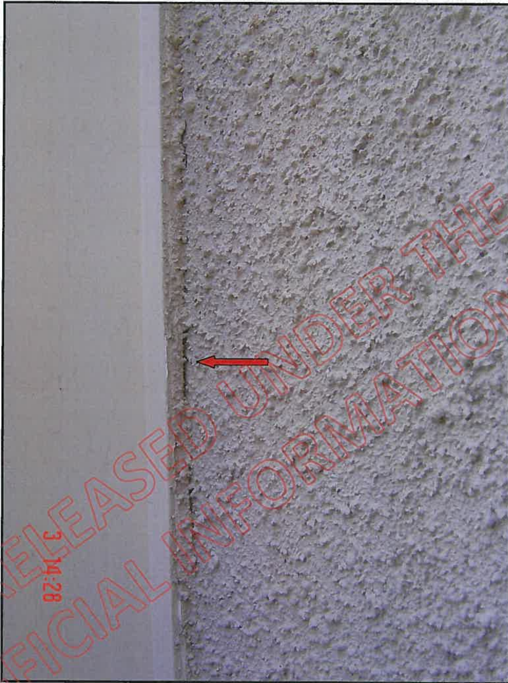
Failed jamb seal at right hand side of balcony door
