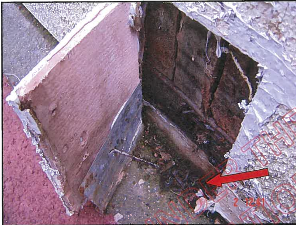
Close up of photograph 4c 104: note bottom plate is less than 50mm from surrounding ground level
