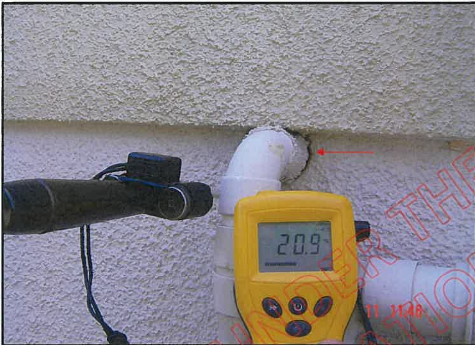
Probe reading at waste entry point; note waste penetration unsealed
