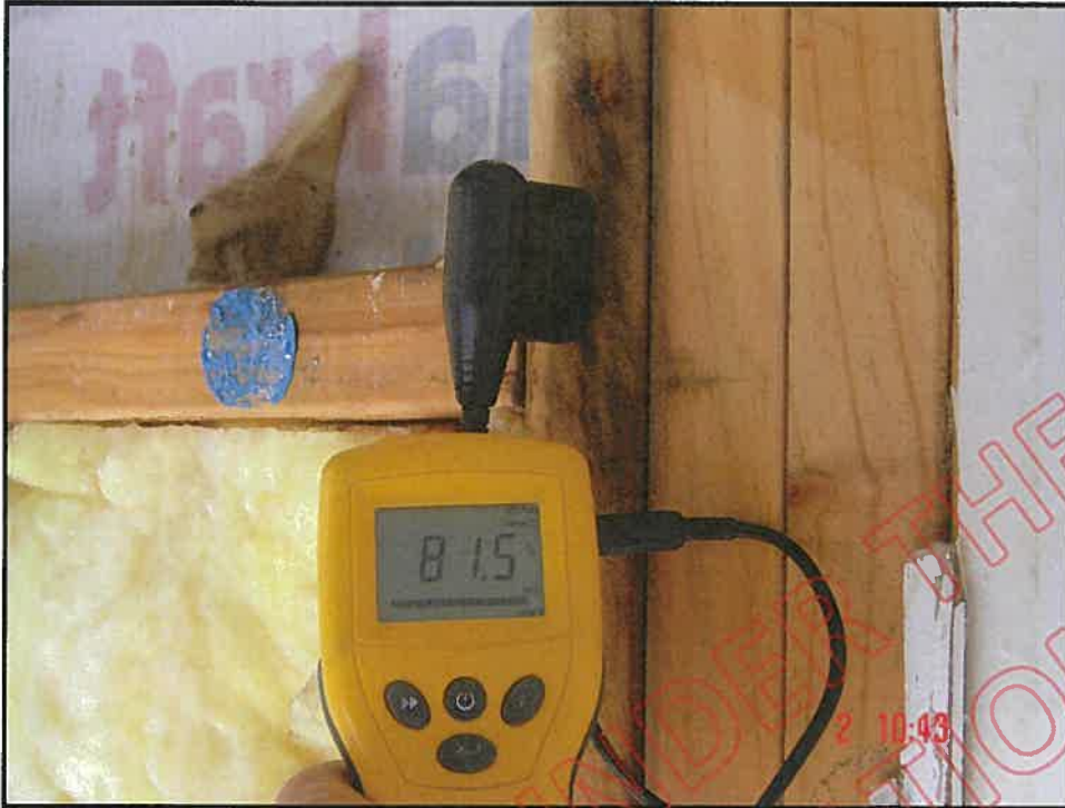
High moisture reading and decay in beam support framing
