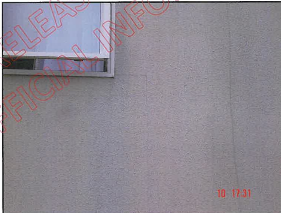
West wall showing incorrect sheet configuration and joint failure
