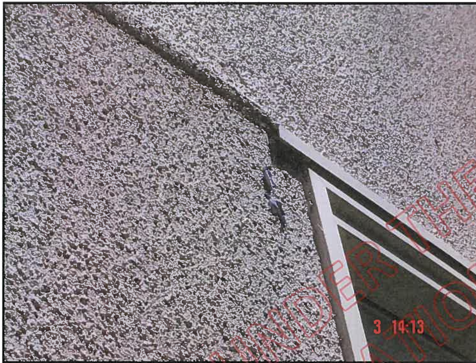
Photograph showing inter-storey H mould terminating at end of head flashing
