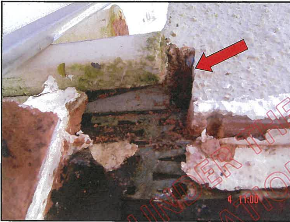
Close up of 5d 112 showing advanced decay and corrosion to nail plate; note no saddle flashing
