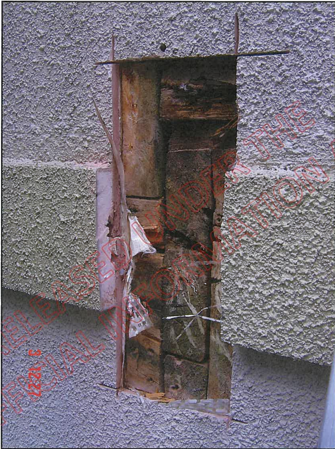
Cut out at north wall inter-storey below balcony wall junction: note advanced decay to studs, plate and end of 450x100mm support beam, note also the incorrect installation of the polystyrene reveal
