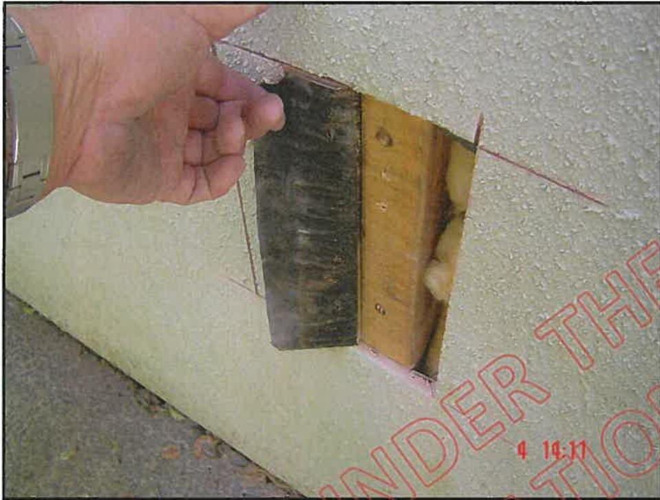
Cut out below garage window; south wall at base
