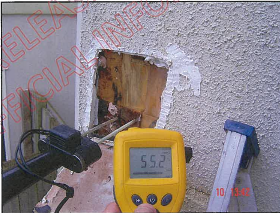
Cut out and high probe reading at northern corner of stair well
