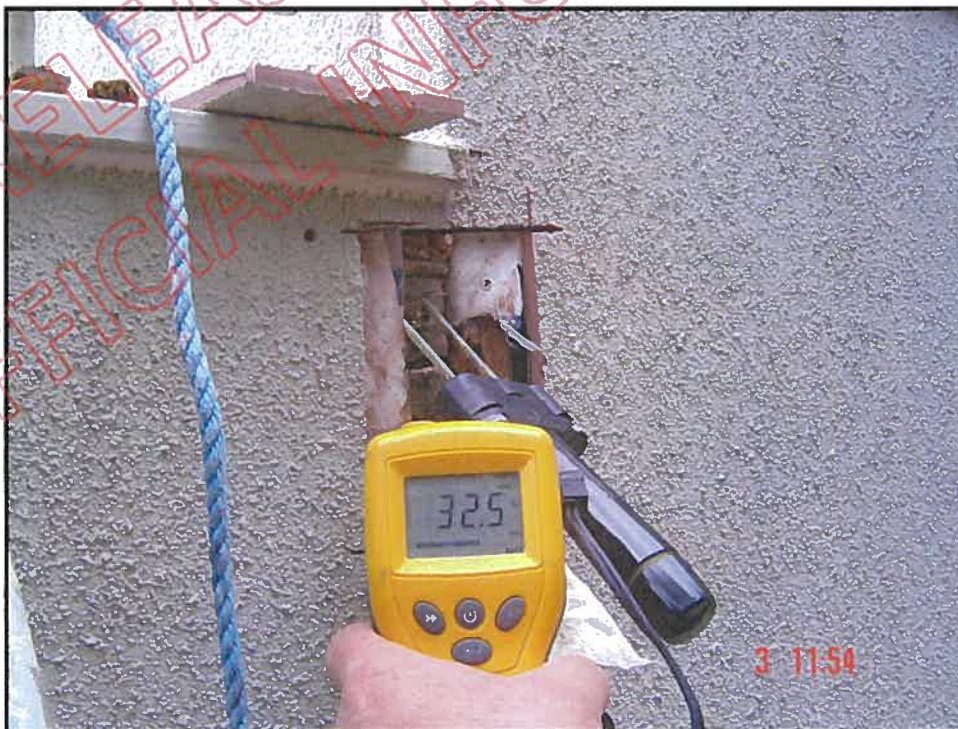
Cut out and high probe moisture reading at north wall / balcony wall junction; Laboratory sample 5.
