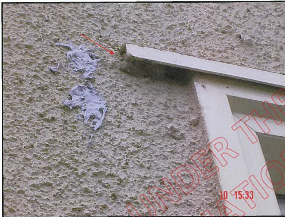
End of head flashing unsealed
