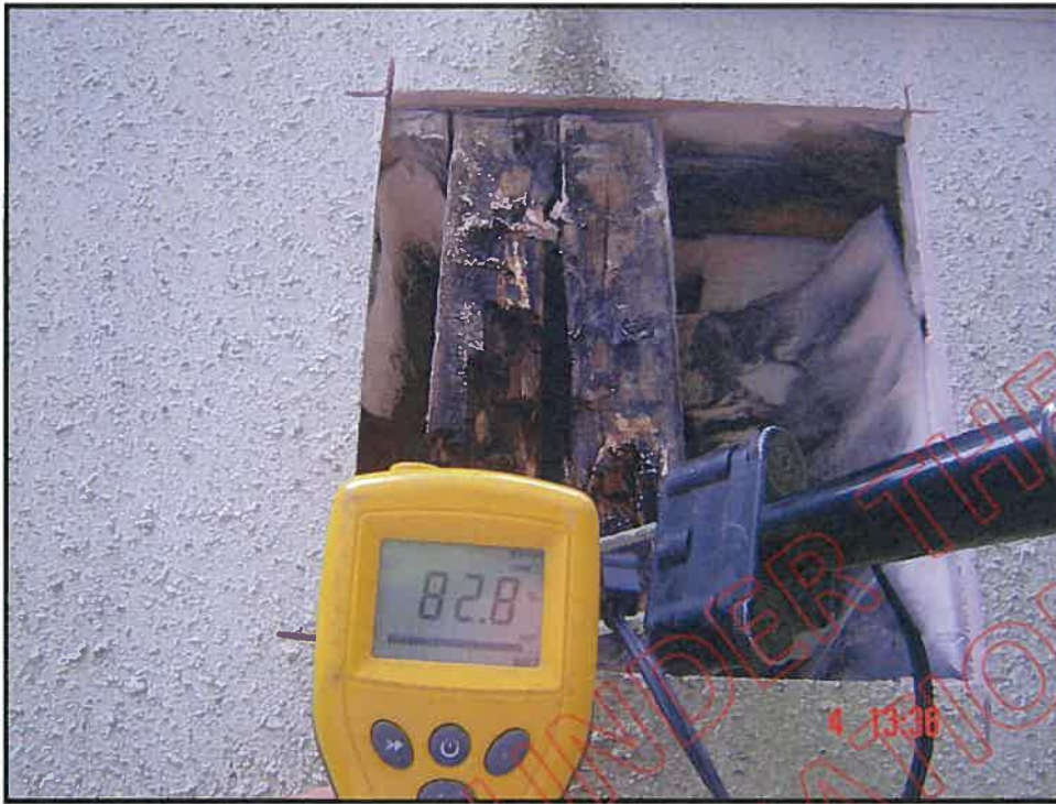
Cut out and high probe reading at south wall/balcony wall junction showing advanced fungal decay
