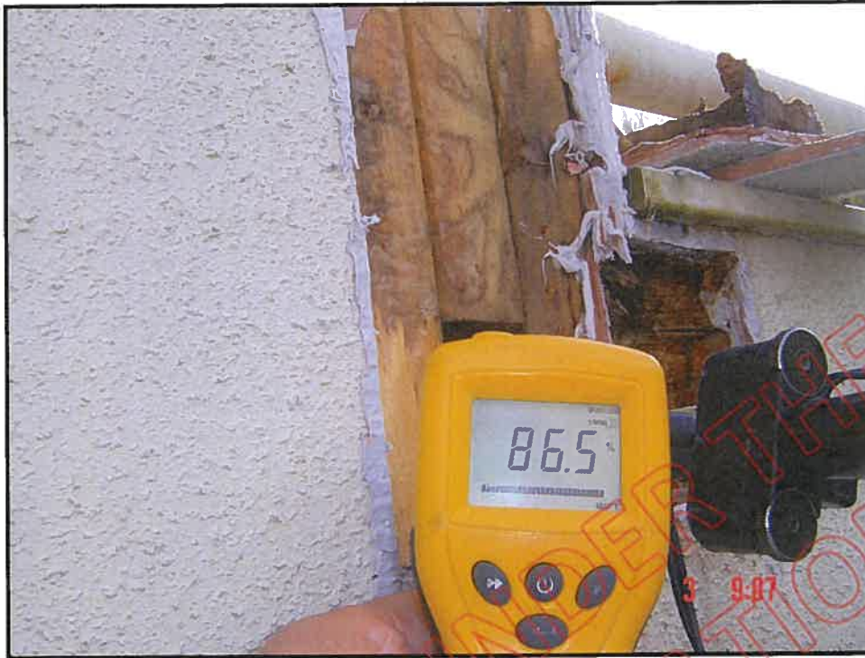
Cut out and high probe reading at south wall/balcony wall junction showing advanced fungal decay
