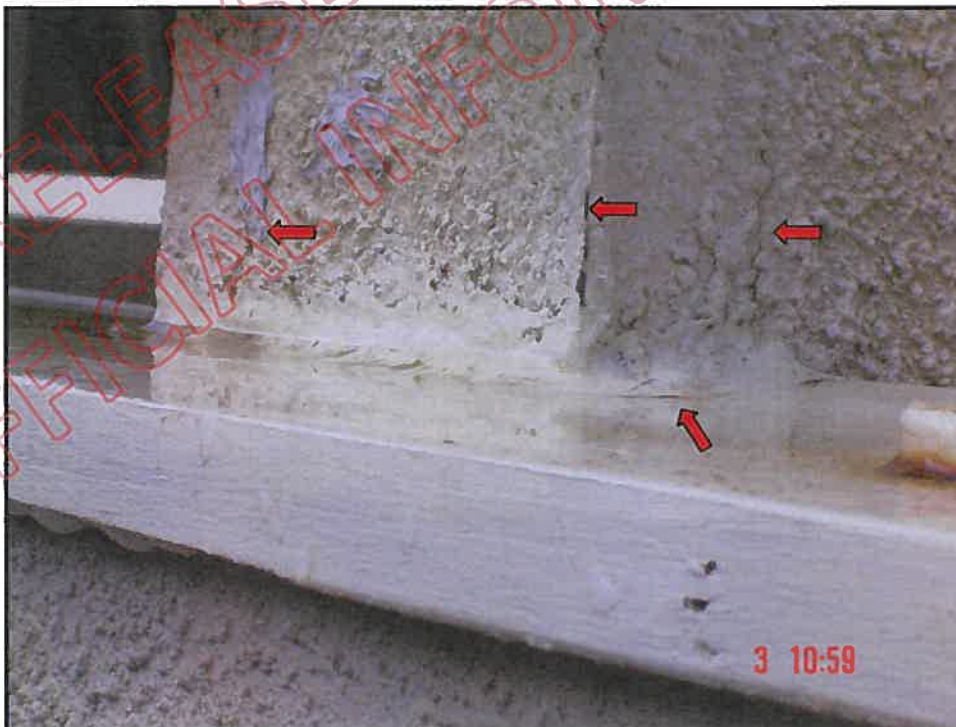
Balcony capping wing wall junction: note cracking at joins to wing wall cladding, no saddle flashing, exposed sealant failing. Point of entry for water ingress
