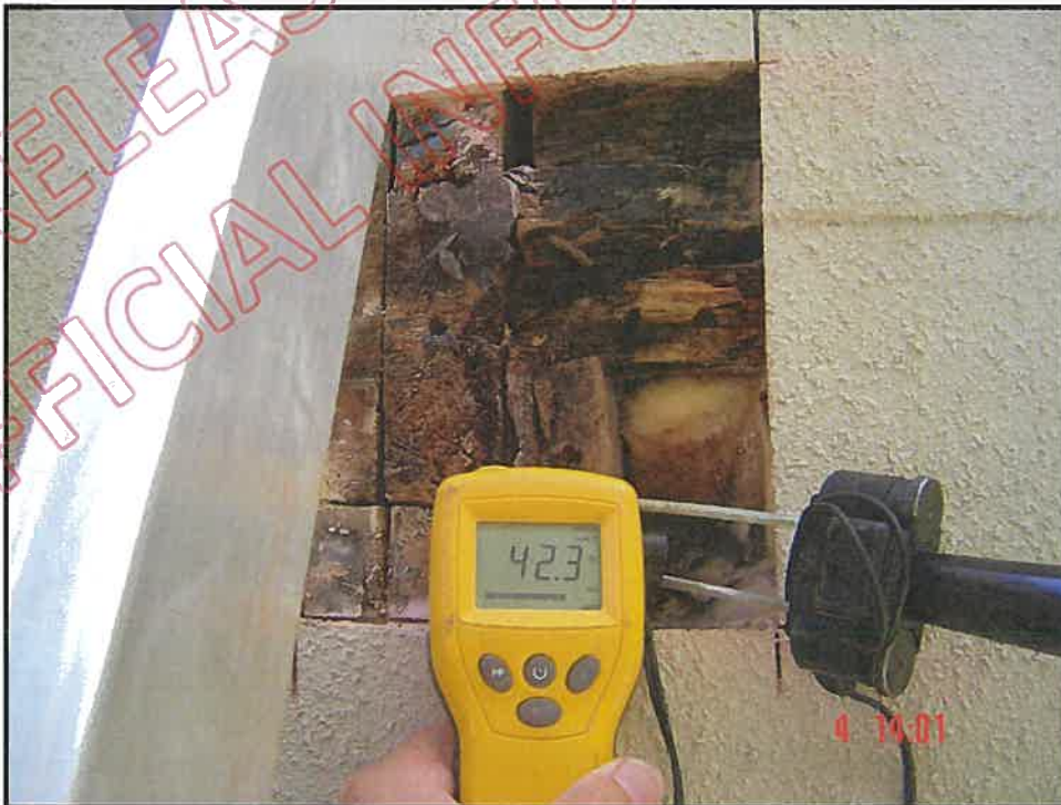
Cut out and high probe reading at south wall inter-storey below balcony junction, showing advanced fungal decay to frame garage beam and plates
