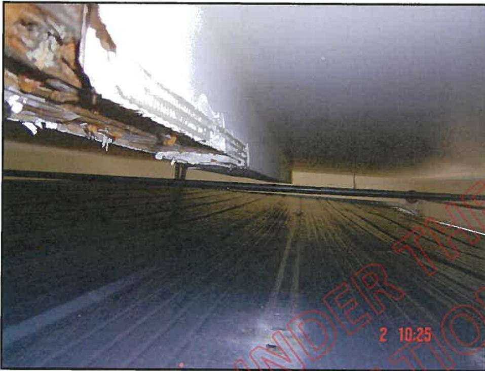
Photograph showing decay and slump in 450x100 garage beam
