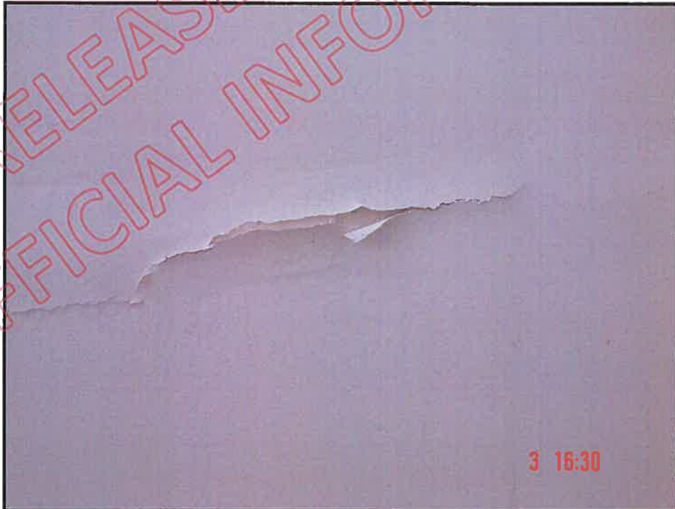
Damage to unit D lounge ceiling due to roof leak
