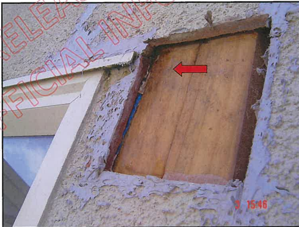
Cut out as above showing early fungal decay
