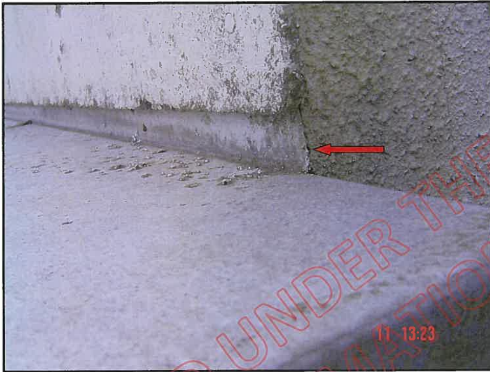
Poor detailing at end of apron flashing: point of entry
