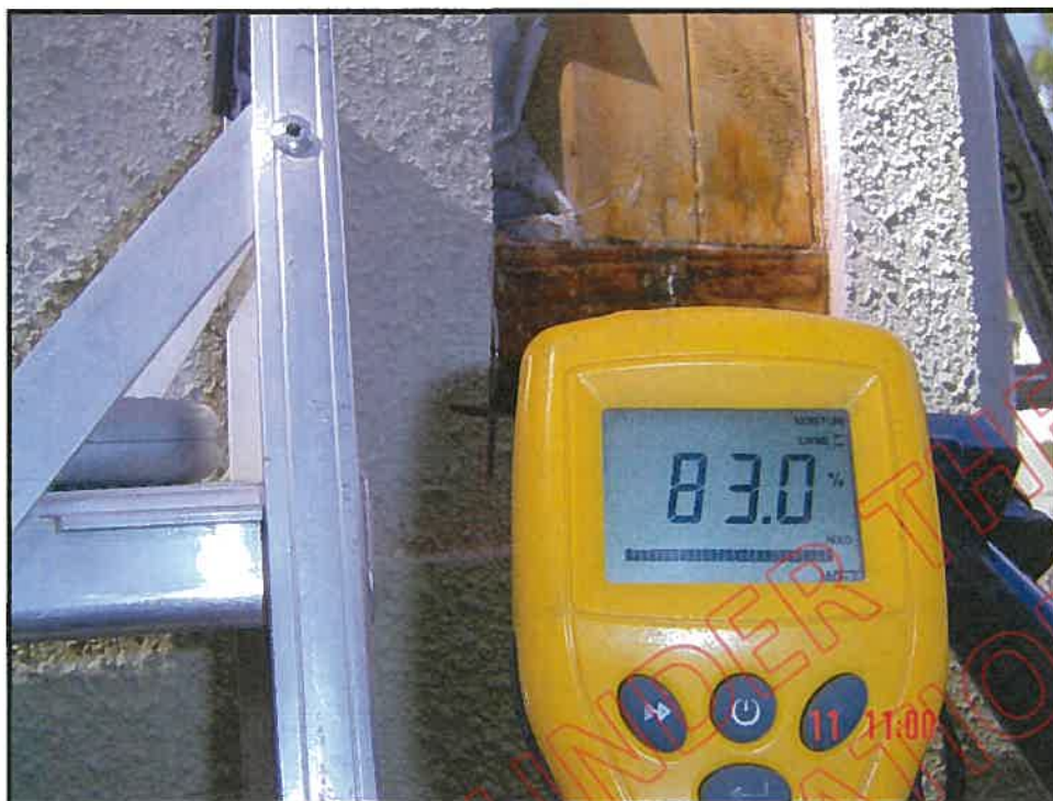
Very high probe moisture reading at cut out at North West corner in er-storey joint; (see cut out No. 12 elevation 2 north side)
