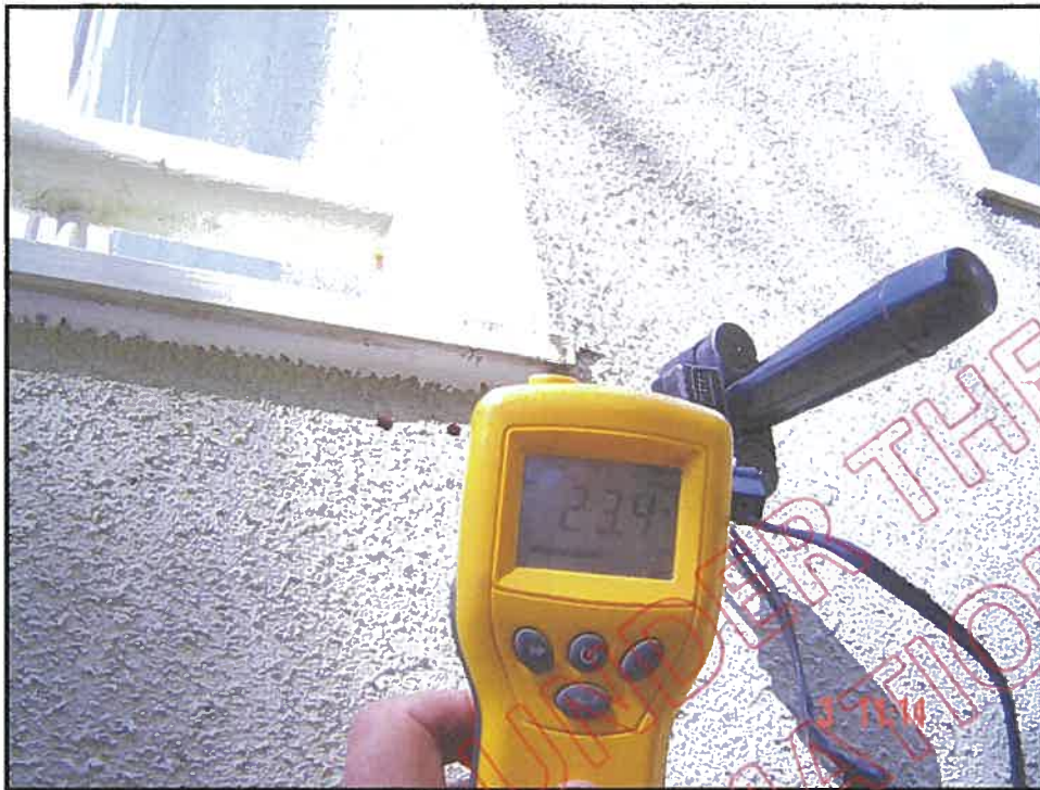
High probe moisture reading at north wall / balcony junction; note no saddle flashing, point of entry for water ingress
