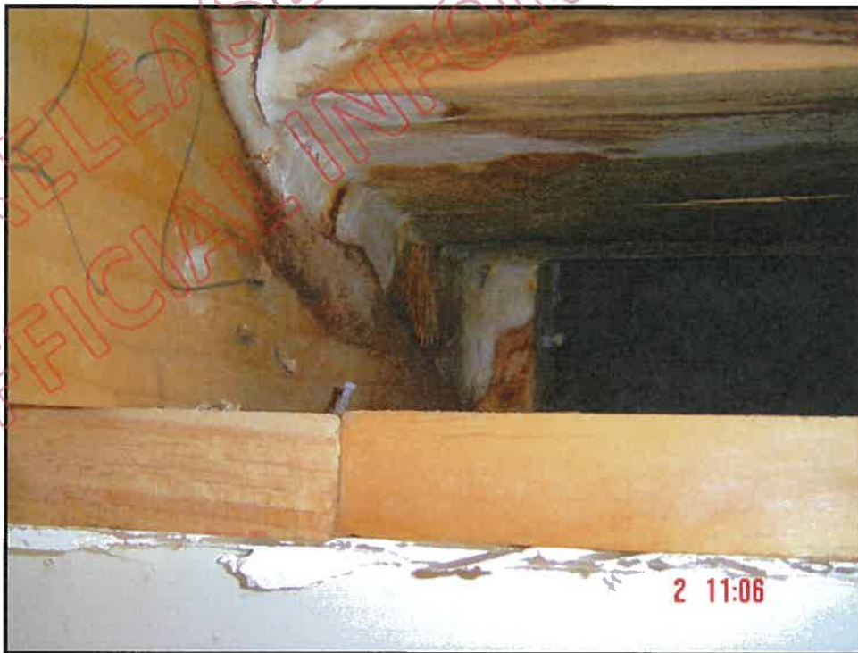
Heavy fungal decay in ceiling and floor joist supporting lounge floor and balcony
