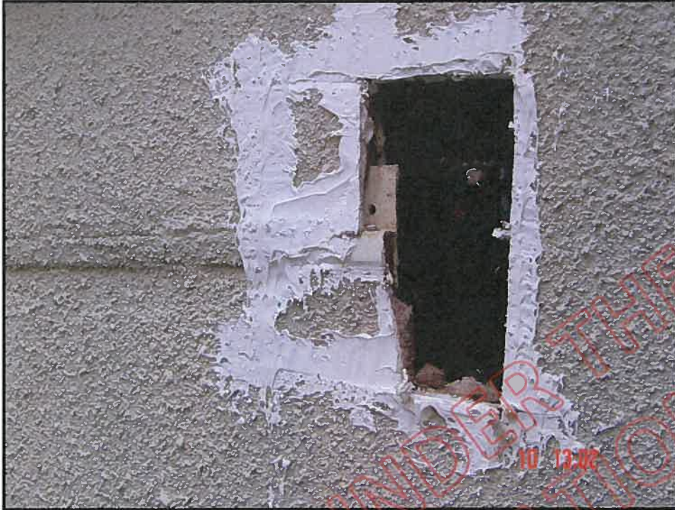
Cut out at first floor inter-storey below living room window showing advanced decay: note inter-storey H mould terminates at vertical-sheet join
