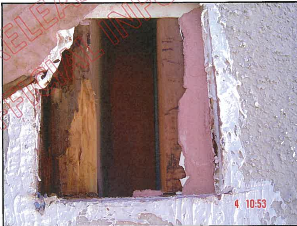
Cut out below inter-storey joint at north east corner
