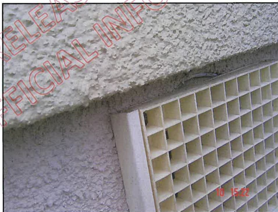
Unsealed extractor fan vent cover
