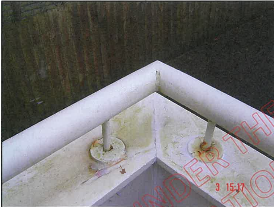
Open and unprotected timber capping mitre joint at north east corner; note also corroded and incorrect design and installation of hand rail stanchions
