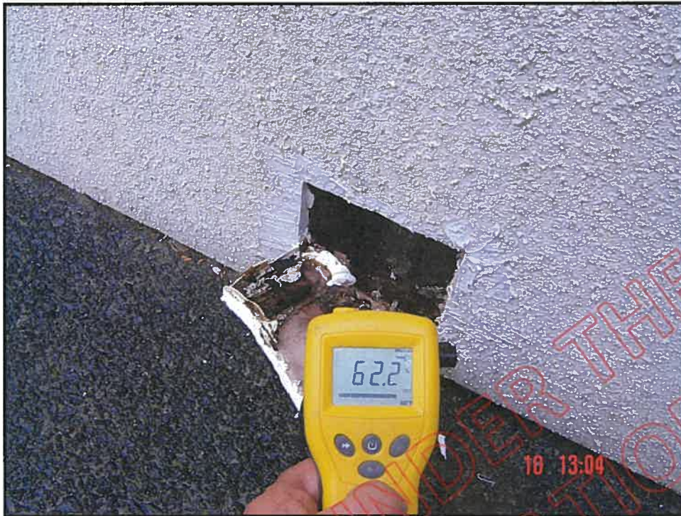
Cut out and very high probe reading at first floor at bottom plate below garage window: note cladding extends down to ground level
