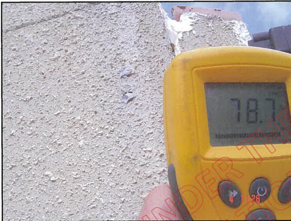
Cut out and very high probe reading adjacent to top left side of living room window, north east corner
