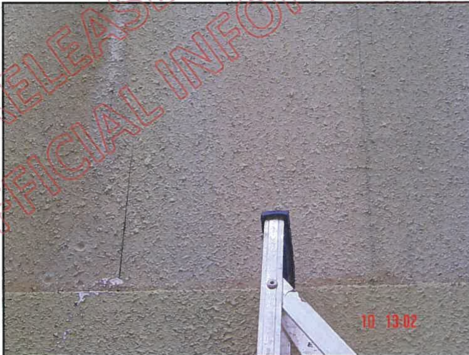
Photograph showing incorrect sheet configuration and joint failure above inter-storey
