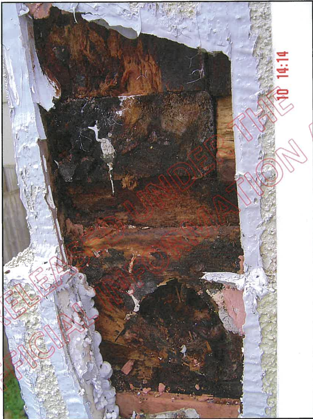
Cut out No. 10 as at photograph 3d 90 showing total decay of the framing, boundary joist, plates and flooring
