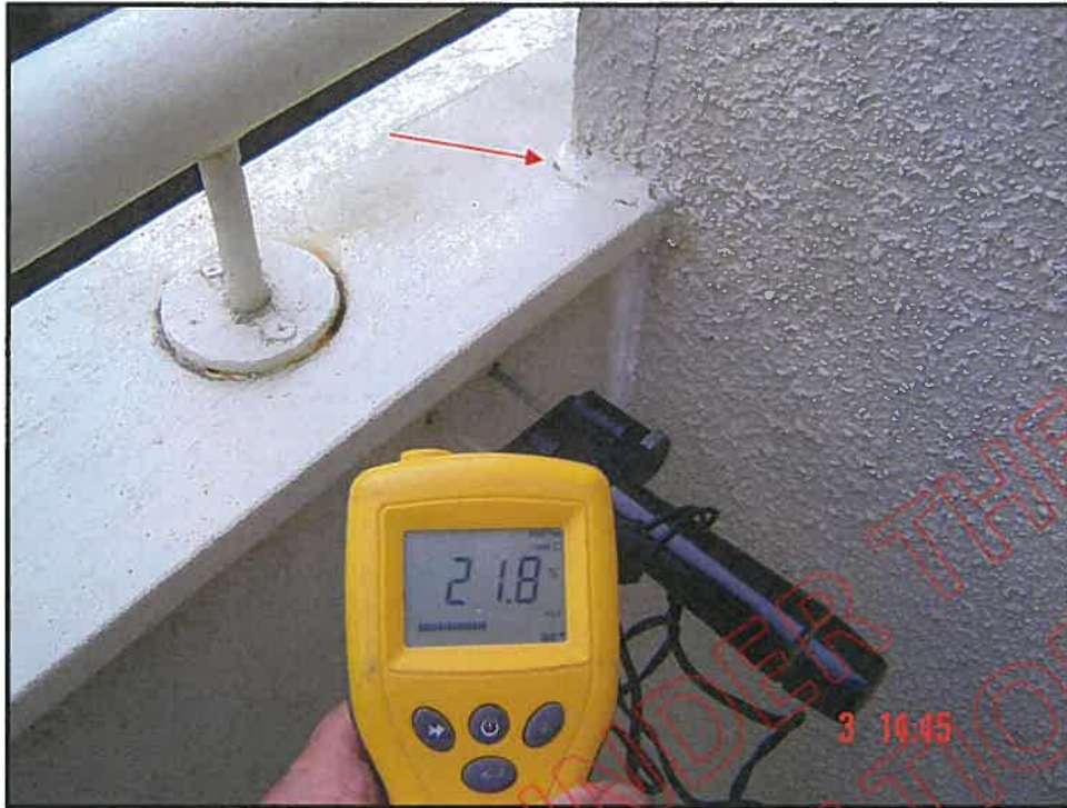
High probe moisture reading at top of balcony wall adjacent to the wing wall; note no saddle flashing at balcony / wing wall junction
