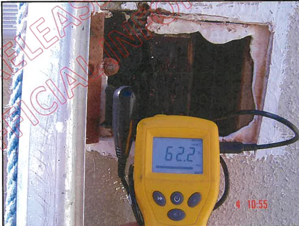
Cut out and very high probe reading below balcony wall and north wall junction
