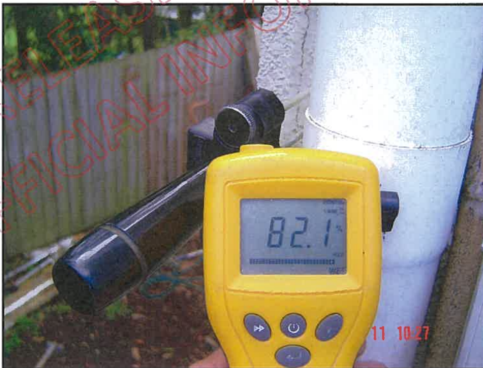
Very high probe reading at west wall below apron flashing junction
