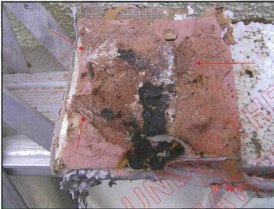
Back of Harditex™ showing decayed building paper and fungal hyphie infestation of the Harditex™
