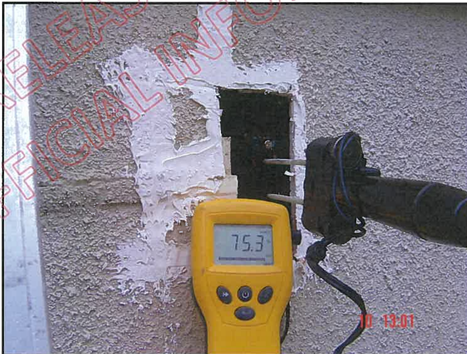
Cut out and very high probe reading at first floor inter-storey below living room window
