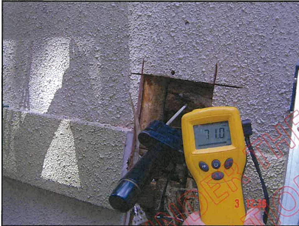
Cut out and high probe moisture reading at north wall inter-storey below balcony wall junction: note advanced decay to studs, plate and end of 450x100mm support beam, note also the incorrect installation of the polystyrene reveal
