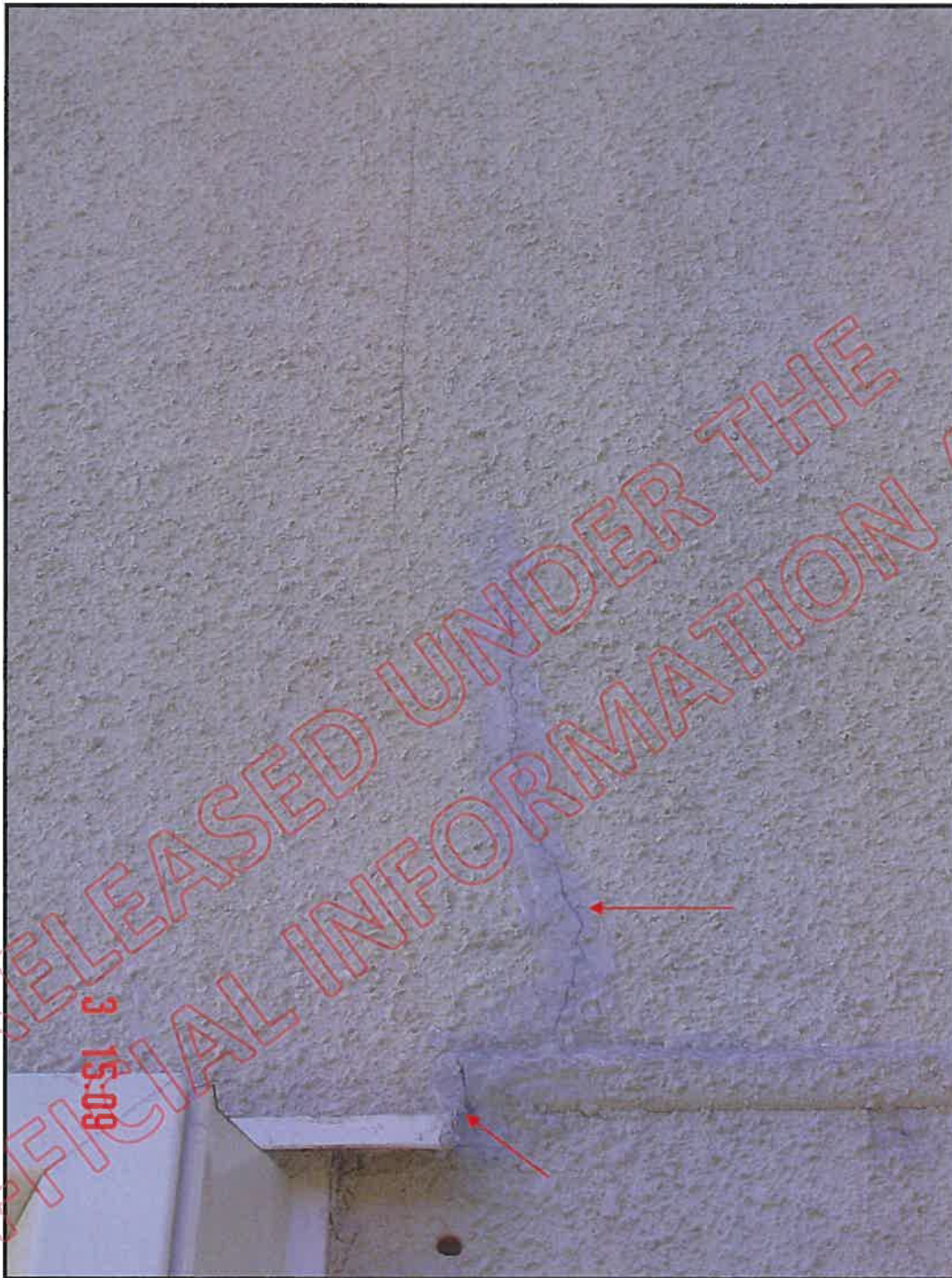
Inter-storey joint butts up to balcony door head flashing right hand side; Open joint is allowing moisture ingress: note cracking to cladding sheet above door head, recently sealed
