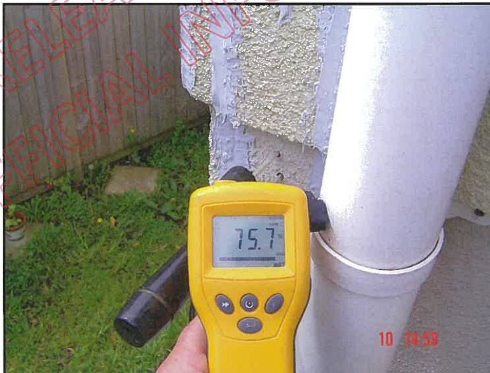
High probe reading below inter-storey junction
