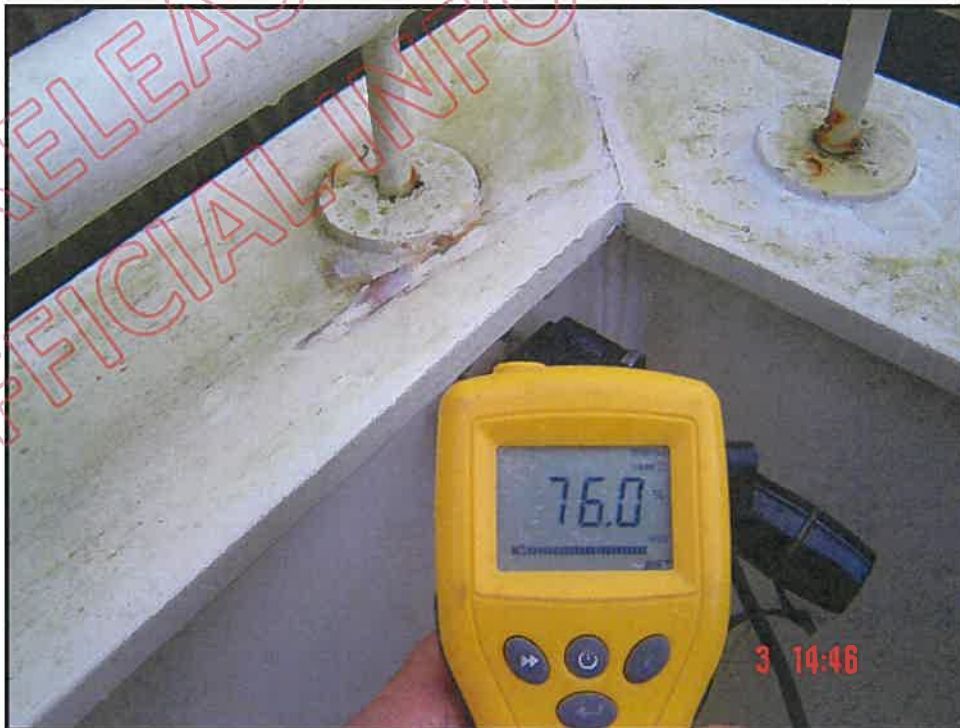
Very high probe moisture reading at top of north east corner of balcony wall
