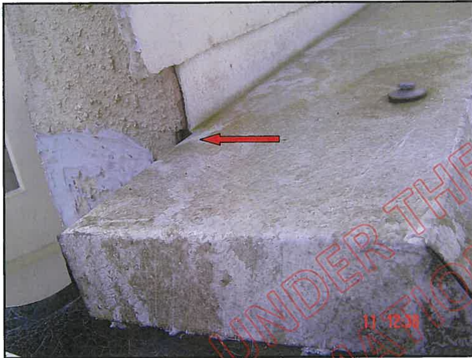
Poor detailing at end of apron flashing: point of water entry
