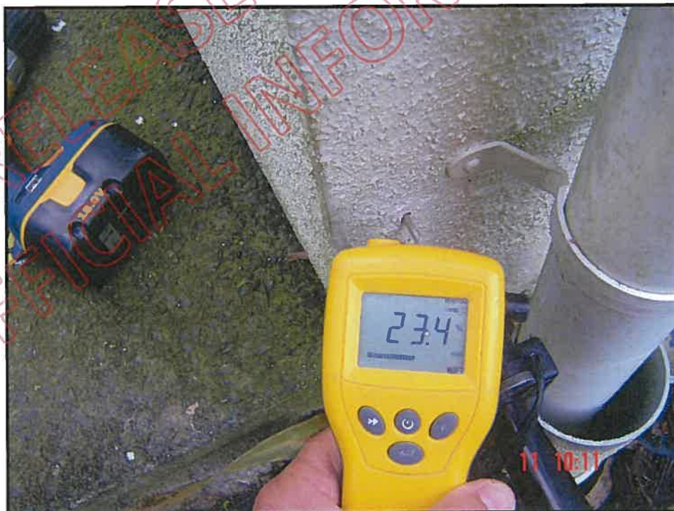
High probe reading at west wall 200mm above base
