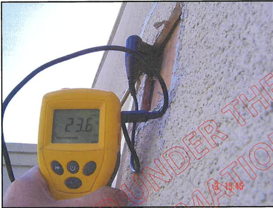
Cut out and high probe reading at head of living room window
