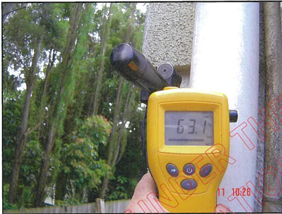
Very high probe reading at west wall below inter-storey
