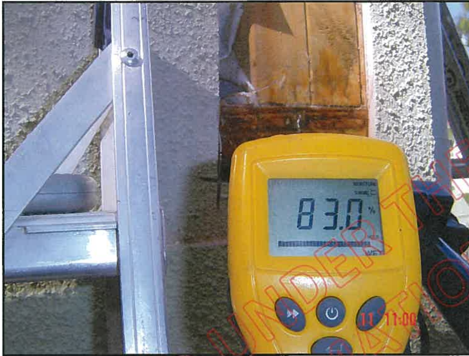
Cut out showing very high probe reading and decay at North West corner above inter-storey joint.
