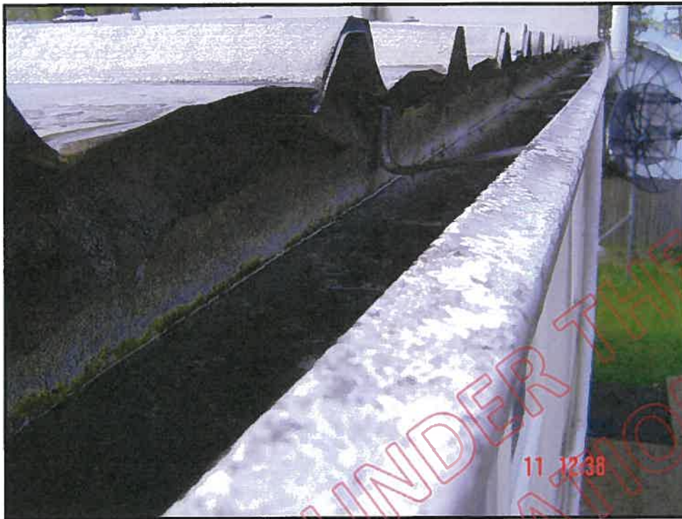
General view of spouting and roof end: note water ponding in spouting
