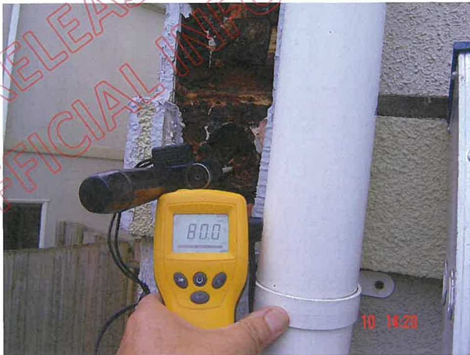
Cut out and high probe reading; northern corner at inter-storey junction
