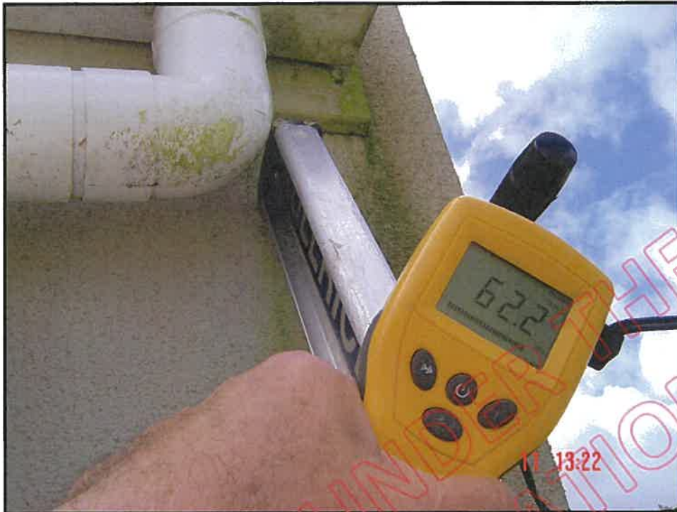
Very high probe moisture reading at south west corner below spouting
