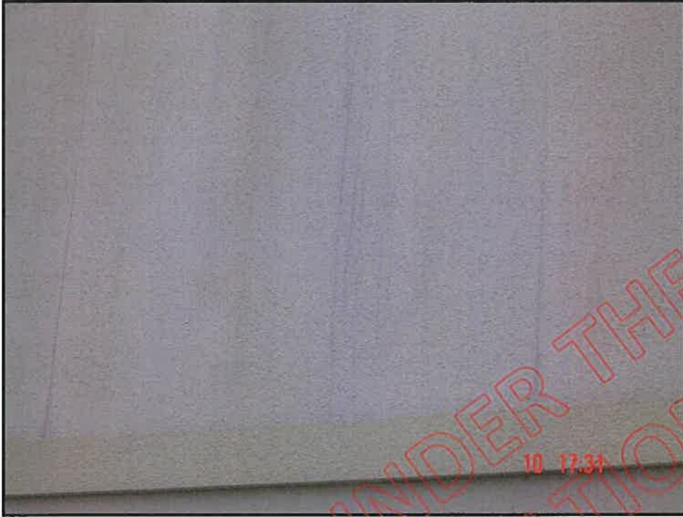
West wall showing joint failure
