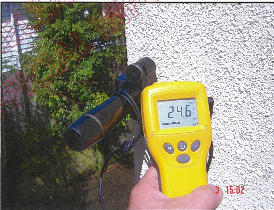
High probe moisture reading near top of wing wall at front
