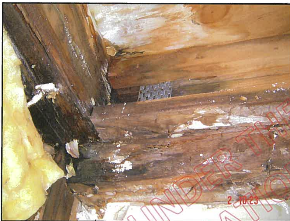
Photograph showing totally decayed 450x100mm beam
