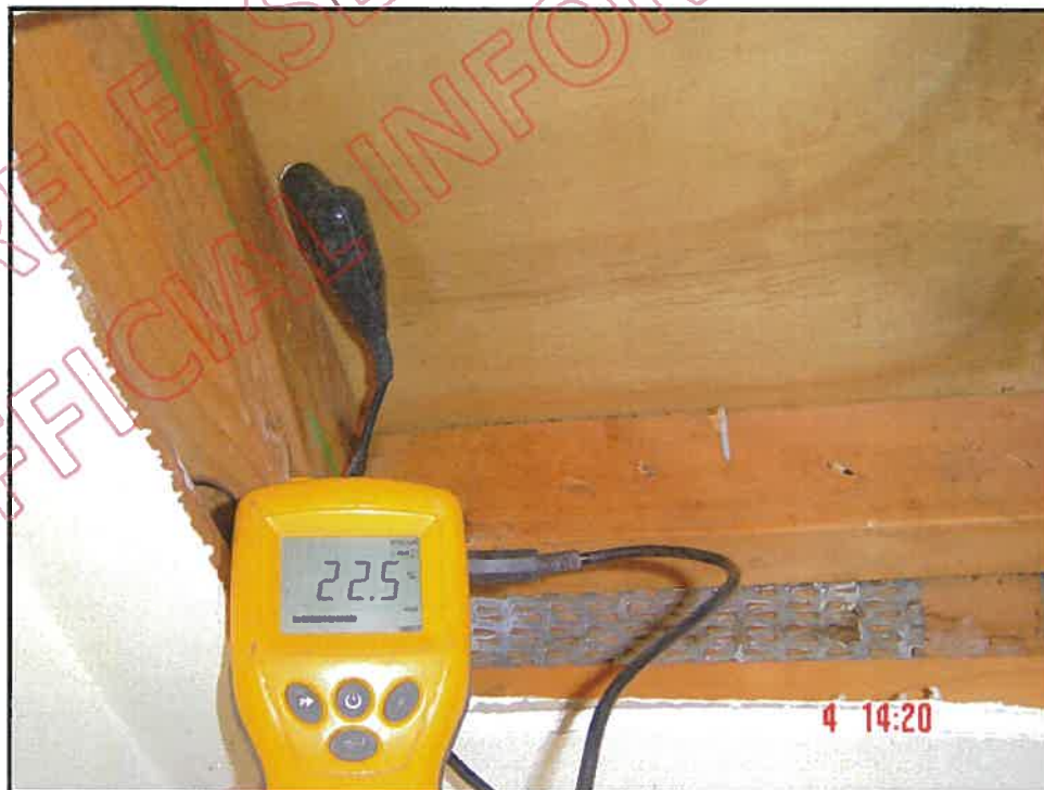
Elevated moisture reading in Unit E garage ceiling
