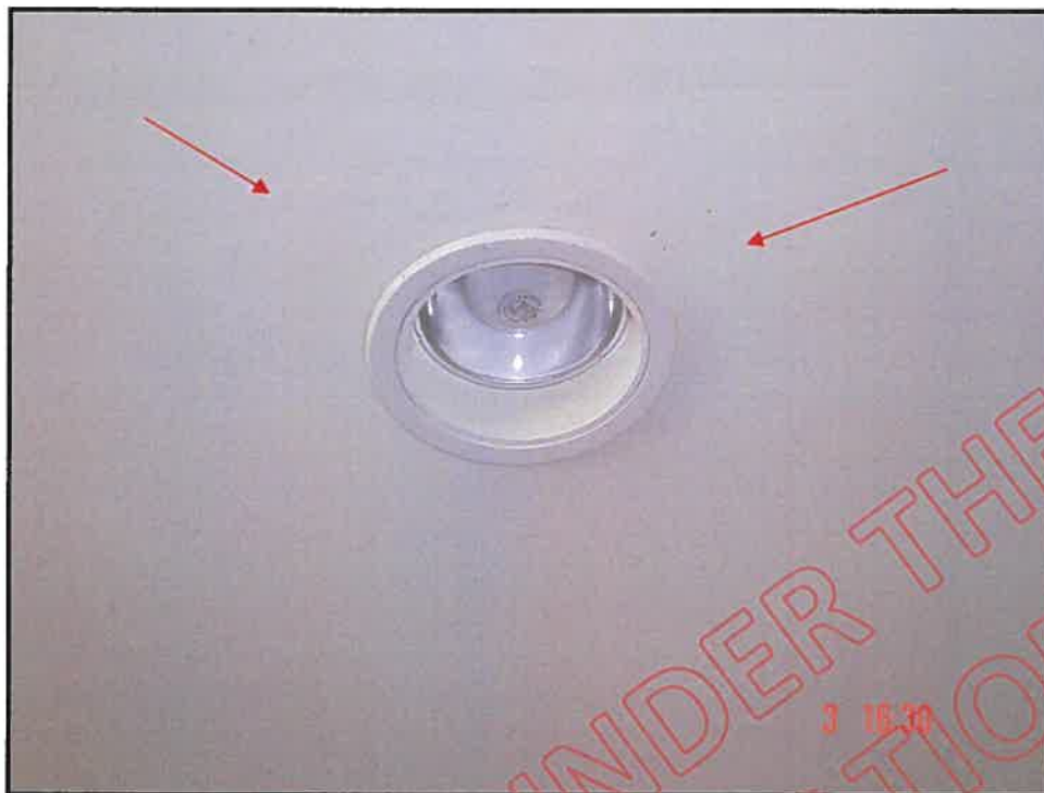
Damage to unit D lounge ceiling due to roof leak
