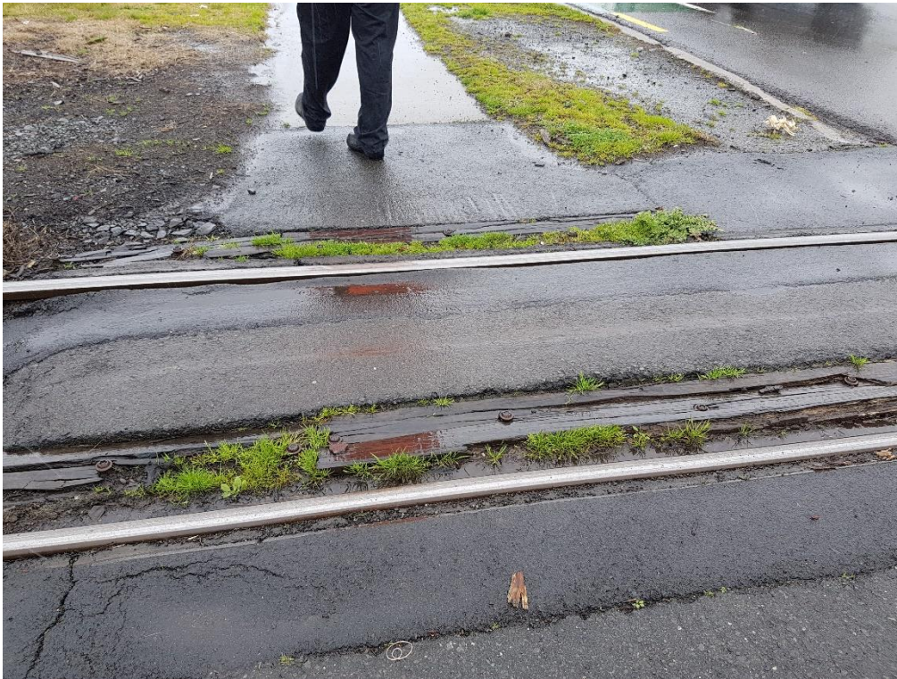
Typical Flange Gaps
