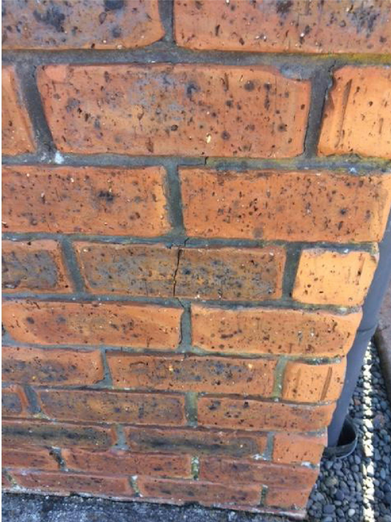
Figure 5 : South west Garage corner, step cracking and a broken brick
