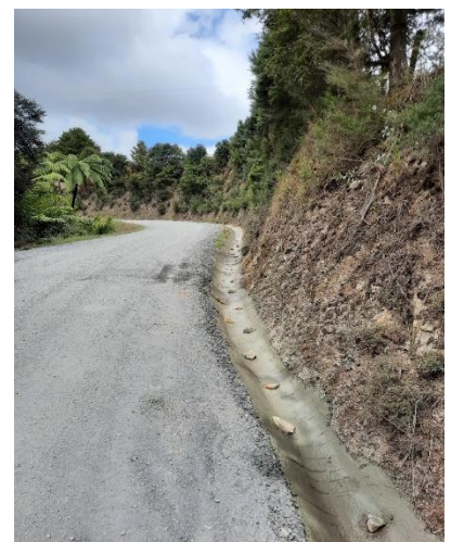
Dish channel – Waipu Caves Rd
