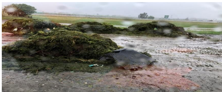
Figure 79: Debris removed from the inlet grates at the Purimu pump station, 9th November 2020
