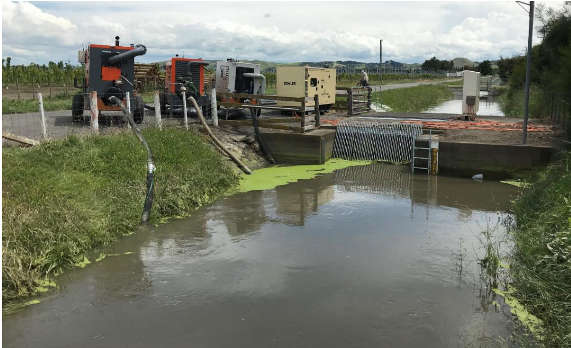
Figure 37 Mobile pumps and generator at Waverely pump station
