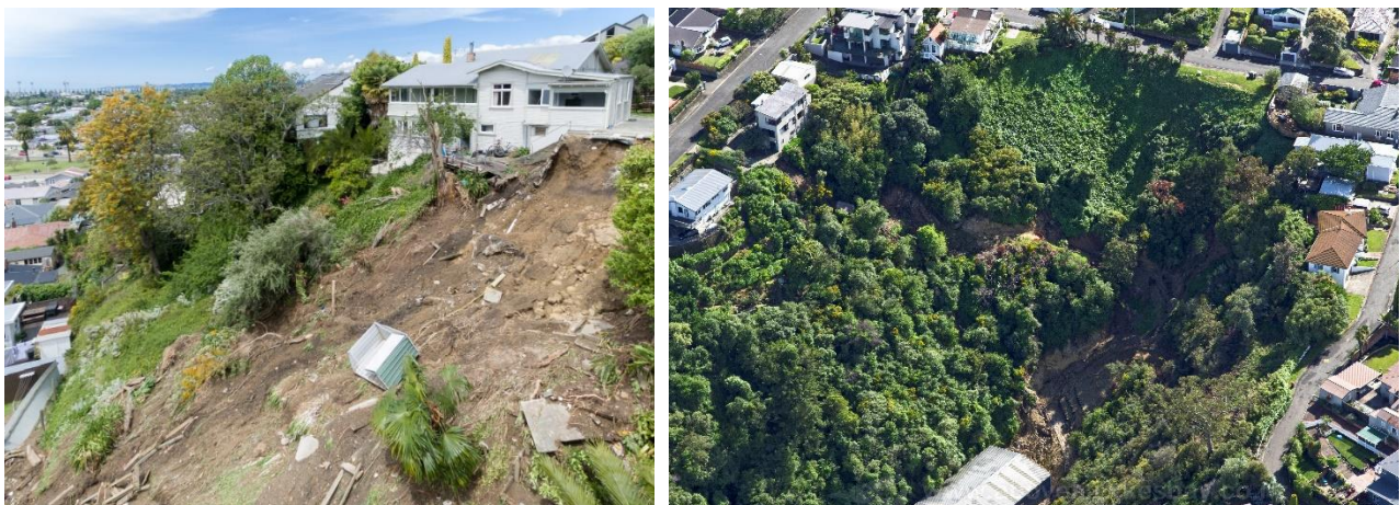
Figure 81: Damage to a property on Napier Hill from landslide, Tuesday 10th November 2020
