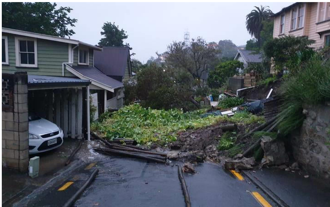
A large slip has affected houses on Brewster Street, Napier. Photo / RNZ
