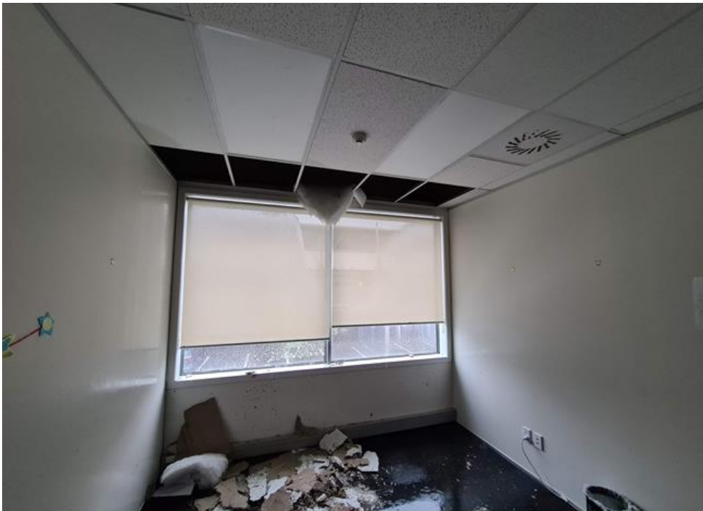
Figure 85: Damage to a commercial building on Vautier Street as a result of heavy rainfall, 9th November 2020
