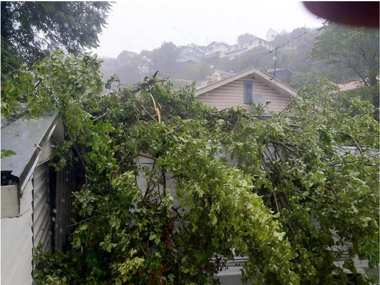
A tree had fallen onto a caravan on Shakespeare Rd in Bluff Hill, Napier, on Monday. Photo / Daniel Bryant
