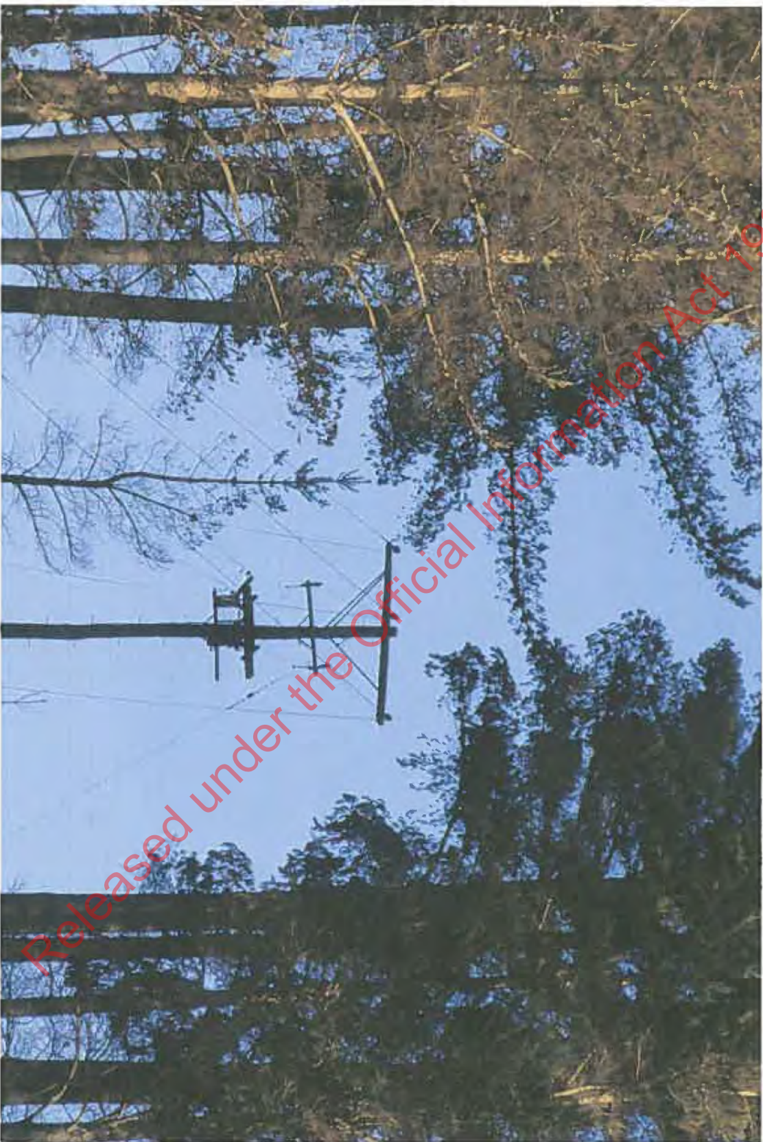
Photos 945 – Further non maintained trim zones on ET2 above 205 Morris Rd.
