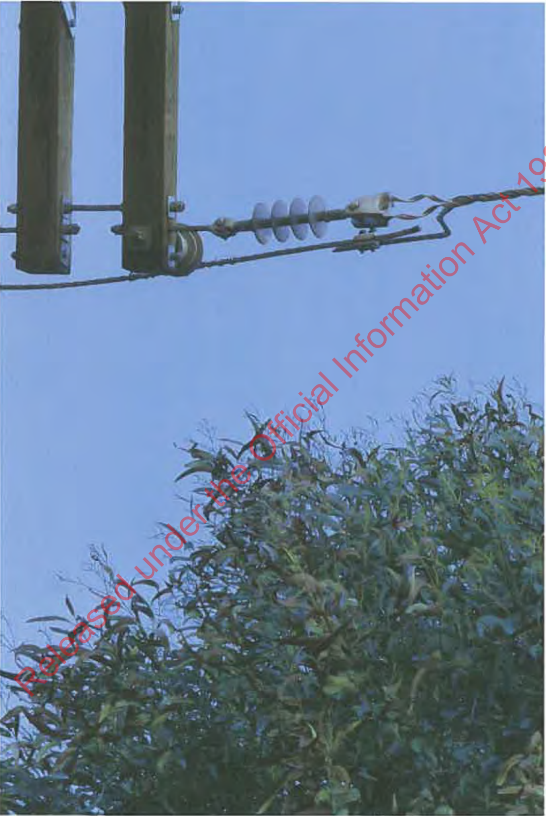
Photos 976 – Looking up the Recloser (A00) pole showing vegetation within 500mm of line.
