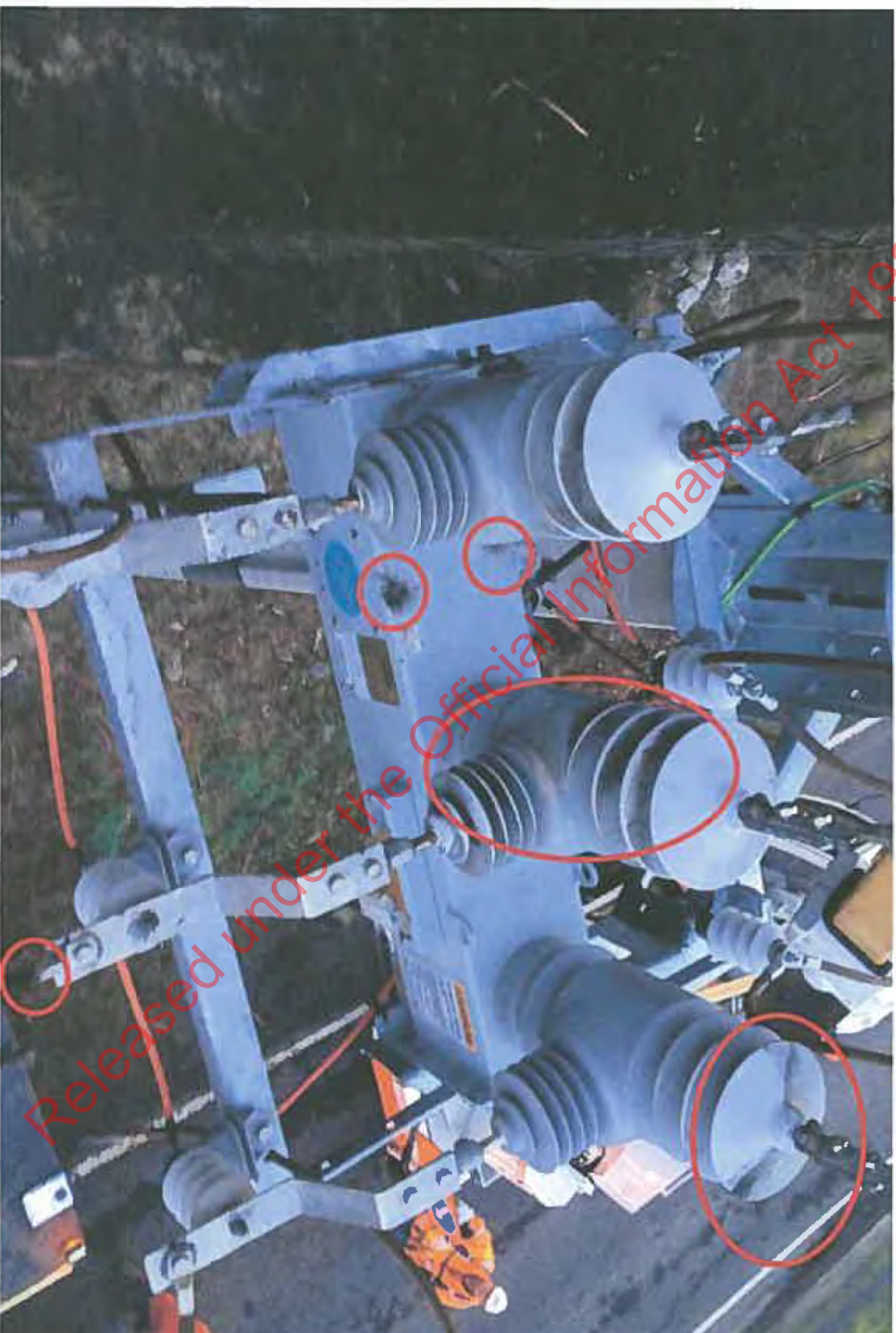
Photos 3 (4) Delta – Recloser unit on AOO pole 821286. Shows damage, carboning and charring to Recloser.
