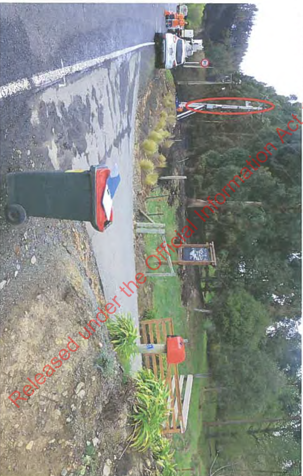
Photos 919 – Approaching the scene to the NW of the entrance to 231 Morris Road. AOO pole visible with Delta staff downloading trip data from the Recloser unit.
