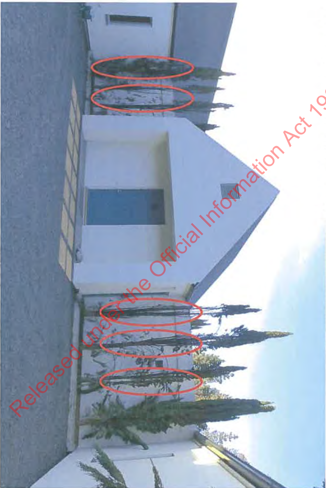
Photos 003 – Fire damaged trees either side of the front door on 47 Coalstage road. Evidence of significant ember attack.
