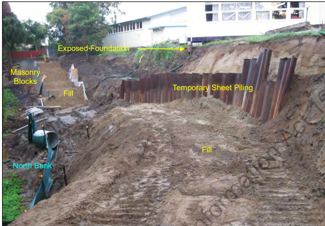
Figure 7: General view of segmental retaining wall during construction c 2009 – photograph supplied to LDE Ltd.
