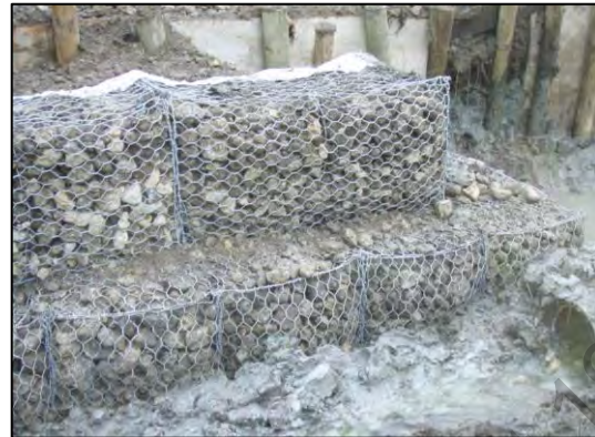
Figure 5e: 22/05/2012 – completed segment of gabions. Note old wooden piles and concrete behind gabion.
