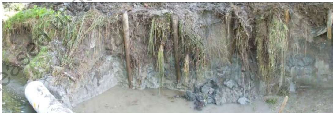
Figure 5c: 16/05/2012: General view of excavation with possible timber pole driven piles exposed in excavation wall.
