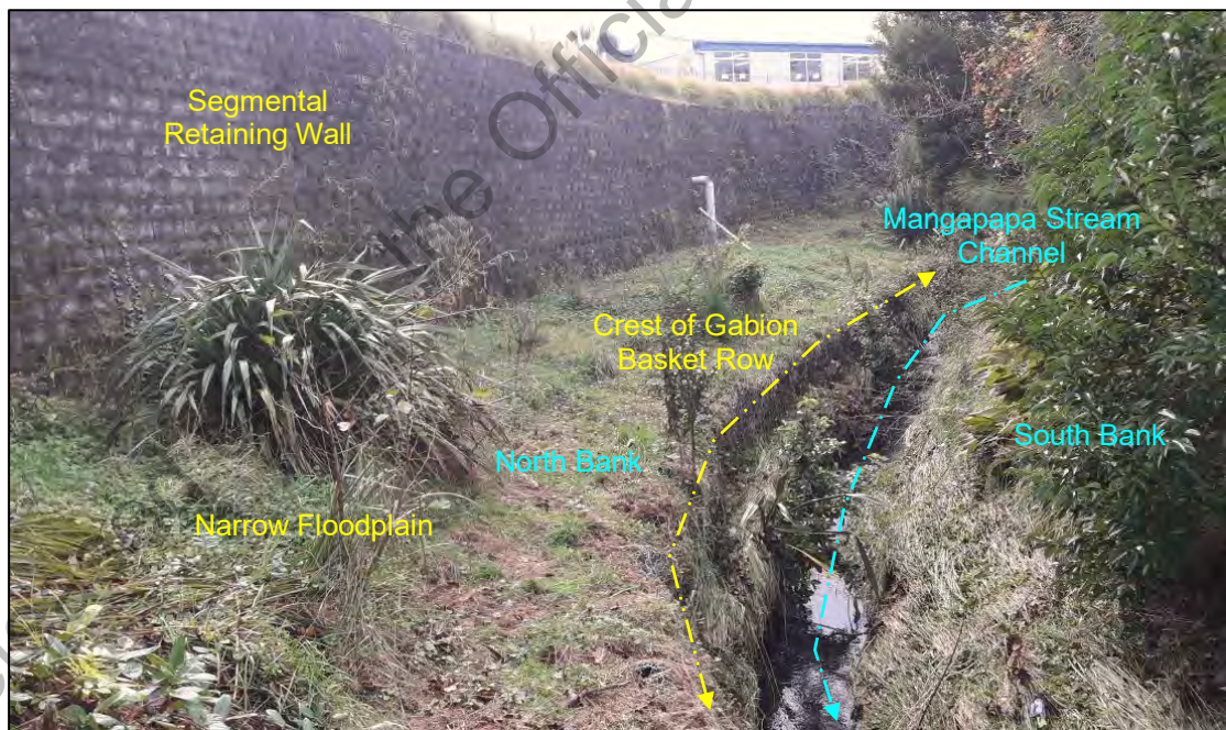
Figure 8: General view of the current Mangapapa Stream condition facing north. Note position of gabion baskets and 4.8m high segmental retaining wall.
