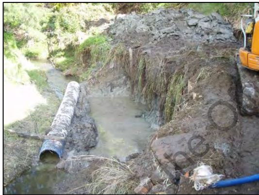
Figure 5a: 16/05/2012 – initial undercut.
