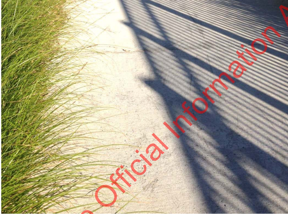
Figure 1: Grass encroaching over the cycleway path
