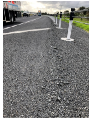
Figure 8: View looking north along the southbound lane, north of Armitage Road on-ramp.
