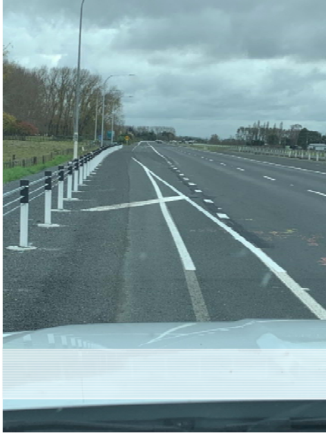
Figure 9: Note pavement marking deficiencies
