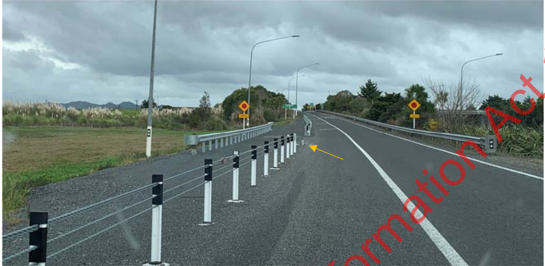
Figure 6: Maintenance bay gap in barrier
