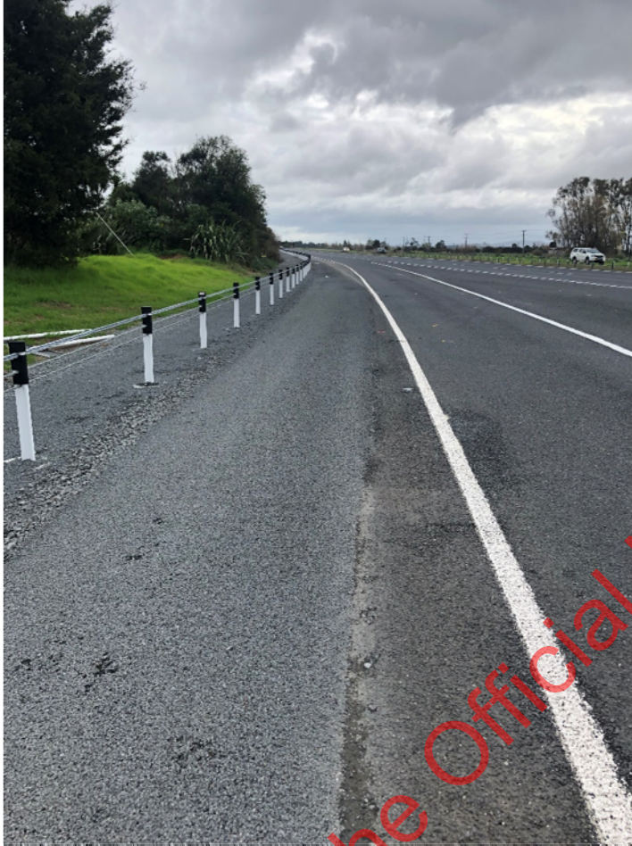
Figure 10: “Expressway” sign lying on the roadside berm
