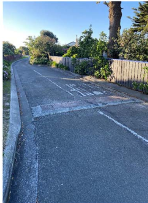
Road markings fading, maintenance required
