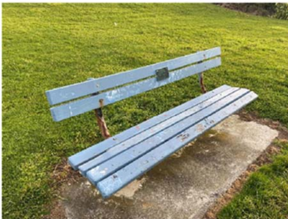
Bench needing removal and a potential new picnic area planned
