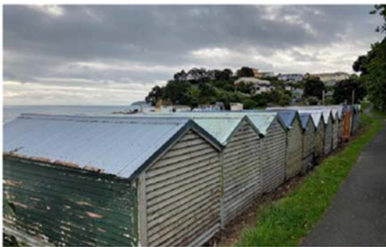
Paint peeling on boatsheds, picture taken from pathway leading to Vella Street
