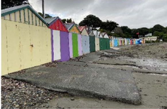
Broken concrete in front of boatsheds, looking South
