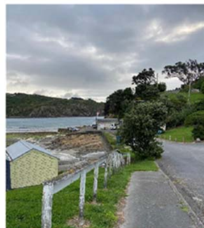
Handrail and footpath needing maintenance, taken from Vella Street looking towards the toilets
