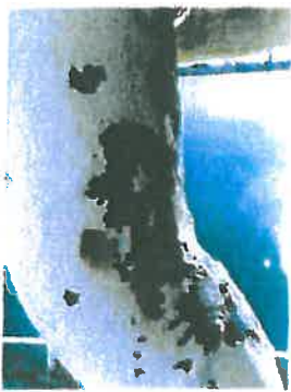
Corrosion on vent pipe
