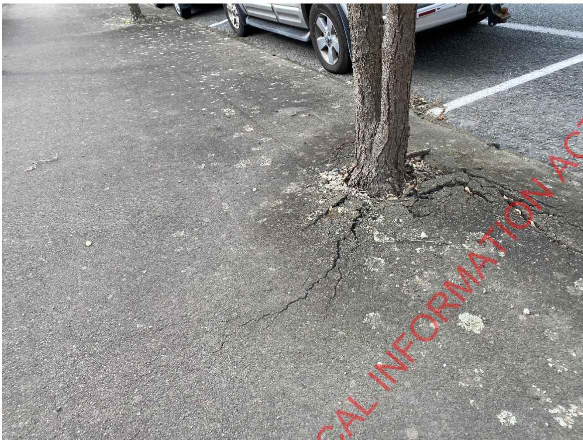
Figure 22: Existing uneven path adjacent to Hutt Road.
