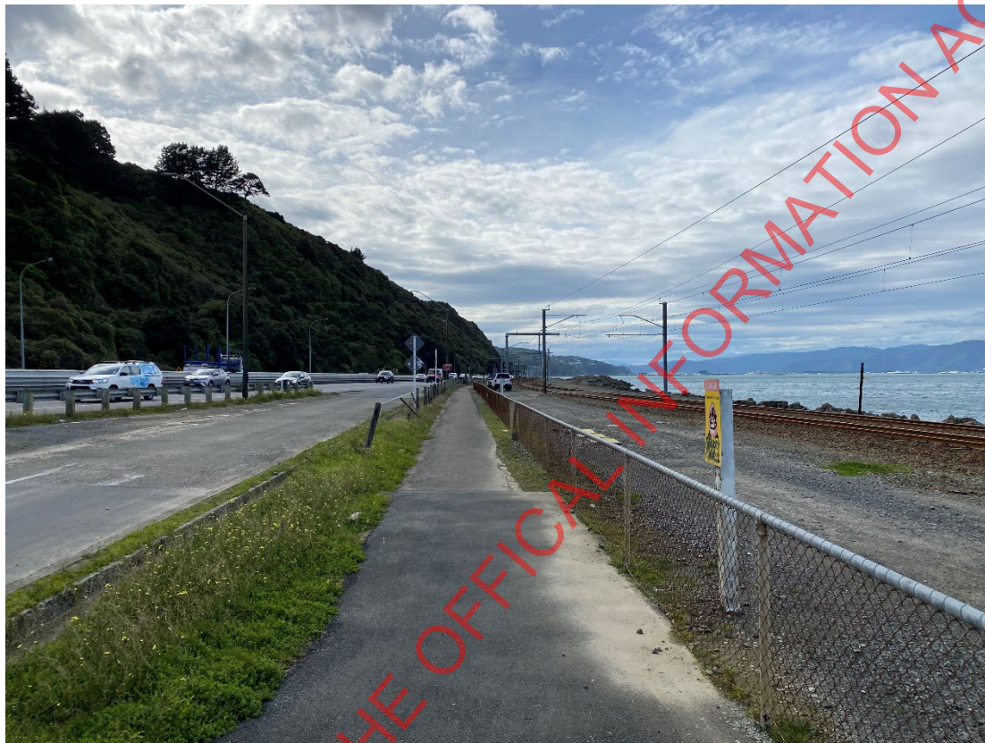
Figure 8: Gravel and debris creeps on existing path near Kiwirail access track
