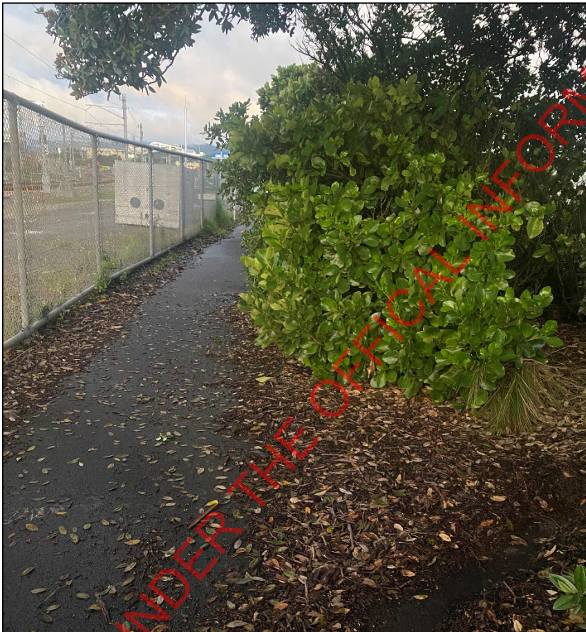
Figure 16: Poor vegetation clearance along the existing path to the north of the interchange
