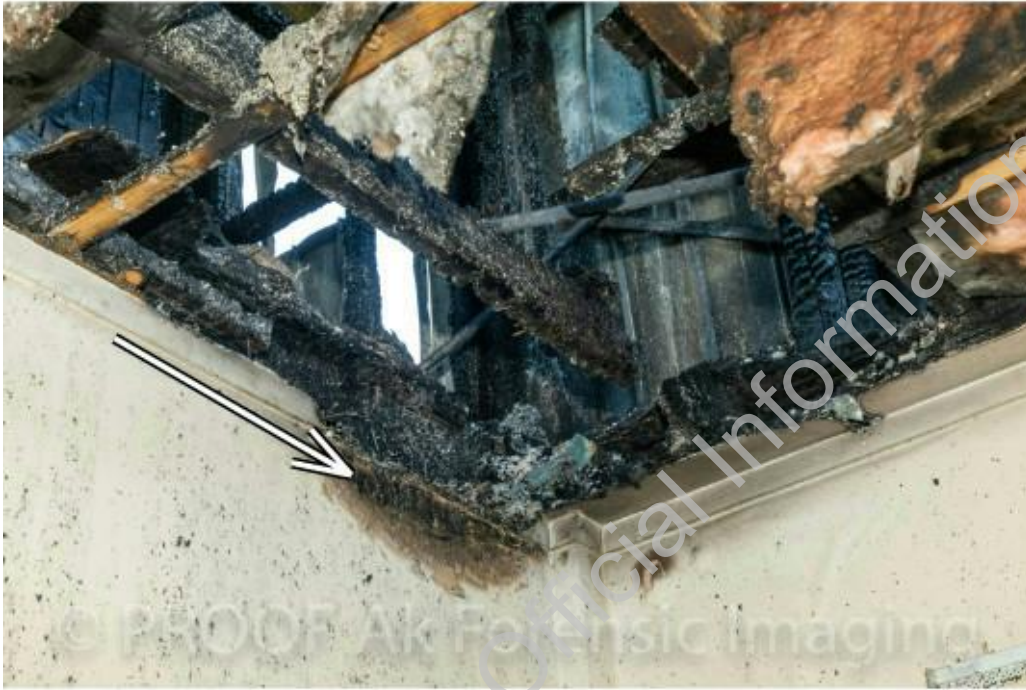
Photograph 25: Arrow indicating irregular burn patterns in bedroom 2. (Courtesy of Police)
