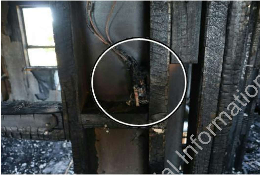
Photograph 31: Bedroom light switch in area of origin. Examined no signs of failure.
