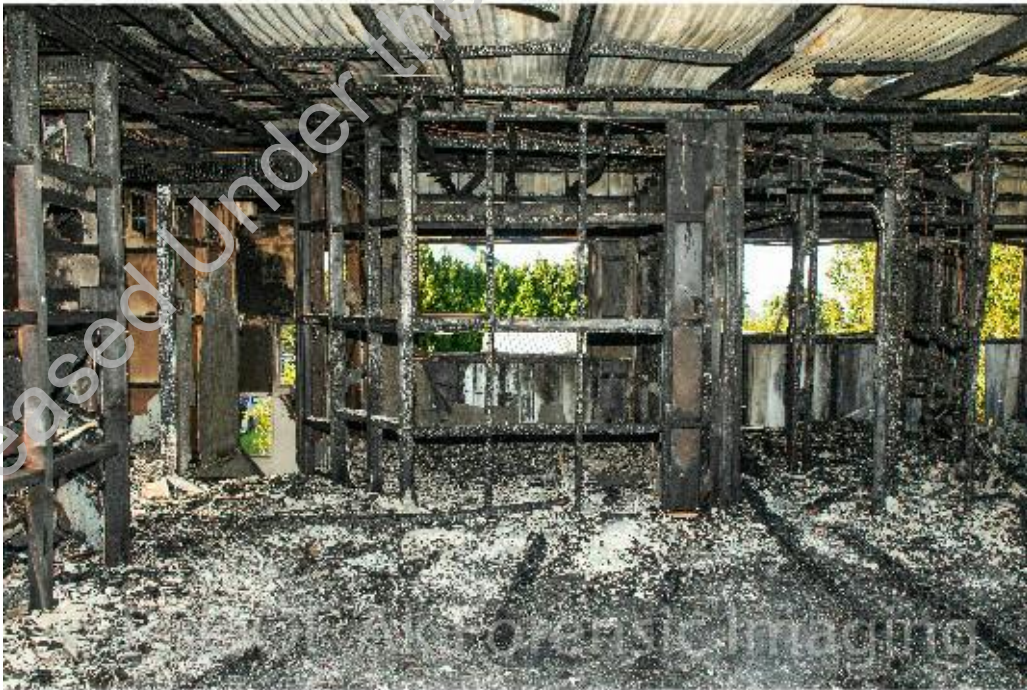
Photograph 32: Lounge room area looking towards front of the dwelling. (Courtesy of Police)
