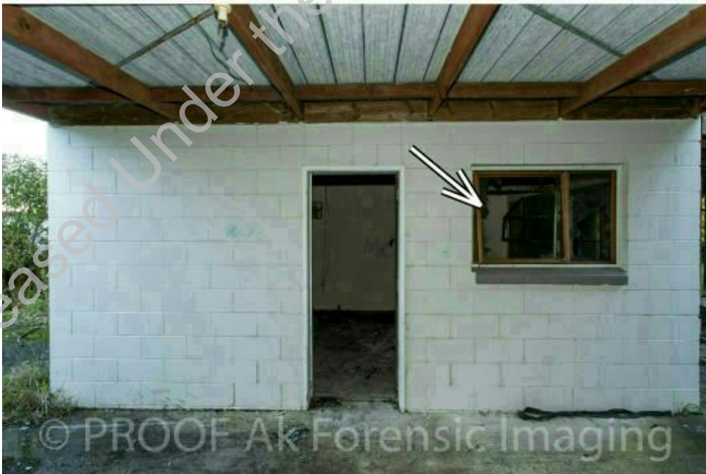
Photograph 9: Mechanically windows broken on the lower levels. (Courtesy of Police)
