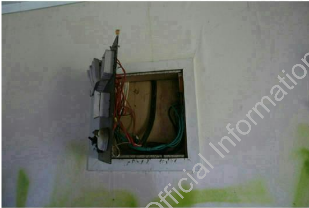
Photograph 21: Cables at the rear of the fuse board.
