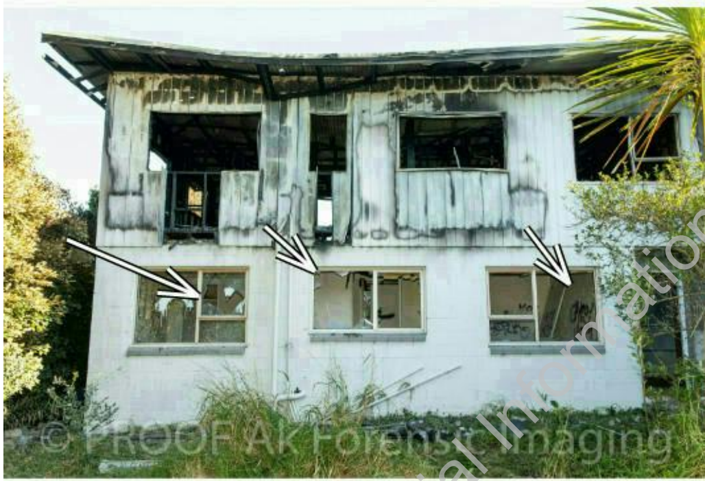
Photograph 7: Arrows indicating mechanically windows broken on the lower levels. (Courtesy of Police)
