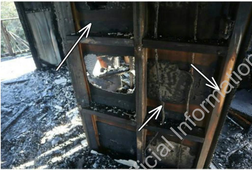
Photograph 30: Unburnt timber wall framing in the kitchen and electrical cables that still have insulation present.
