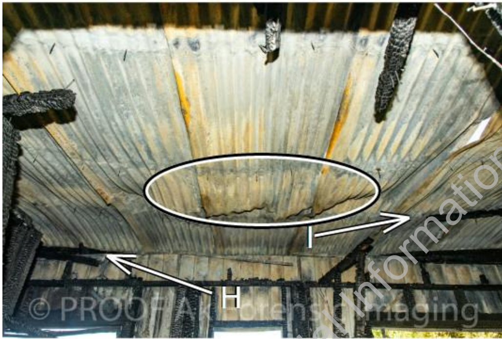
Photograph 34: Roof in the area of origin (Bedroom 2). Arrow I timber roof purlins consumed by fire. Circle indicating Roofing iron starting to bow. Arrow H Wall plates consumed by fire. (Courtesy of Police)
