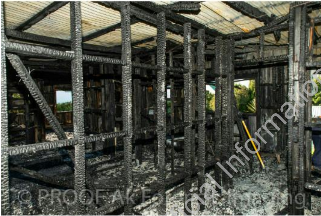
Photograph 33: Hallway area leading to bedrooms and area of origin. (Courtesy of Police)
