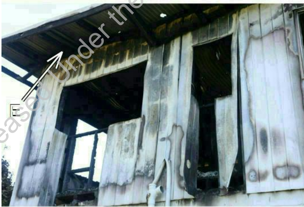
Photograph 7: Arrow E indicating soffit and timber support beams in the area of origin consumed by fire.
