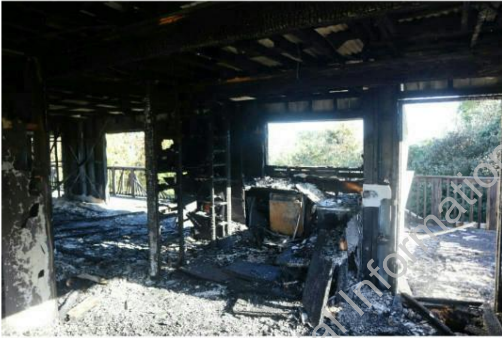
Photograph 28: Kitchen/Living area on upper level. Area of least damage.
