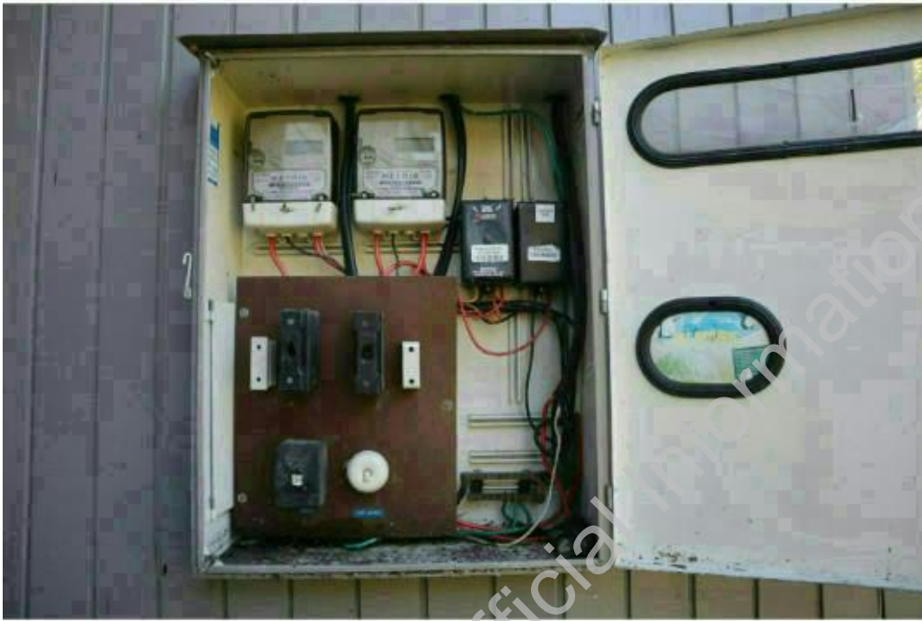
Photograph 8: Mains power meter undamaged.
