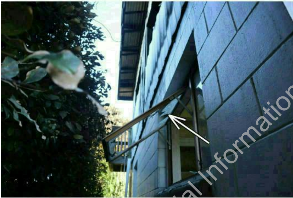
Photograph 3: Mechanical window break on lower level.
