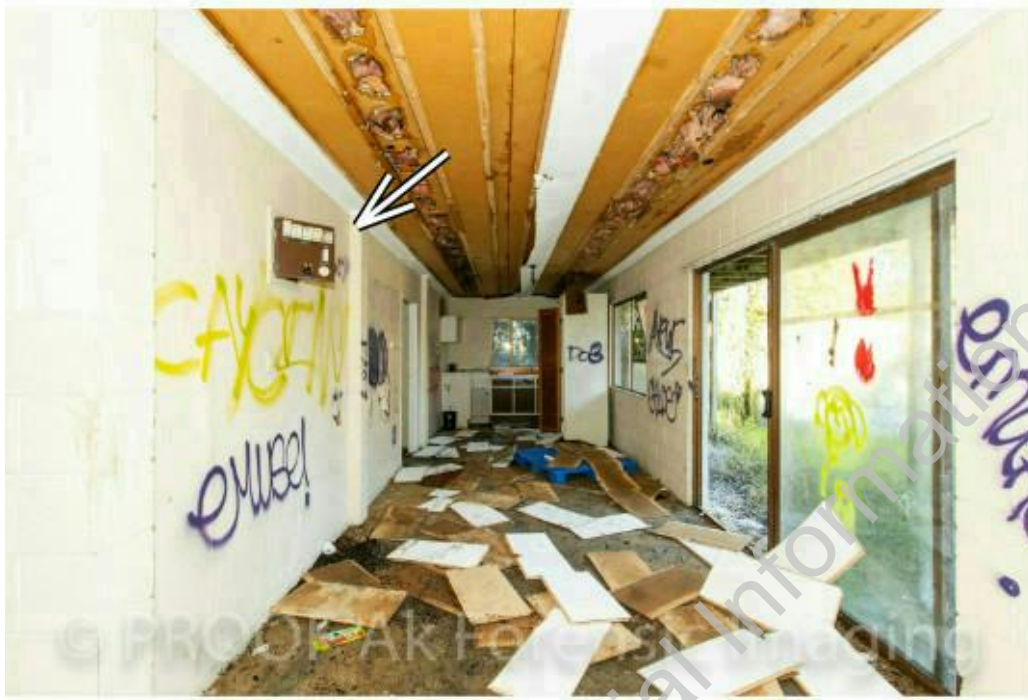
Photograph 19: Living area on the lower ground floor. Arrow indicating located of the fuse board. (Courtesy of Police)
