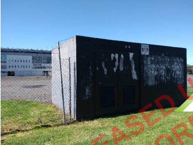
Figure 3 Transformer on northern boundary of site, facing south
