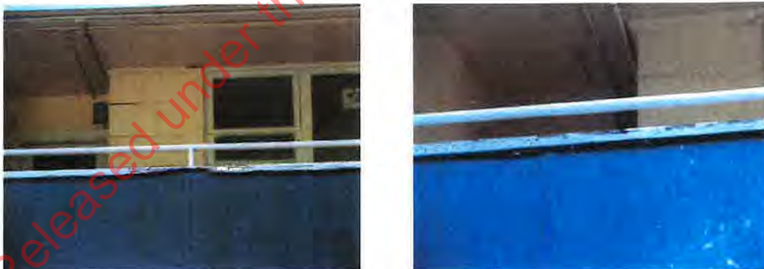
Rotting Top Timber Railing to Balustrade
