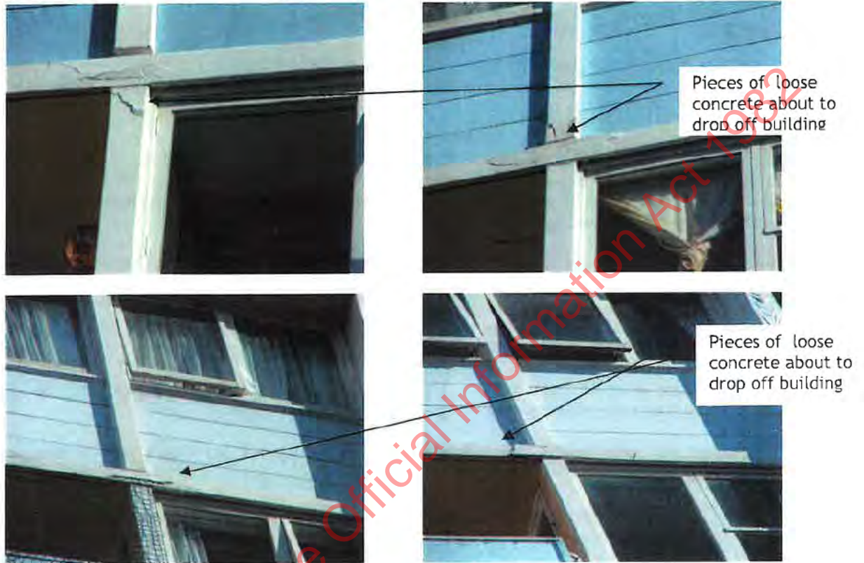
Front Façade - Concrete About to Spall
