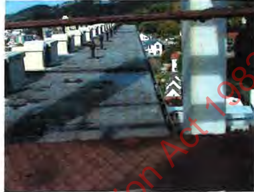
Upper Roof Needs Replacement
