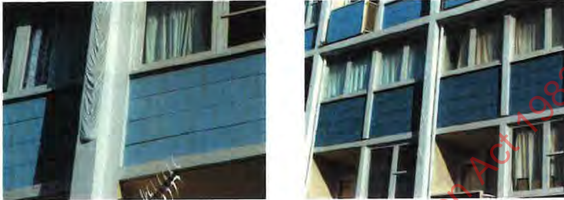
Failure of Paint System (Delaminating).
