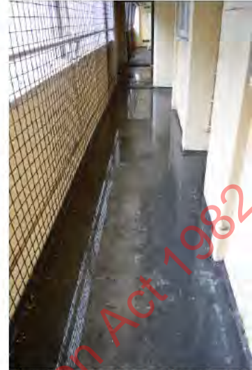
Figure 71. Looking at the extent of flooding on the First Floor level. (Archifact-Architecture & Conservation Ltd., 2014)
