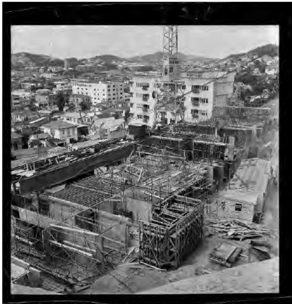
Figure 6. Gordon Wilson Flats under construction, The Terrace, Wellington. Negatives of the Evening Post newspaper. Ref: EP/1957/0397-F. Alexander Turnbull Library, Wellington, New Zealand. http://natlib.govt.nz/records/23171607
