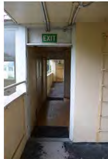
Figure 45. Looking into a typical junction along the walkway that leads into lift lobby for that level. (Archifac-Architecture & Conservation Ltd., 2014)
