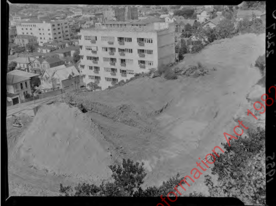
Figure 5: McLean Flats with earthworks for Gordon Wilson Flats, 1955. EP/1955/2247-F, Alexander Turnbull Library, Wellington. Note that the image shows the McLean Flats prior to the enclosure of their north-facing balconies.
