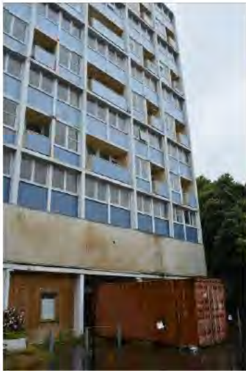
Figure 27. Looking at the northern end of the eastern elevation. Note the steel shipping container slotted into the main entrance to protect visitors from falling debris. (Archifact-Architecture & Conservation Ltd., 2014)
