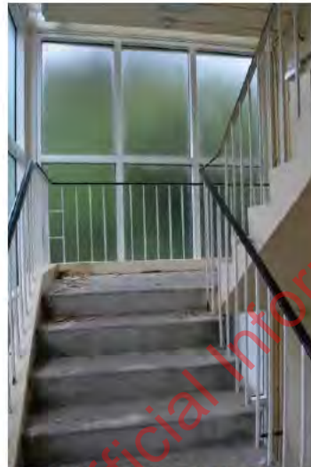
Figure 41. Looking at a typical stairwell positioned at the north and south ends of the building. (Archifac-Architecture & Conservation Ltd., 2014)
