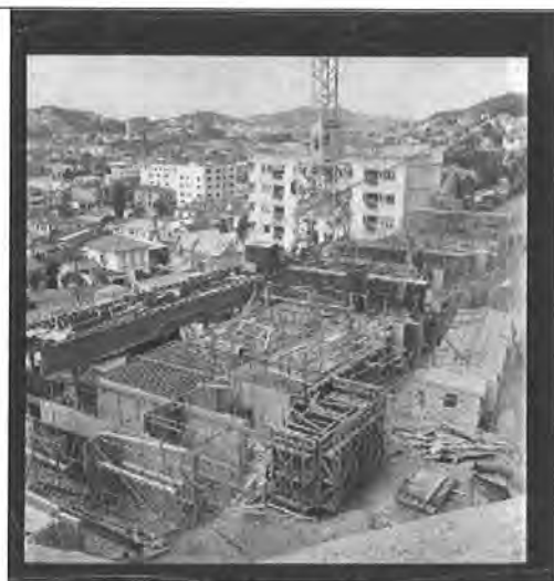
Gordon Wilson Flats under construction circa 11 February 1957. The McLean State Flats are behind the Downer crane. Evening Post . (Timeframes EP/1957/0397-F)
