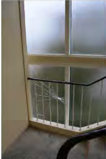
Figure 69. Looking at broken glazing within the southern stairwell. (Archifact-Architecture & Conservation Ltd., 2014)
