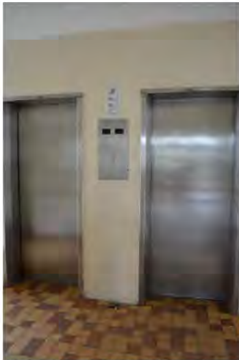
Figure 40. Looking at the main passenger lift entrance lobby at Ground Floor level. (Archifac-Architecture & Conservation Ltd., 2014)
