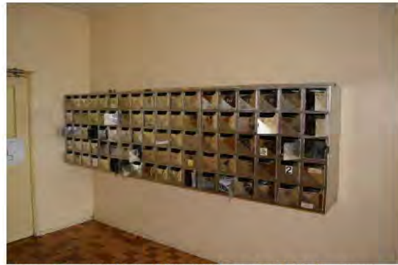
Figure 39. Looking at the stainless steel letterbox array within the main entrance lobby. (Archifac-Architecture & Conservation Ltd., 2014)
