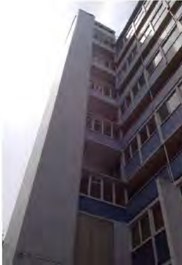
Figure 21. Looking north at the left tower and its junction with the west elevation. (Archifact-Architecture & Conservation Ltd., 2014)
