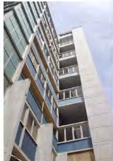
Figure 20. Looking south towards the lift tower and its junction with the west elevation. (Archifactor-Architecture & Conservation Ltd., 2014)
