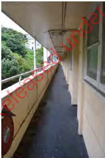
Figure 43. Looking north along a typical balcony walkway providing access to flats. (Archifac-Architecture & Conservation Ltd., 2014)
