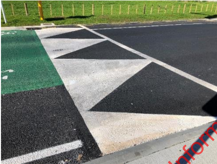
Figure 3: Sharks' Teeth on approach ramp (southbound lane)
