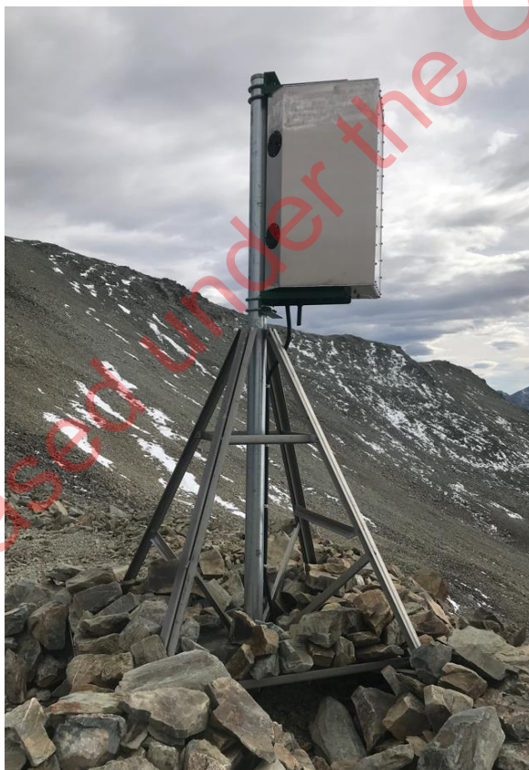
Figure 20- Wi-fi link tower
