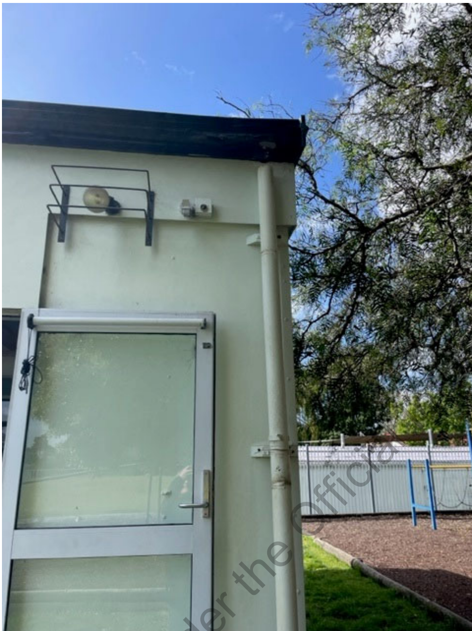
Block I Guttering and Asbestos issue
