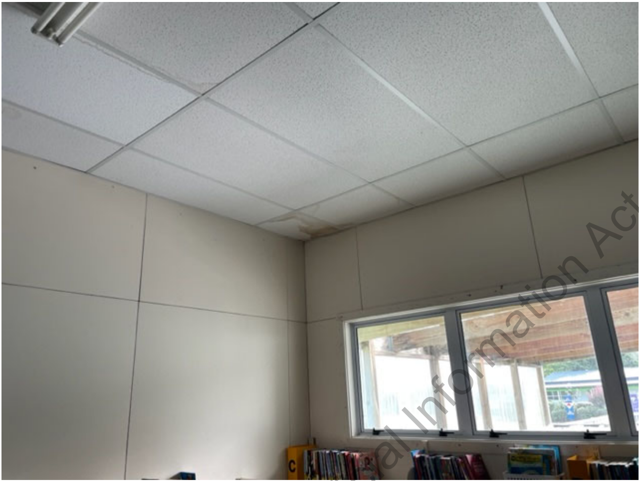
Block E Ceiling issues
