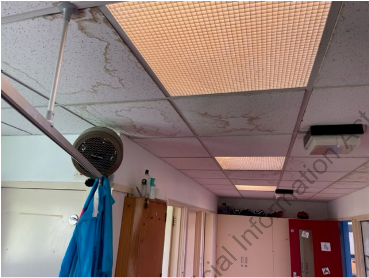
Block E Special needs Ablutions Ceiling issues
