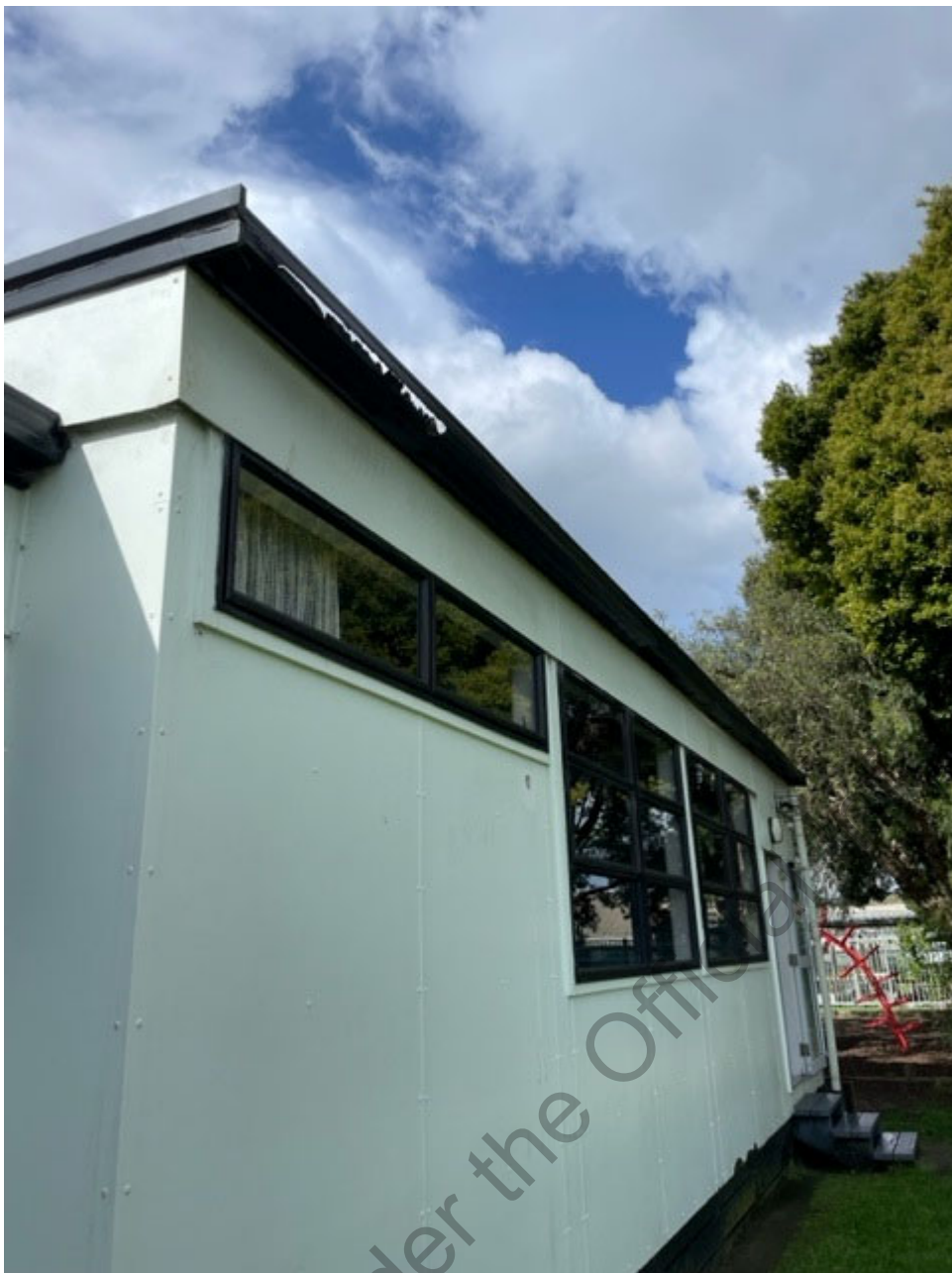
Block I - Downpipes used to connect to guttering
