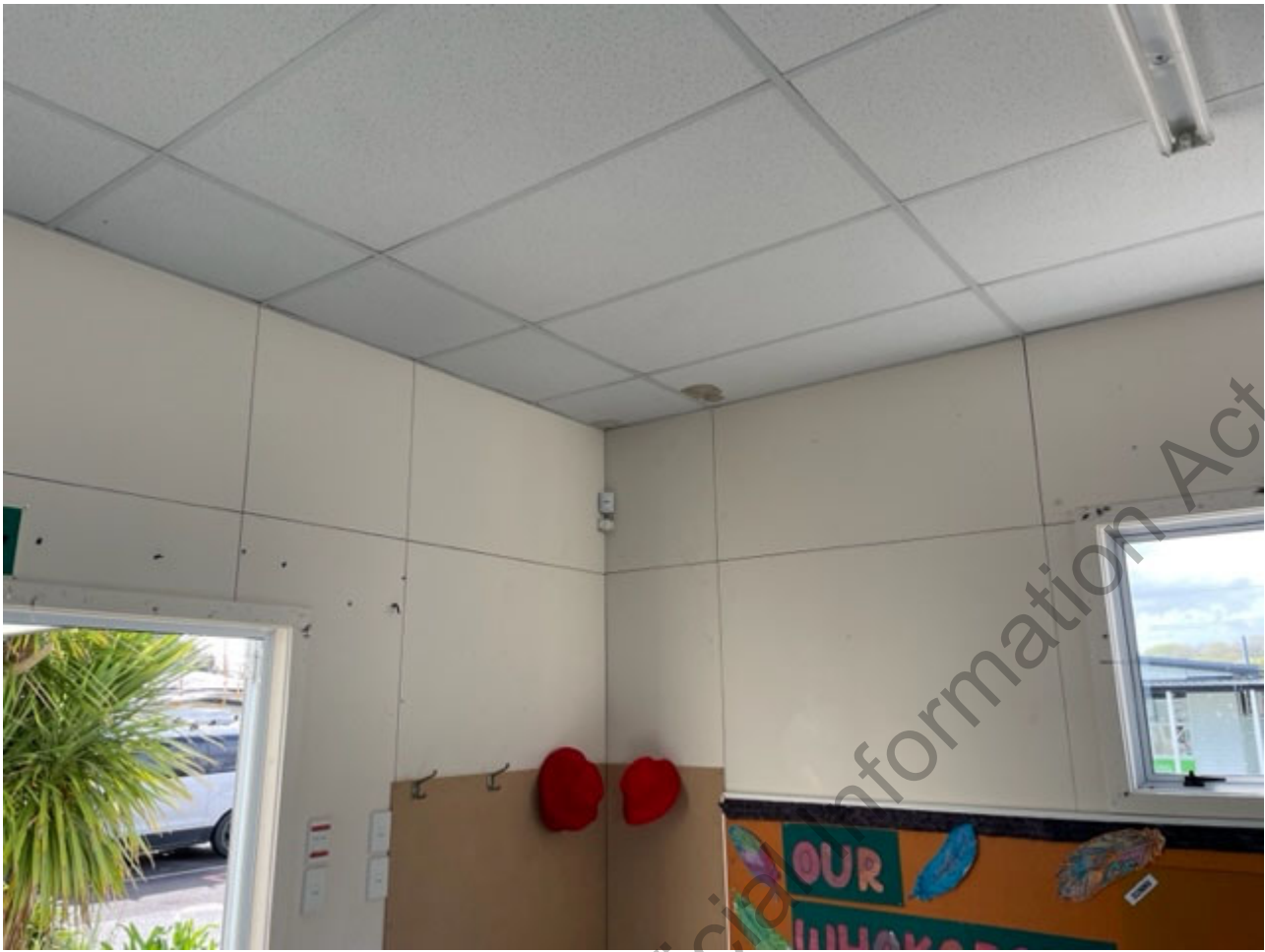
Block E Ceiling issues
