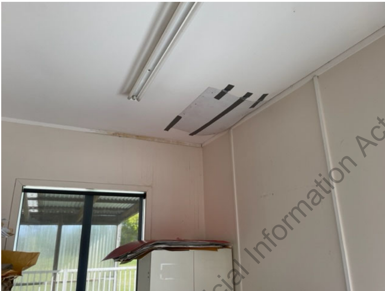
Block E Special needs Ablutions Ceiling issues
