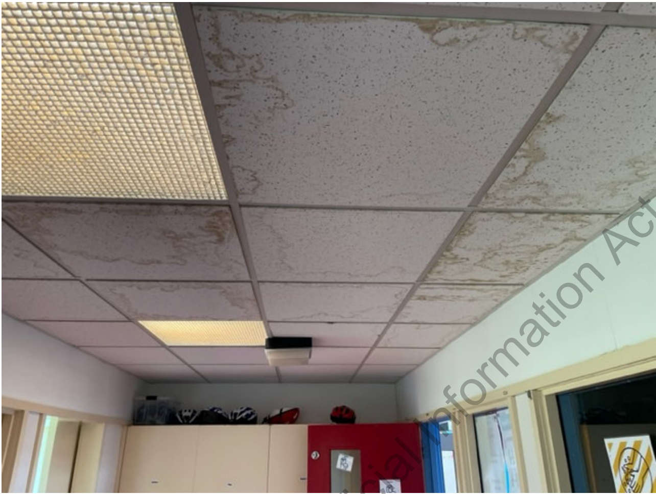
Block E Special needs Ablutions Ceiling issues
