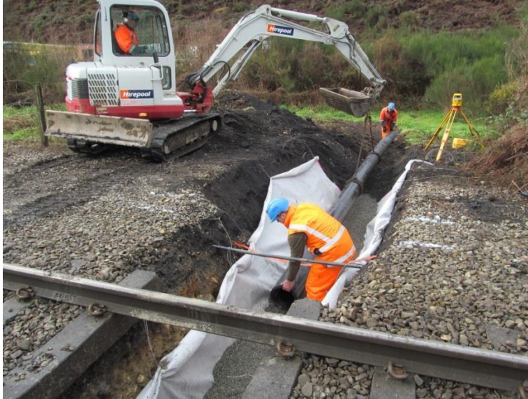
Figure 7:21 Installation of approved PH carrier pipe under main line, Reefton Yard, SNL
