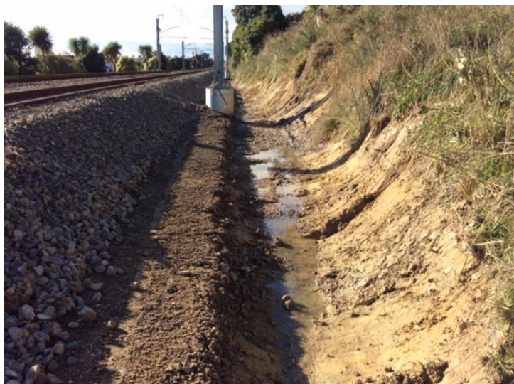
Figure 7:10 Cess/formation shoulder and V type drain at base of slope at 47km NIMT
