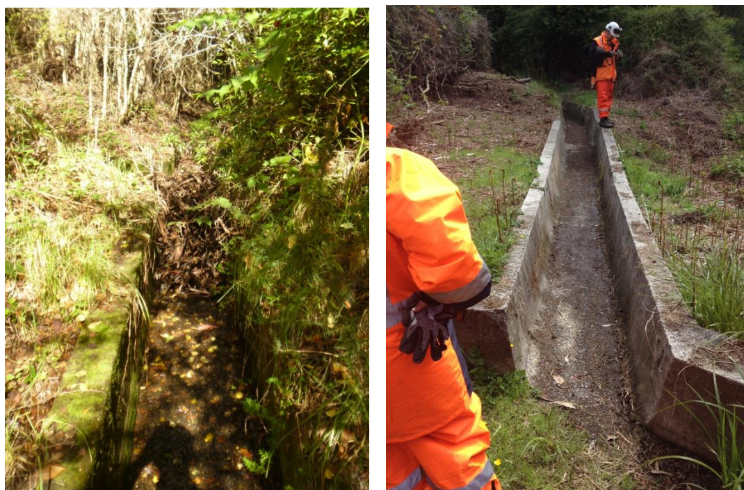
Figure 7:6 Interceptor drain above 389km MSL blocked and then after cleaning
