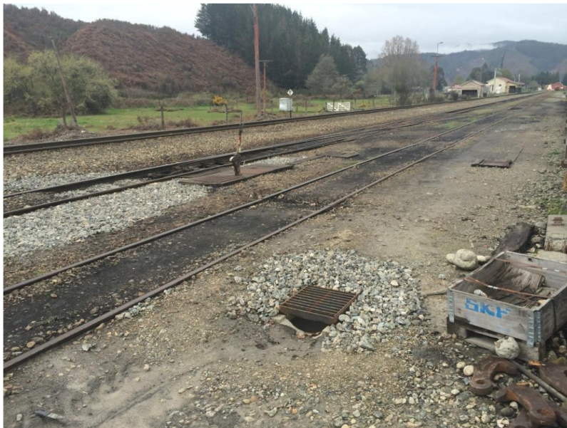
Figure 7:22 Grated sump, Reefton Yard, SNL
