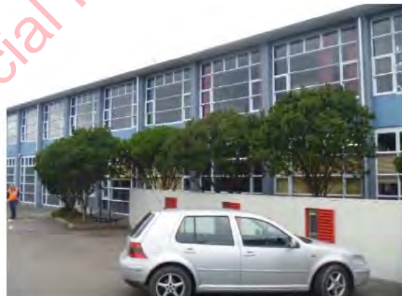
Photo 4: West elevation having additional perimeter columns at ground floor to line up with original perimeter columns at first floor level
