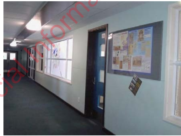
Photo 18: Corridor at 1 st floor towards the east elevation with the new timber wall additions
