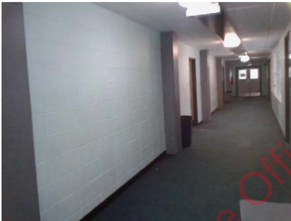
Photo 17: Corridor at 1 st floor towards west elevation with the original concrete block walls
