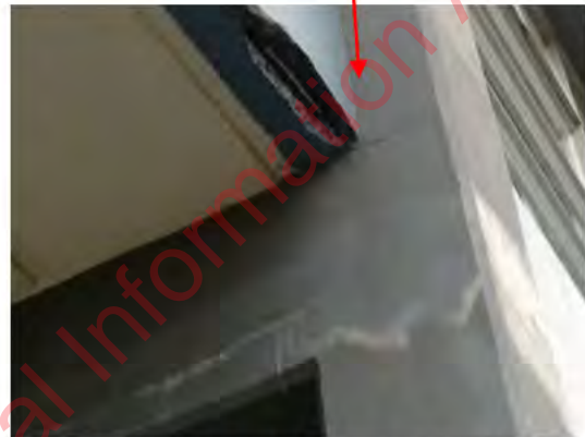
Photo 6: Details of the concrete spalling at first floor level and the horizontal cracking of the additional perimeter columns at ground level
