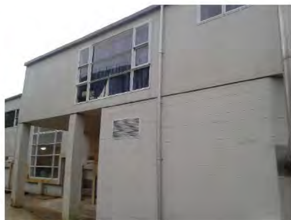
Photo 8: View of the concrete block walls at ground and metal cladding with timber framing at first floor.
