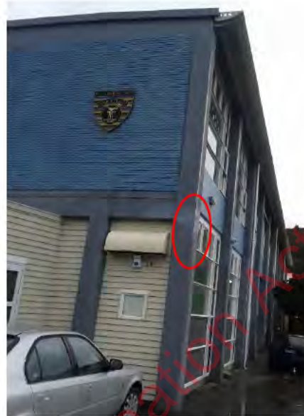
Photo 2: North-west corner elevation showing cracking at the additional column on west elevation
