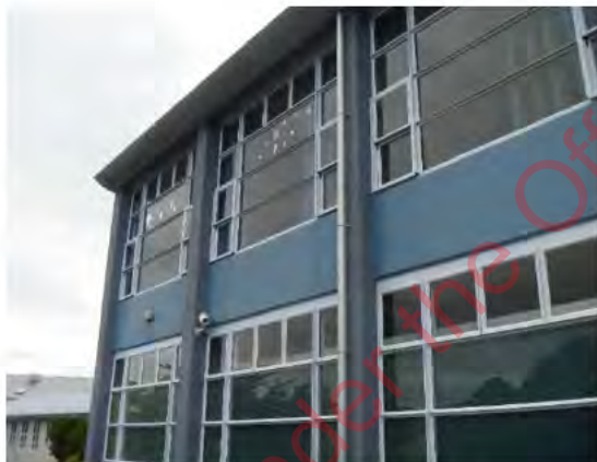
Photo 3: North end of West elevation with the short height of precast panels only at first floor level
