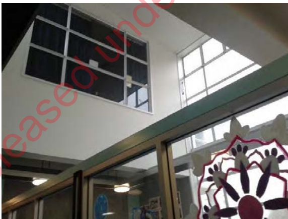
Photo 19: Opening/ floor void facing towards the east elevation with part of the addition at 1 st floor
