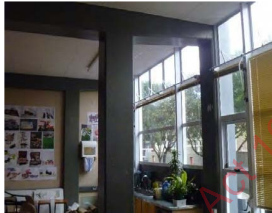
Photo 16: Concrete frame at ground floor towards the west end with the new column along perimeter
