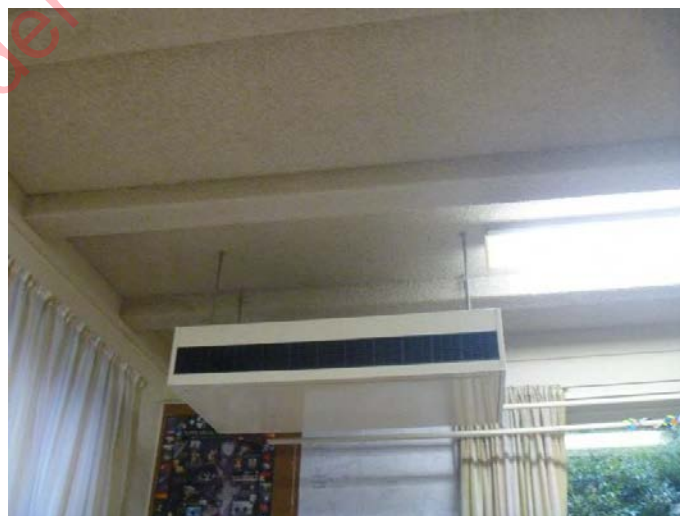
Figure 3: Heater in ground floor classroom
