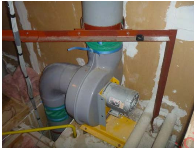
Figure 8: Extractor fan and exhaust support
