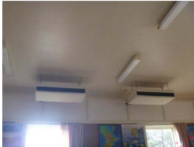
Figure 4: Heaters in first floor classroom
