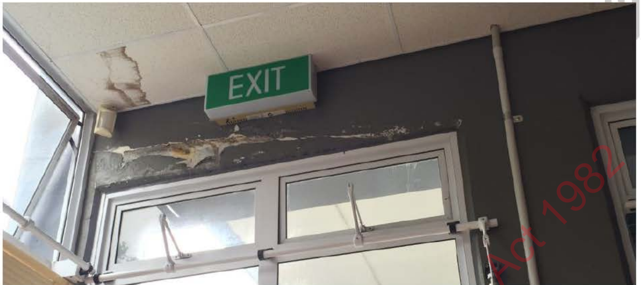
Picture 1 - Typical example of damage at junction between new/original concrete.
