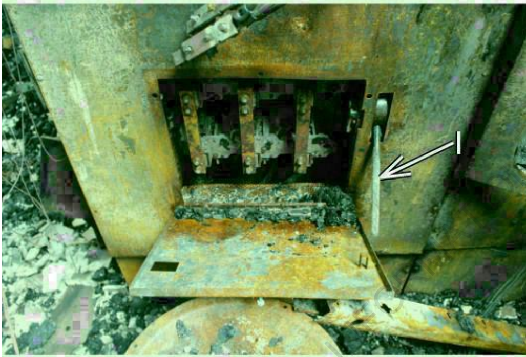
Photo 32. "I" Main electrical distribution cabinet lever was in the "Off" position.
