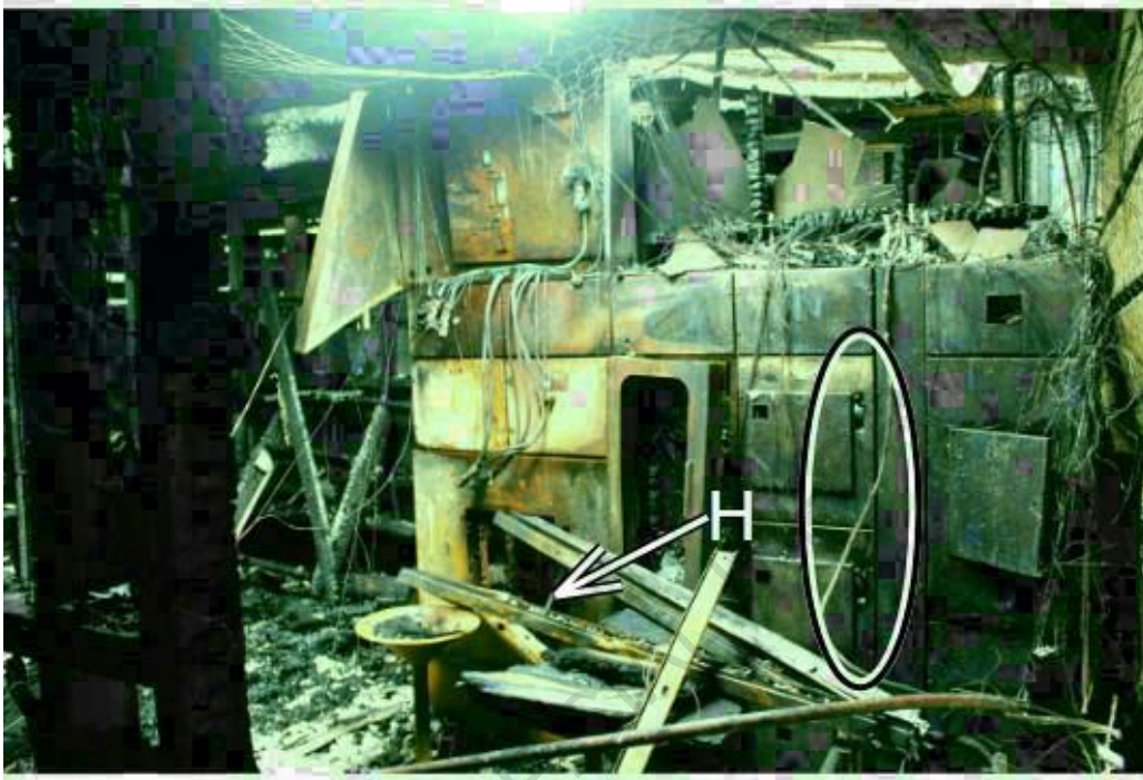
Photo 31: Tavern electrical distribution cabinet. "H" is the leading electrical on/off lever. The oval depicts the two subsidiary levers in the "On" position.
