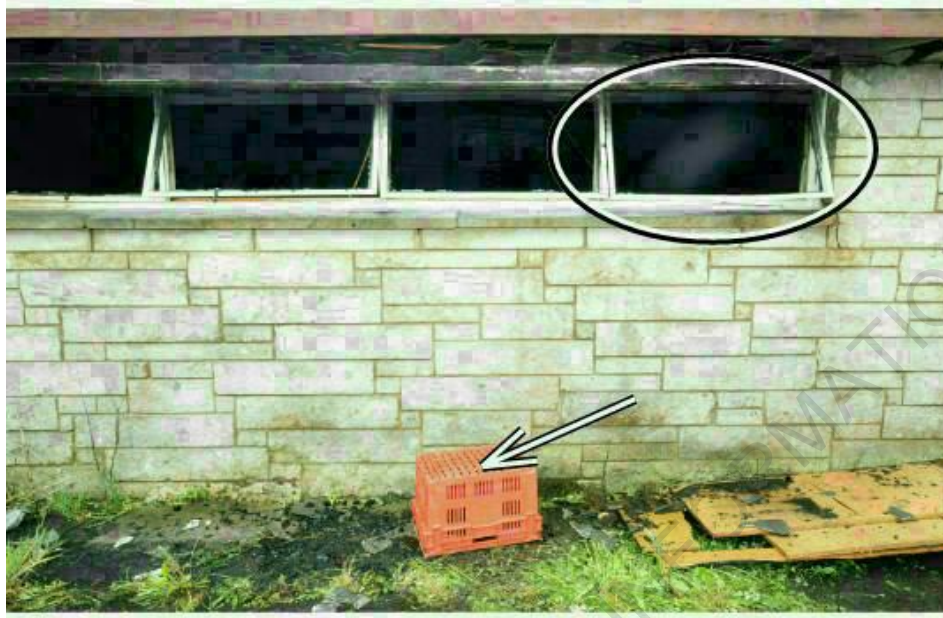
Photo 15: Right damaged aluminium window sash. The arrow depicts a red plastic crate. (Photo courtesy of Police).
