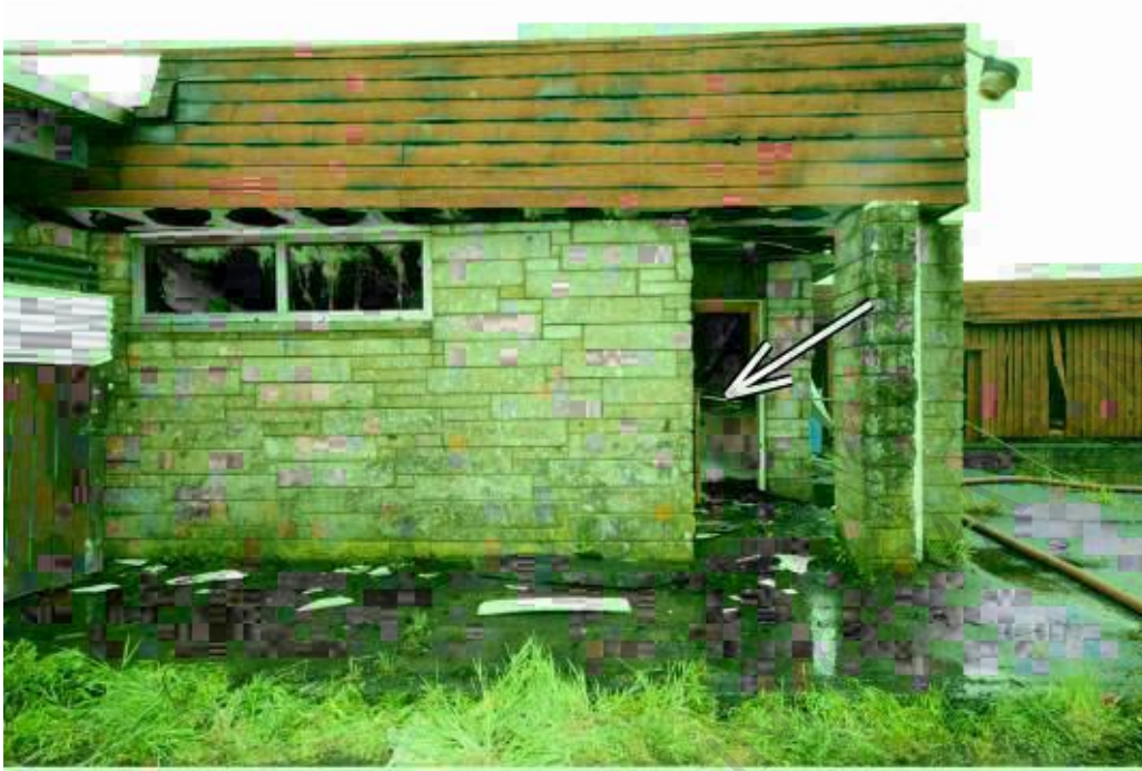
Photo 8: Single door forced opened by firefighters. Arrow depicting damaged door. (Photo courtesy of Police.)
