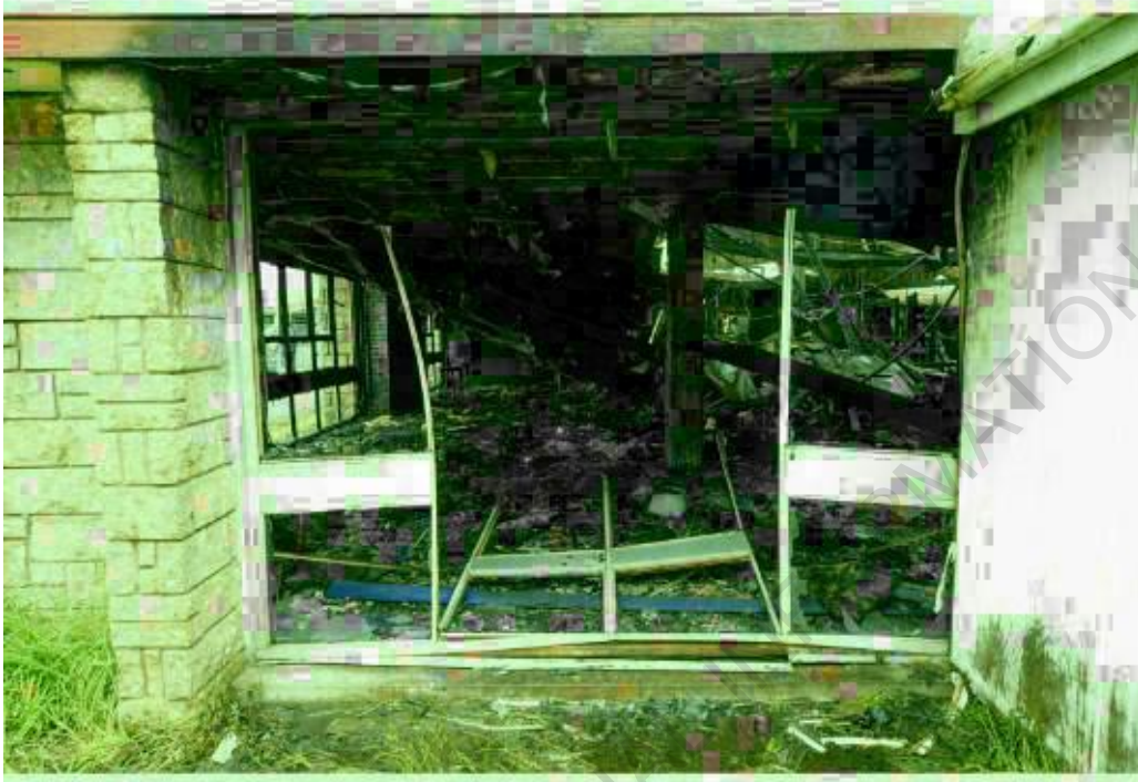
Photo 18: View of the aluminium window and interior of Club 865. (Photo courtesy of Police).
