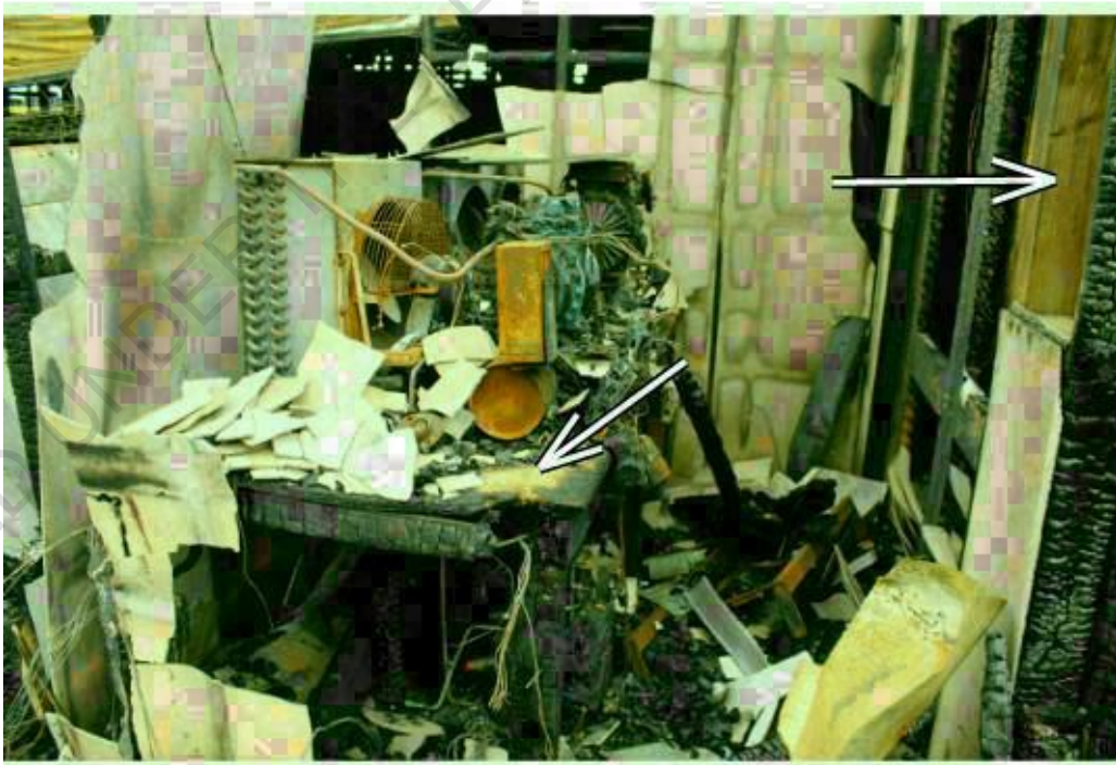
Photo 28: Arrows depicting timber and shelving that was not fire damaged.
