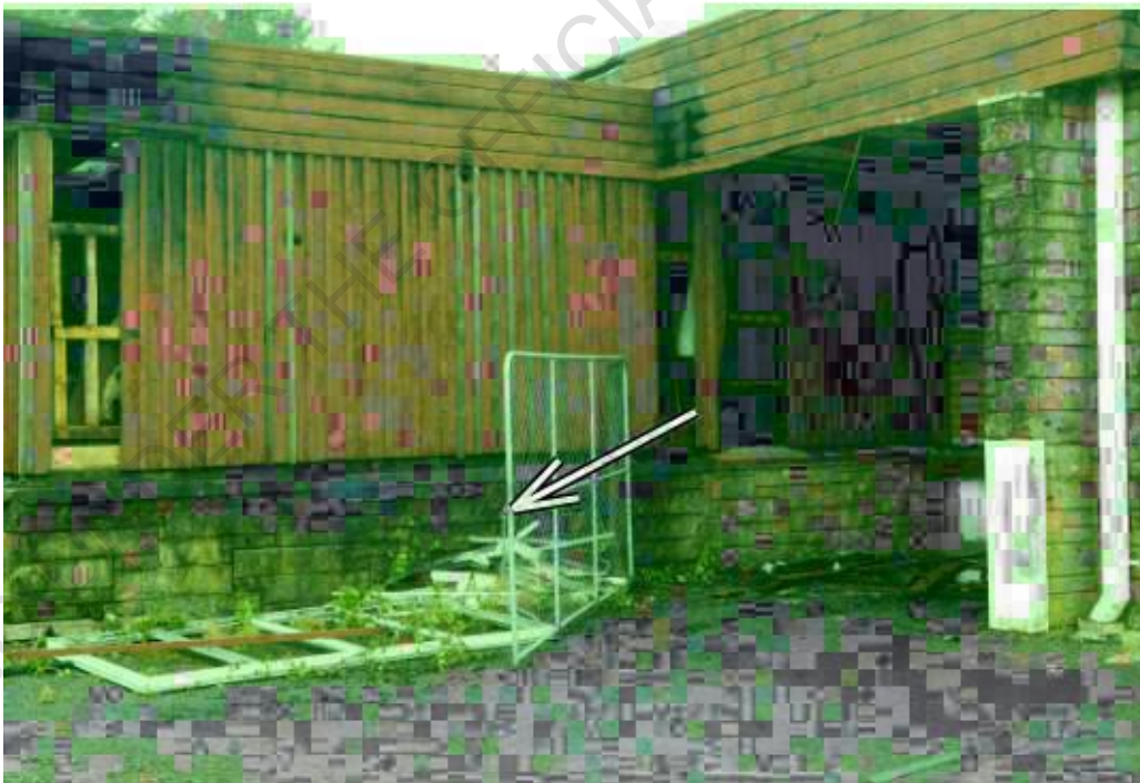
Photo 13: The gate chain was cut prior to fire fighters arrival. Northwest corner of the tavern. (Photo courtesy of Police.)
