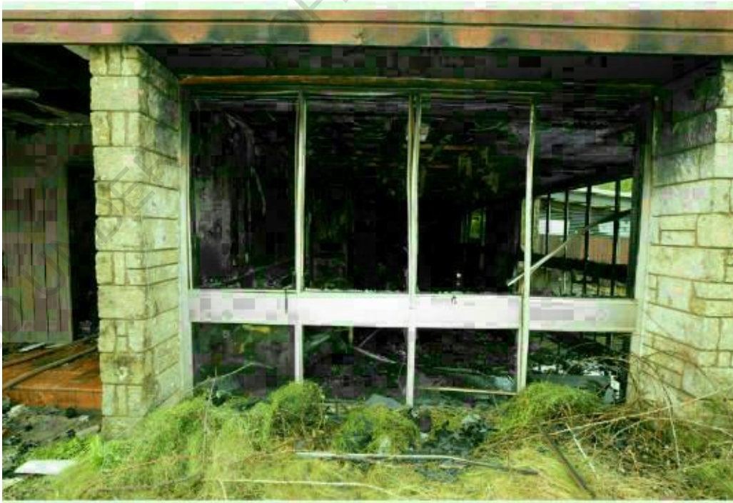
Photo 25: Exterior aluminium of restaurant. Photo courtesy of Police.
