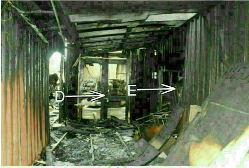
Photo 11: "D" refrigeration/generator. "E" Entrance doors to storeroom.
