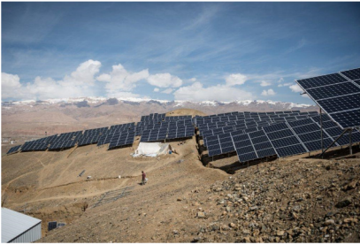
Solar panel arrays built by New Zealand
