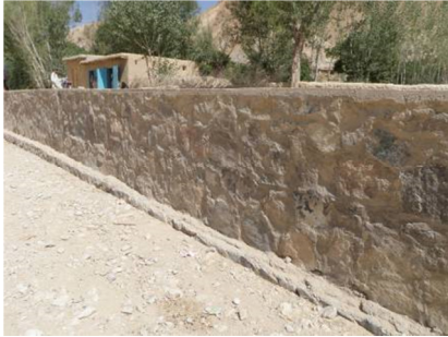
A flood protection wall at De Himan village built with NZDF assistance
