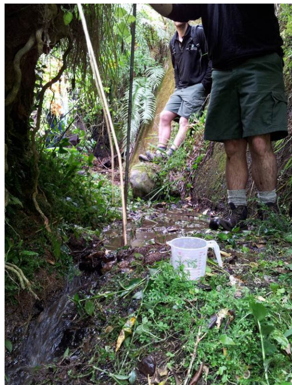
Photo 8: Seepage flow from beneath spillway chute and dam toe approximately 12 litres per min.
