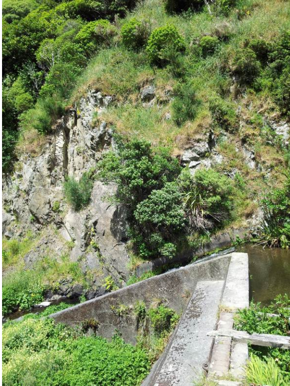
Photo 17: Woollen Mills dam crest, spillway chute wall and right abutment. Note rock-fall middle left in photo.
