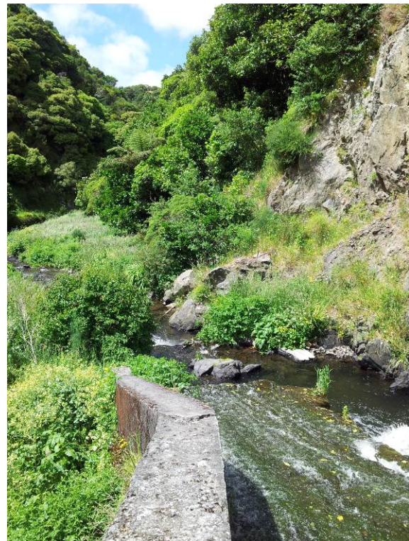
Photo 16: Woollen Mills spillway chute and wall looking downstream. Note rock-fall upper right in photo.
