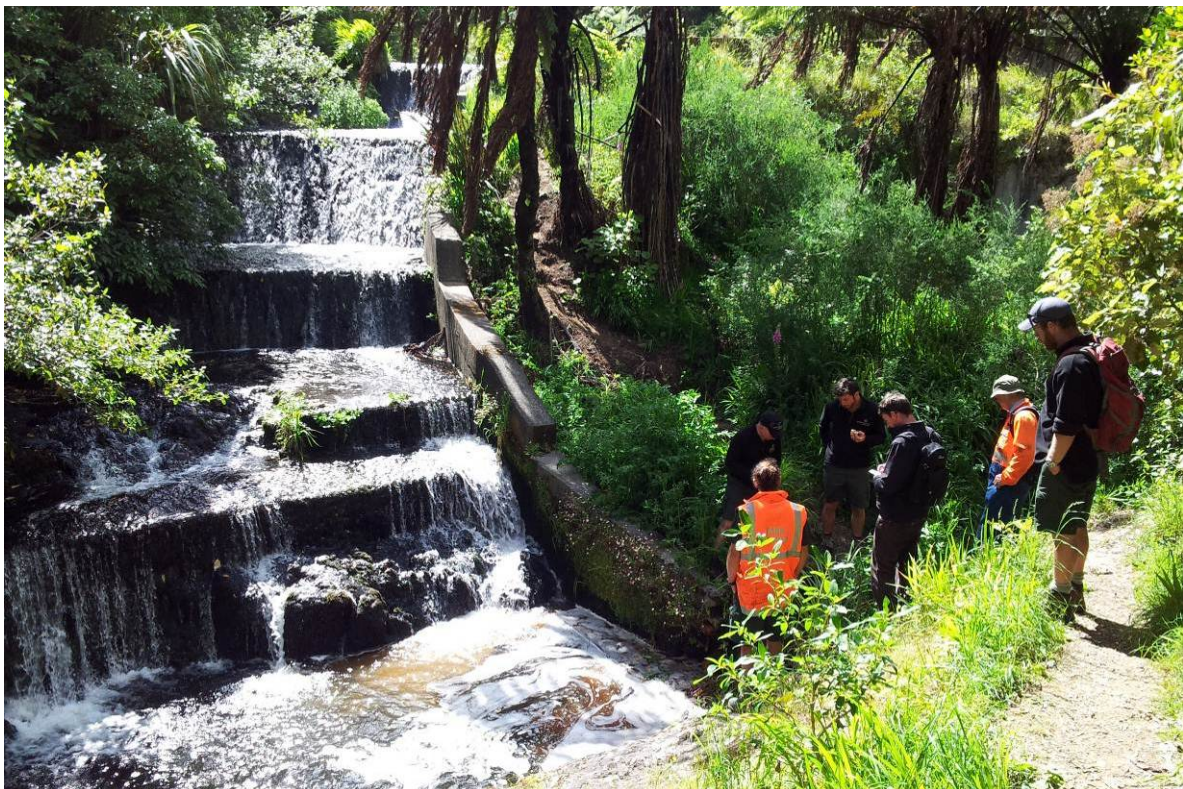
Photo 11: Spillway chute, plunge pool and downstream toe. Outlet pipe amongst people standing right of middle.
