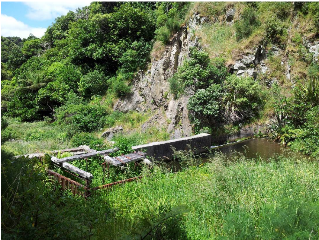
Photo 13: Woollen Mills dam and reservoir looking from upstream left abutment toward downstream right abutment. Note that the impounded reservoir is very small.
