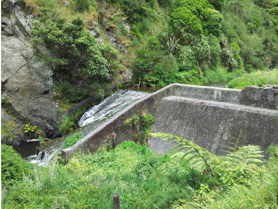
Photo 23: Woollen Mills spillway and dam looking upstream from downstream left abutment. Note damaged spillway chute and visible extent of upstream regression.
