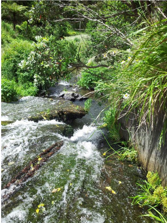
Photo 19: Spillway chute looking toward plunge pool. Note chute damage and overhanging vegetation.
