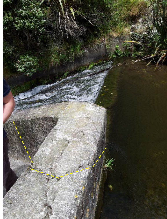
Photo 18: Woollen Mills spillway crest and chute. Crack extends down spillway wall, across dam crest wall and down upstream face toward spillway crest.
