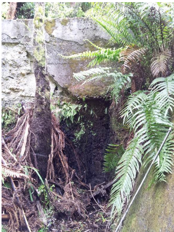
Photo 7: Seepage emerging from poor quality concrete beneath spillway chute.
