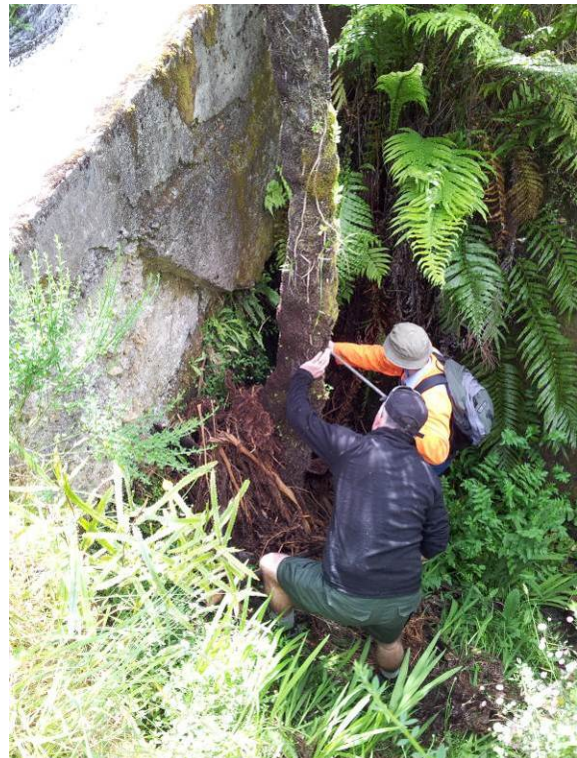
Photo 6: Seepage emerging from poor quality concrete beneath spillway chute.
