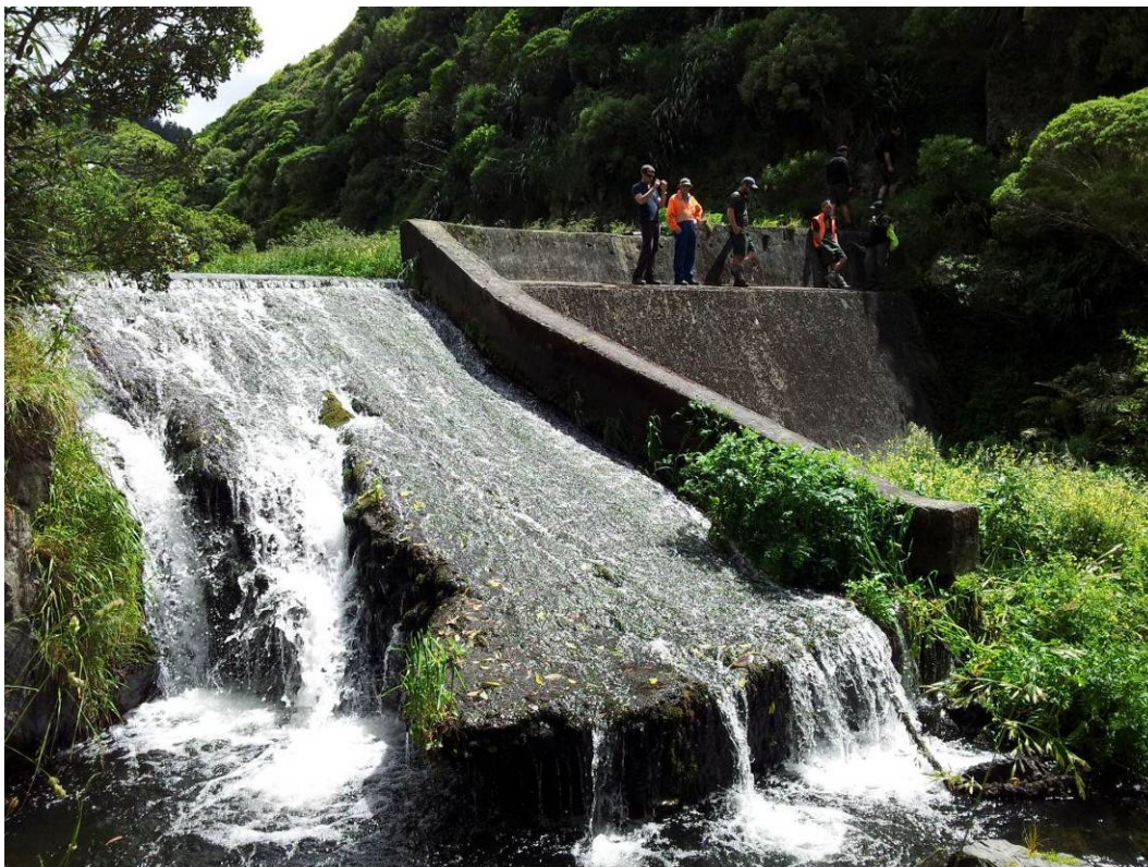
Photo 22: Woollen Mills spillway and dam looking upstream from toe of rock-fall. Note damaged spillway chute and major undermining. Probing with a long stick indicated a very large cavity under the remaining chute slab in centre photo. Cavity horizontal extent approx. 1.5m and depth approx. 2m.
