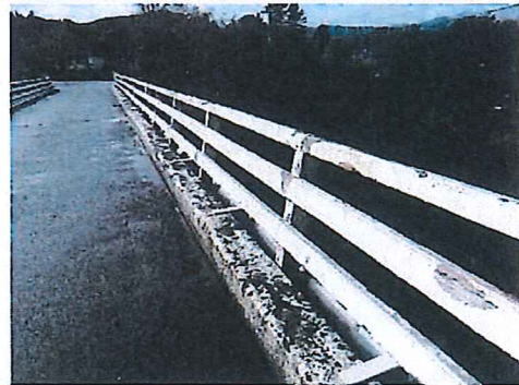
Repainting of timber kerbs and handrails required - No decay detected to the rails.
