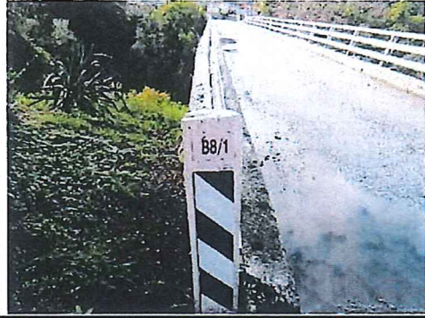
Ponding to right hand upstream approach.
