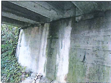
Left hand abutment - Note deck joint leaking.
