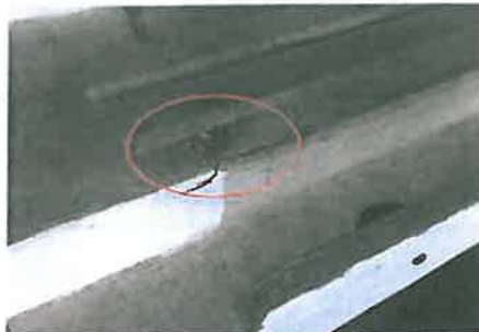
16. Location of cracks in patches of lower terrace seating
