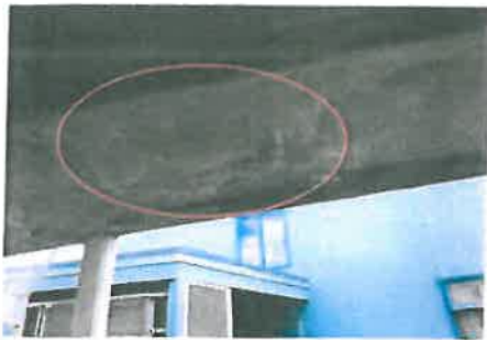
21. Location of cracks in patches in main beam under upper terrace
