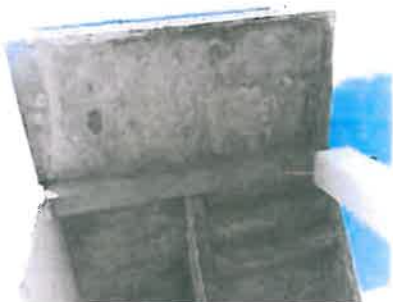
3. Location of cracks from upper South landing support beam
