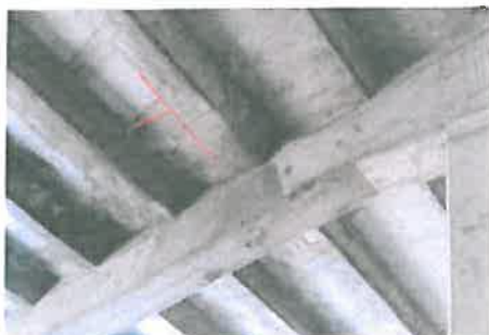
5. Location of cracks in upperside of upper terrace seating
