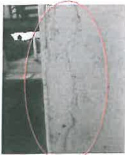
1. Location of crack in rear SW concrete column
