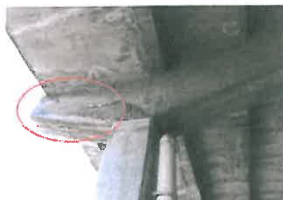
8. Location of cracks in patching of upper terrace beam
