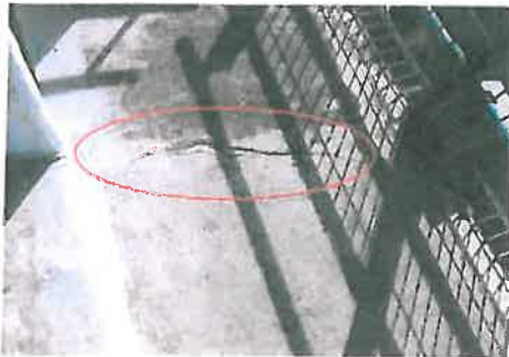
25. Location of cracks in upper deck
