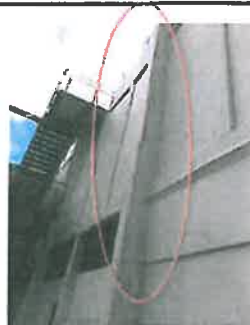
2. Location of crack in rear intermediate concrete column
