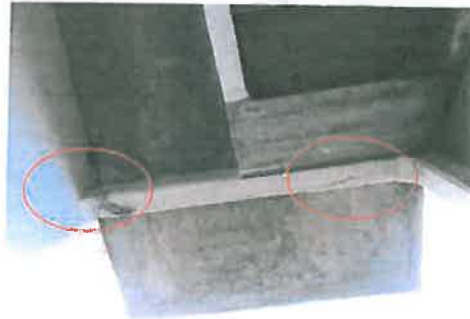
24. Location of failure cracks in upper Nth landing stair beam
