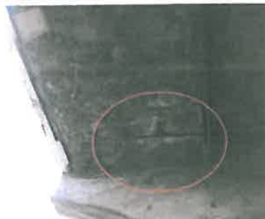
20. Location blown off cover concrete and rusting reinforcement in underside of upper terrace seating
