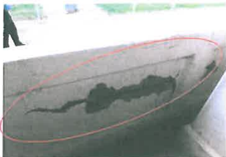
19. Location fallen off cover to rebar in lower seating front wall
