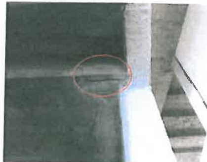
26. Location of cracks in exterior concrete stairs
