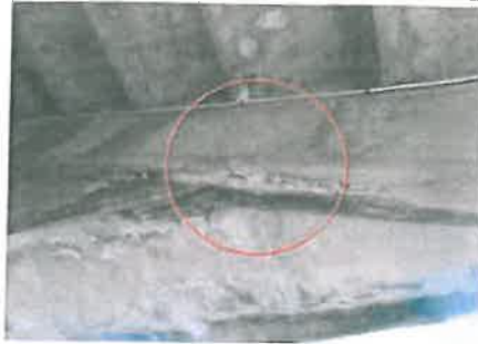
22. Location of cracks in main beam under upper terrace
