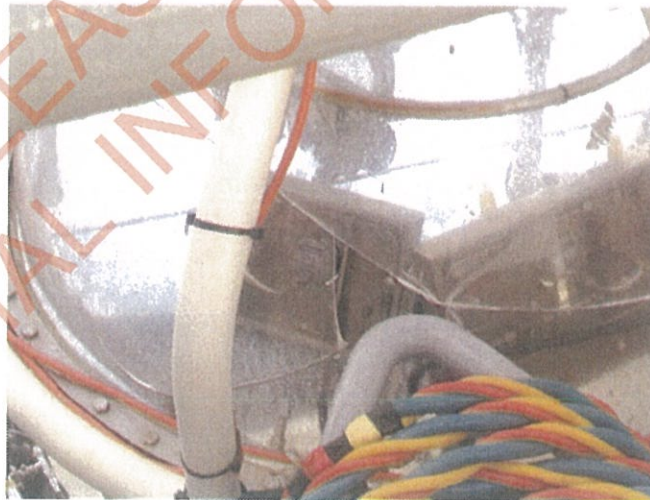
Figure 5: MAN Dive Bell damage
