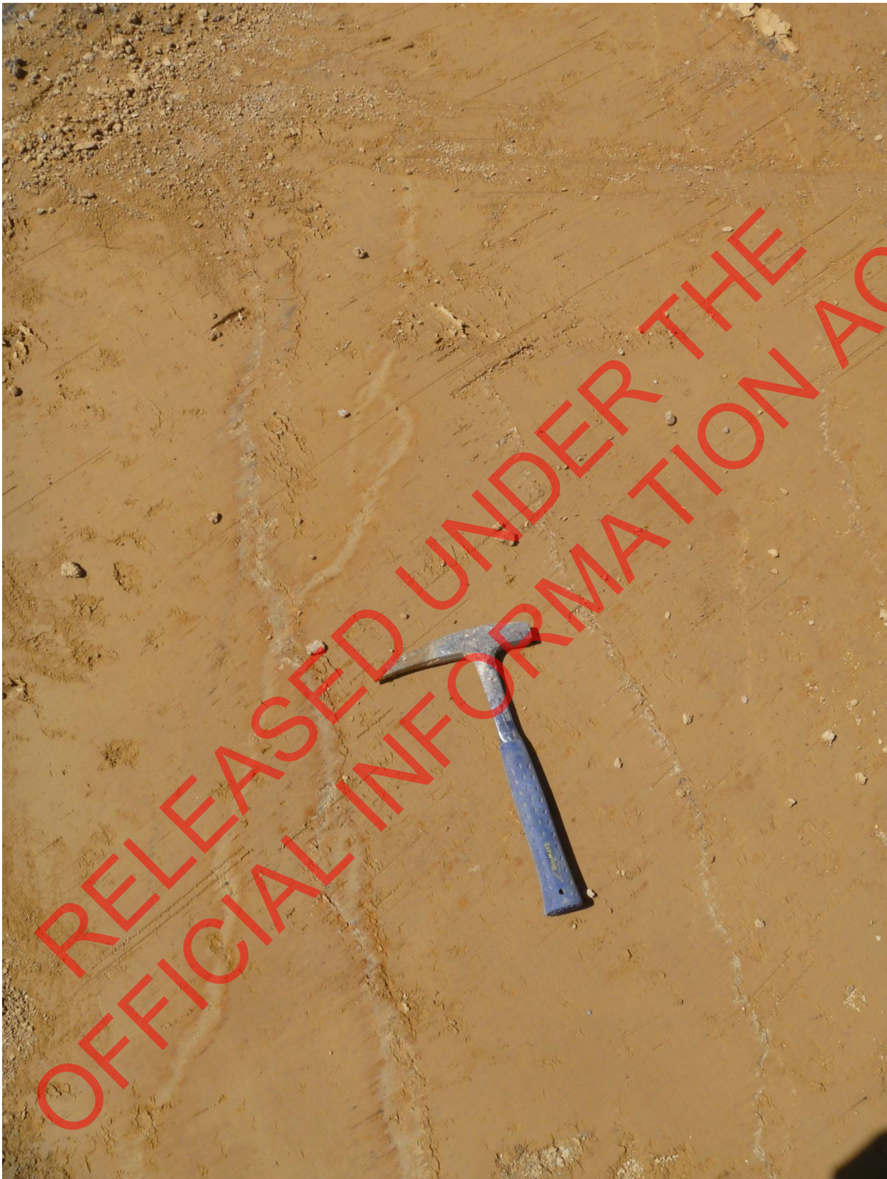
Photograph 17: Cross cutting cracks
