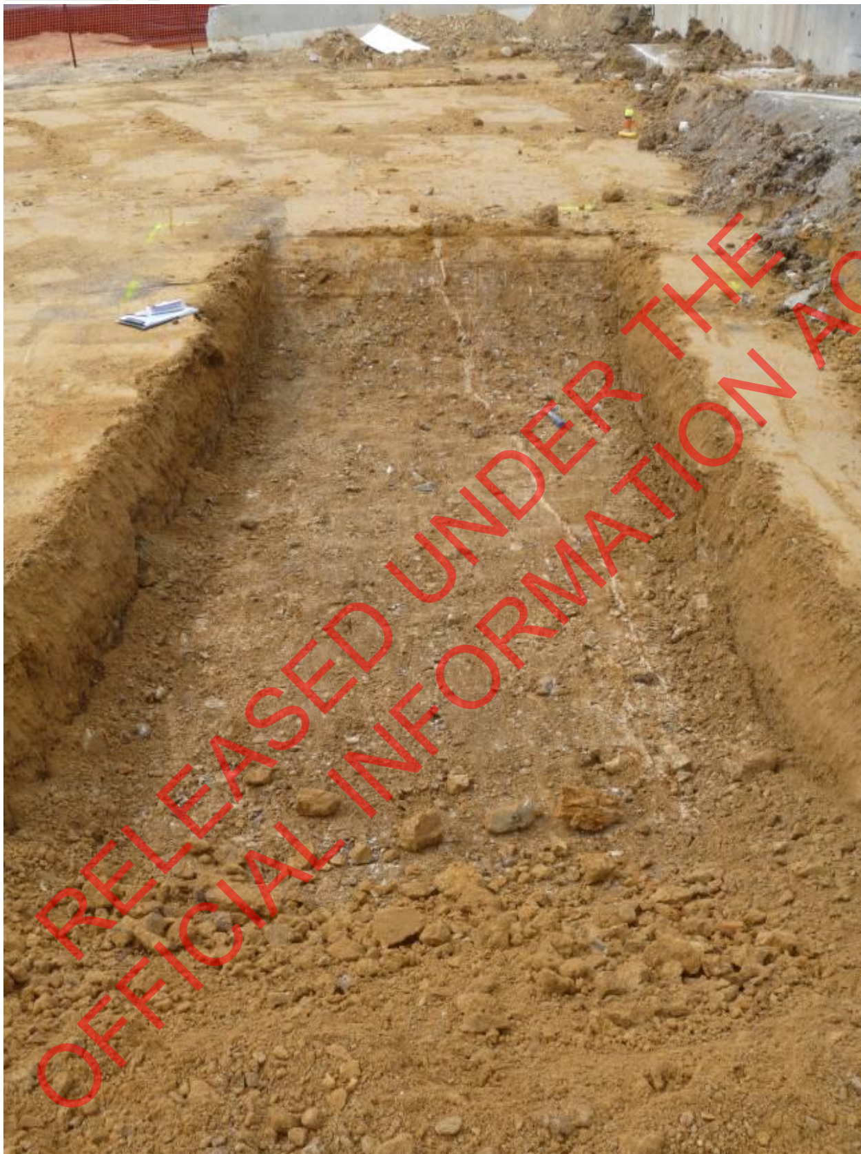
Photograph 10: Large crack extending into Layer 4
