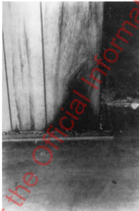
FIGURE 6.3.7.2.3 Inverted Cone Pattern Fueled by a Natural Gas Leak Below the Floor Level.
