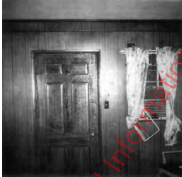
FIGURE 6.3.7.11.2.2 Blistering of Varnish on Door and Slight Scorching of Draperies, the Only Indications of the Natural Gas Flash Fire.
