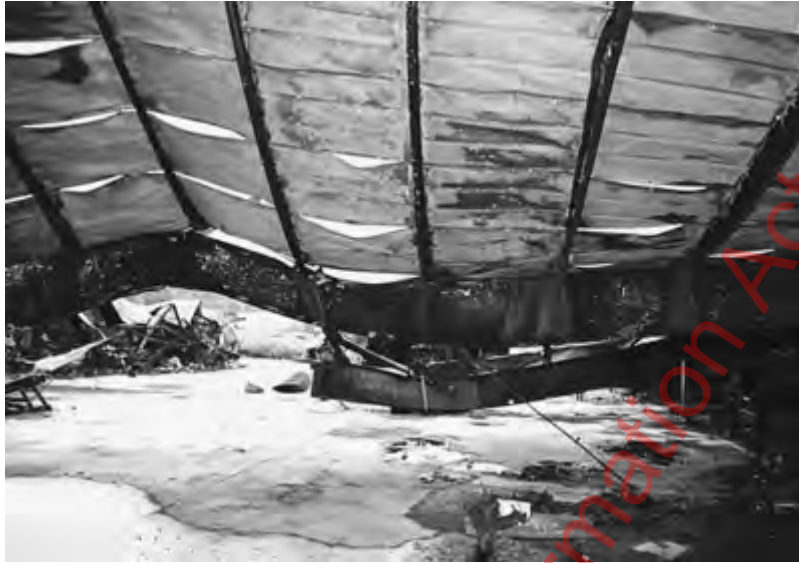
FIGURE 6.2.9.1 Steel I-Beam Girders Deformed by Heating Under Load.
