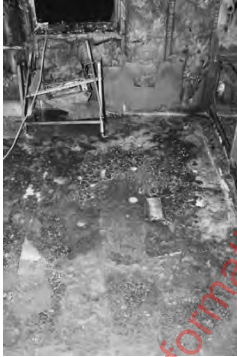
FIGURE 6.3.7.8.5(b) Fire Patterns on Linoleum Floor Resulting from Fully Developed (Post-Flashover) Fire in Full-Scale Test Burn of Residential Structure; No Ignitable Liquids Were Present.
