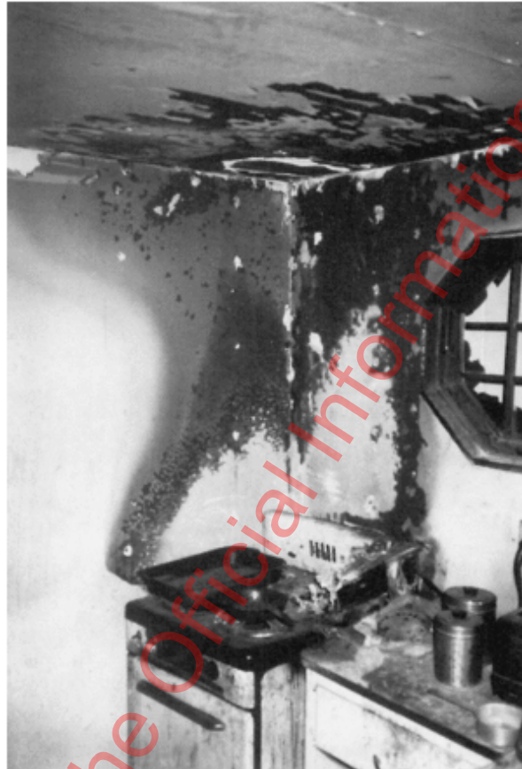
FIGURE 6.2.11 Clean Burn on Wall Surface.
