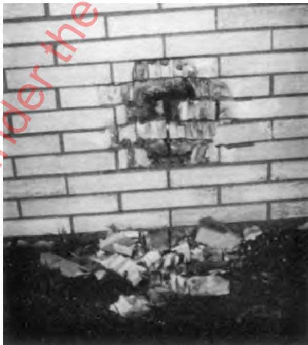
FIGURE 6.2.9.2 Damage to an Outside Brick Wall Caused by Thermal Expansion of an I-Beam in the Basement.
