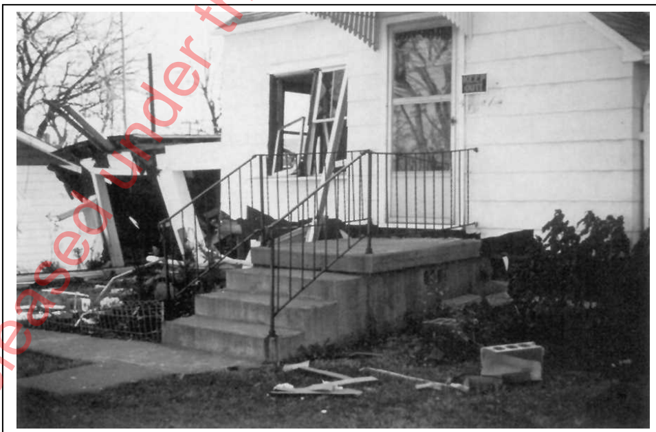
FIGURE 21.3.1 Low-Order Damage in a Dwelling.
