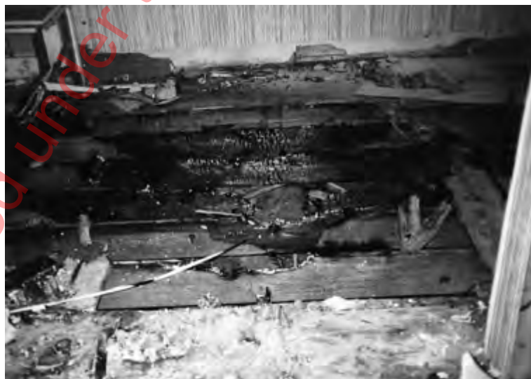
FIGURE 6.3.7.12 Saddle Burn in a Floor Joist.
