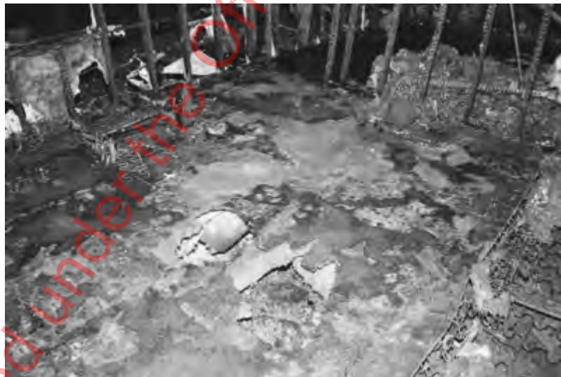
FIGURE 6.3.7.8.5(a) Fire Patterns on Floor Resulting from Fully Developed (Post-Flashover) Fire in Full Scale Test Burn of Residential Structure. Floor Was Carpeted and Room Had Typical Residential Furnishings; No Ignitable Liquids Were Present.
