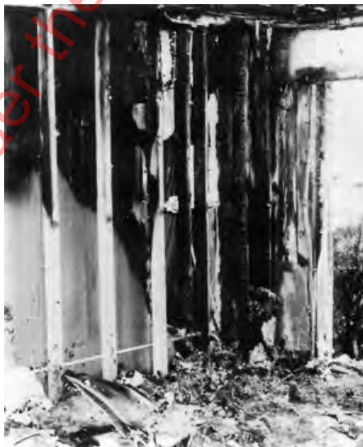
FIGURE 6.3.7.1(b) V Pattern Showing Wall and Wood Stud Damage.
