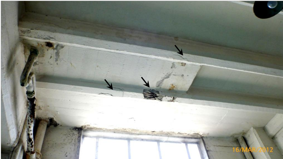
Figure 16. Spalling of the secondary beams that support the Distributing Gallery floor.
