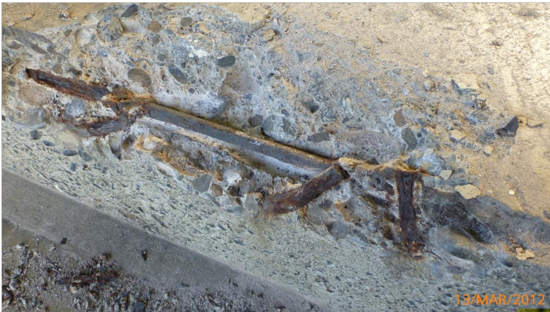
Figure 12. Corrosion along the top of bleacher riser beams as a result of a combination of poor concrete quality, consequent carbonation, and insufficient cover. Section loss on the principal reinforcement estimated as 30%.
