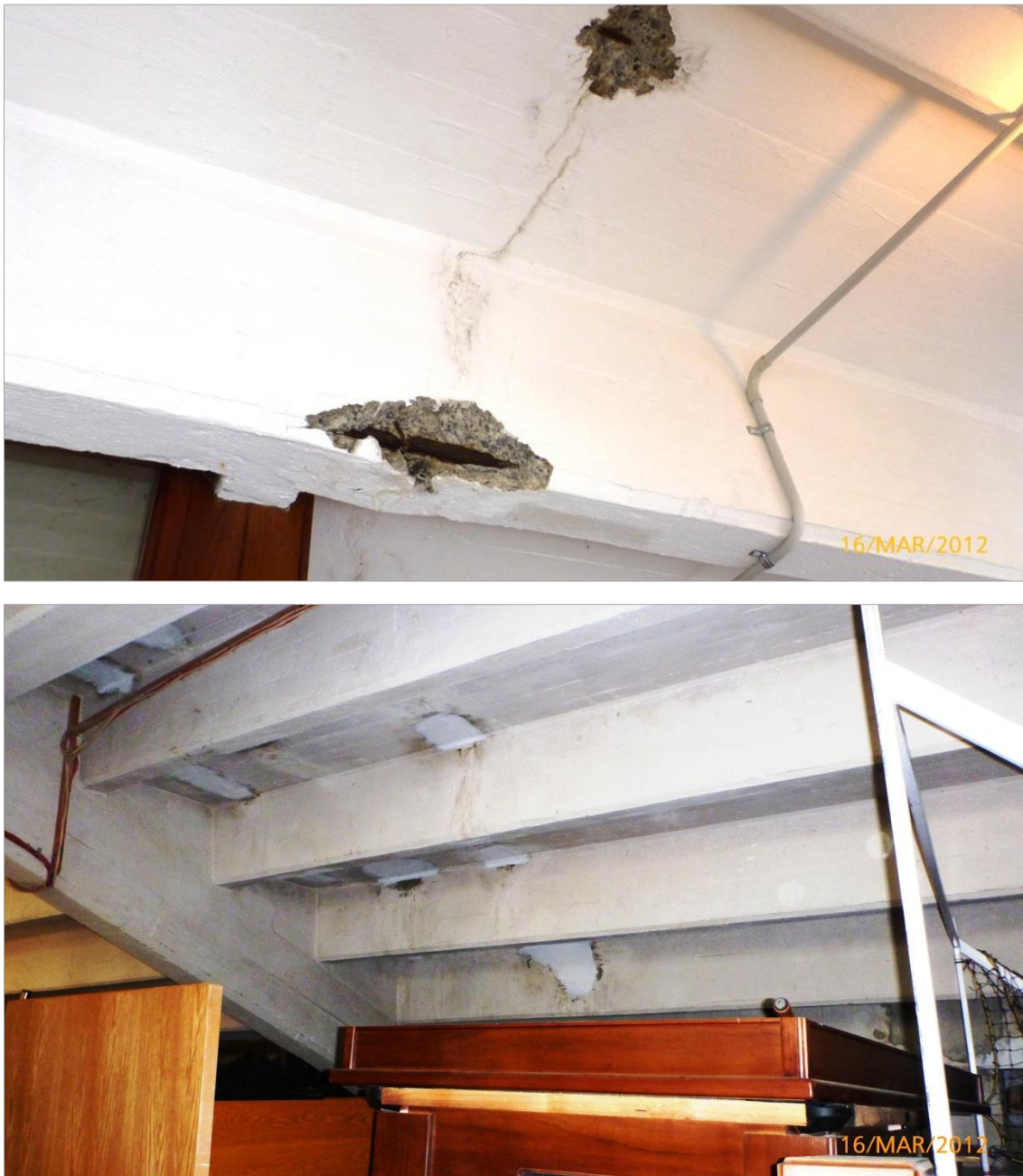
Figure 15. Examples of developing and patch repaired spalls on the undersides of riser beams. The spalls typically occur along the lines of shrinkage cracks or construction joints in the concrete that permit water entry from the exterior terraced seating.
