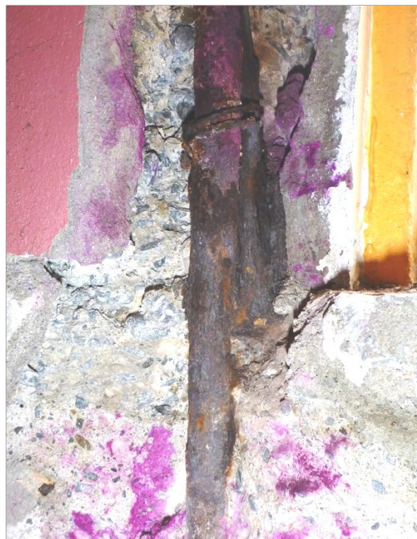
Figure 14. Exposed reinforcement responsible for spall in Figure 13(i). Cover to the \frac{5}{8} " dia. vertical bar is 47 mm (including plaster layer) but the concrete is rumbly and deficient in cement paste. The purple colour is due to phenolphthalein indicator.
