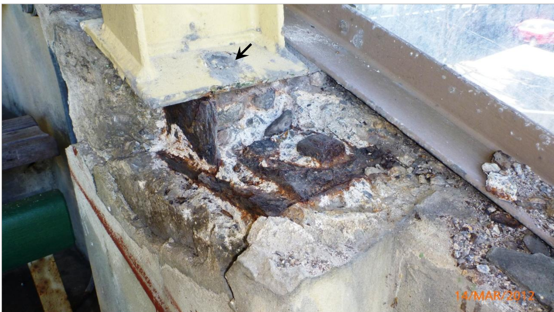
Figure 25. Exploratory breakout of the pedestal showing remnants of the original RSJ and connection to the structural concrete column. Note that the new RSJ is not bolted on this side.
