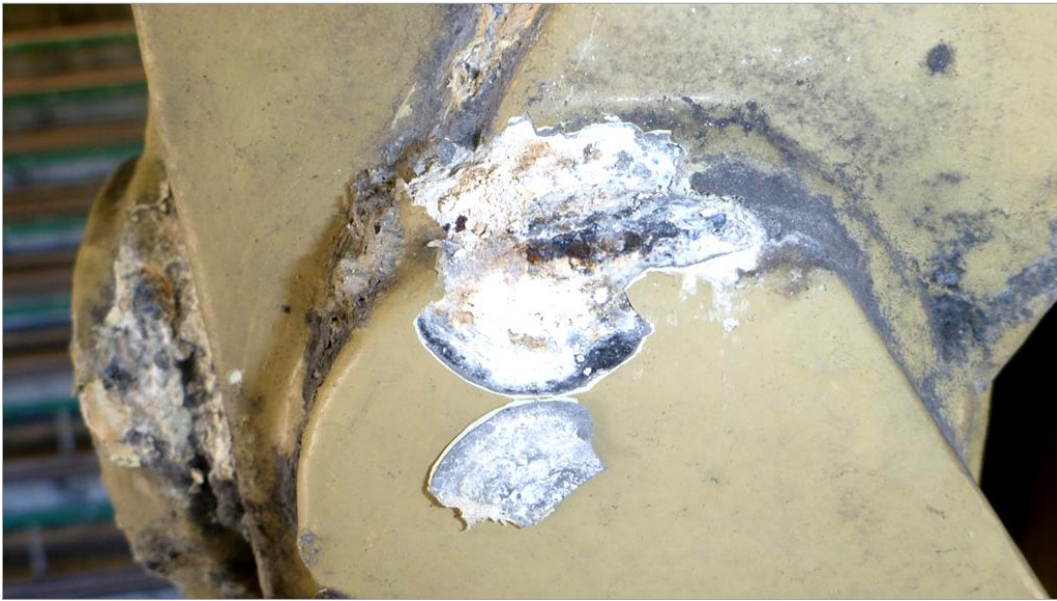
Figure 21. 'White rust' under paint blister, indicating rapid consumption of the hot-dip galvanising that protects the underlying weld and base steel against corrosion.
