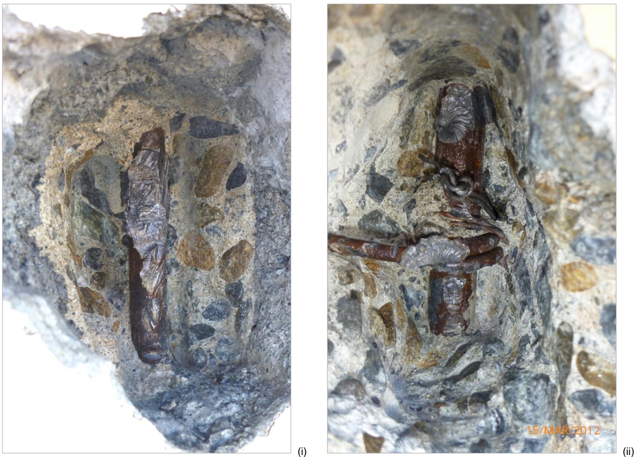
Figure 8. Condition of reinforcement in sound concrete: (i) \frac{3}{8} " diameter bar in middle of wall panel between Bay 2 windows and (ii) \frac{5}{8} " diameter bar with \frac{3}{16} " stirrup in adjacent perimeter column C27. Both bars display faint signs of active corrosion, suggesting they have been depassivated.
