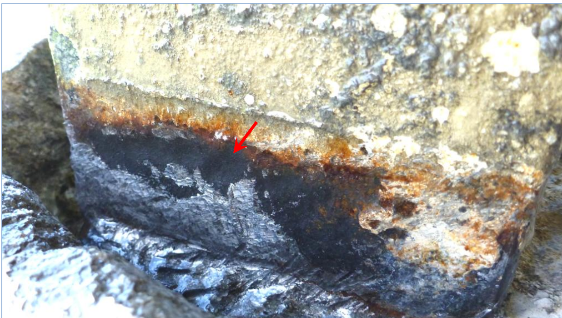
Figure 23. Narrow band of pitting corrosion present on column angles where they are embedded in a concrete pedestal. The arrowed pit is approximately 2 mm deep.
