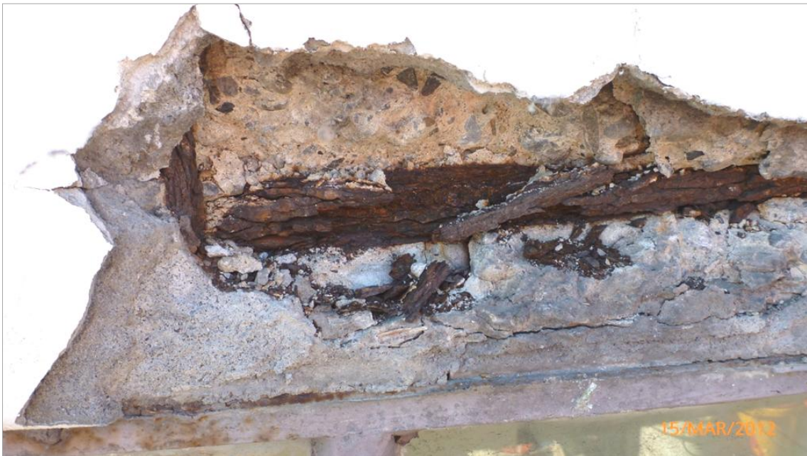
Figure 4. Completely corroded lintel bar above ground floor window (2 nd bay from North). Note that aside from the plaster render, there is minimal protective concrete cover to this bar.
