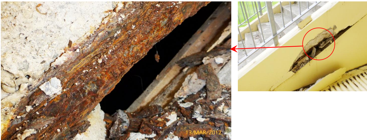
Figure 10. Spall on the inner spring beam of the northern stand access stairs.
