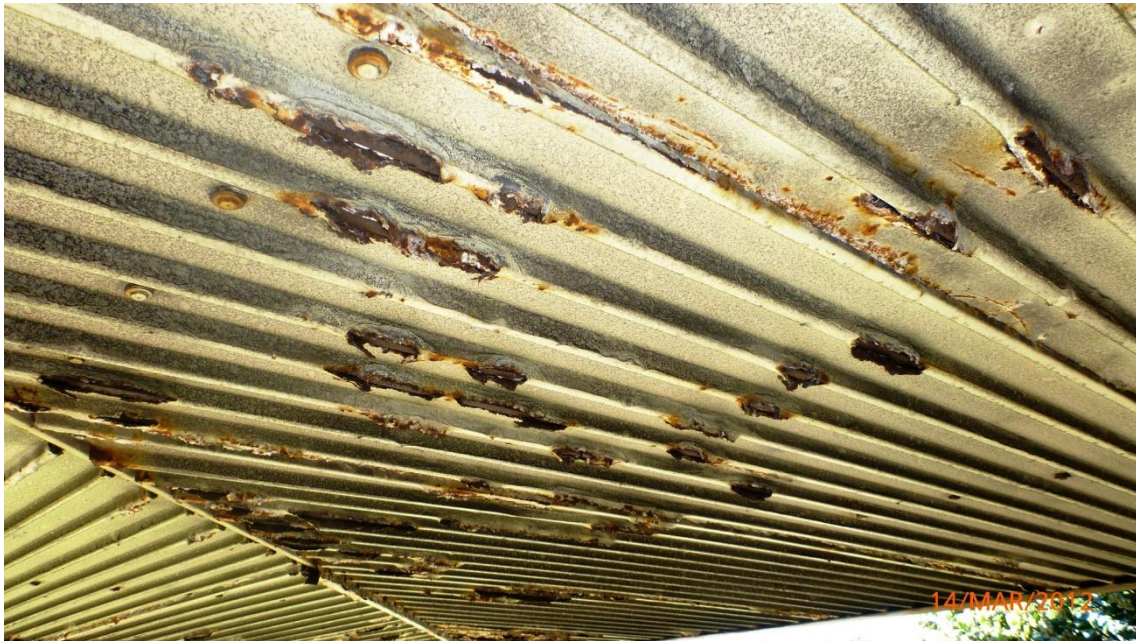
Figure 26. Corrosion of roof soffit lining – southern eave.
