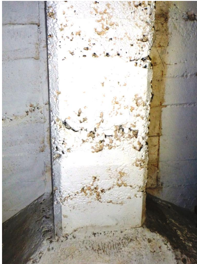
Figure 1. Poor concrete compaction in the base of concrete perimeter column (Sussex Street elevation; basement archive room).
