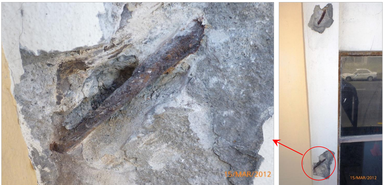
Figure 7. Exploratory breakout of spalls adjacent to the left side of the Bay 3 window reveal. This diagonal hoop reinforcement appears to tie vertical trim bars around the window openings into the main column reinforcement. The original bar diameter appears to be 1/2" but loss of section due to corrosion in the worst area approaches 50%. The bar is almost on the surface of the concrete, directly below the plaster system.
