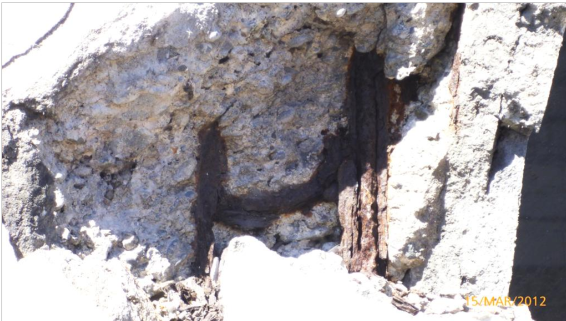
Figure 6. Corroding bars exposed at spall adjacent to Bay 9 gallery window (refer to Figure 2(i) for view of spall prior to breakout). The reinforcement is embedded in loosely-compacted concrete, which has afforded little protection against corrosion.
