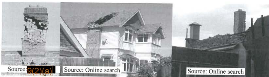
Typical chimney damage (brick chimneys damaged severely)
