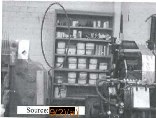
Crack developed in the brick wall behind the rack at the anchor
