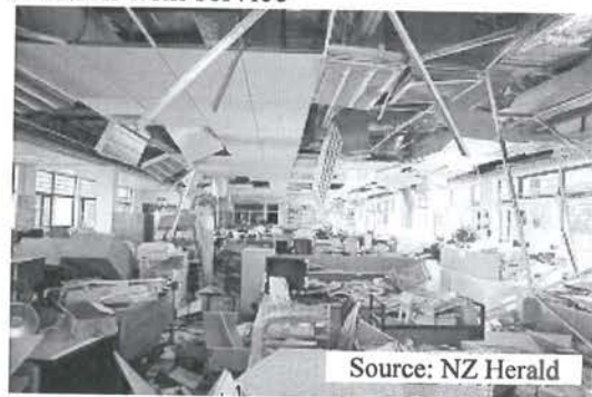
Severely damaged ceiling system
