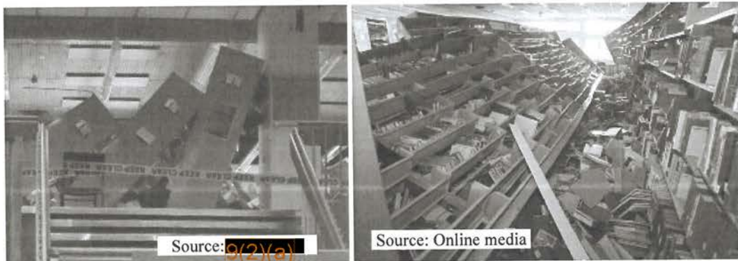
Damage to book shelves in library
