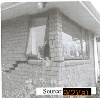
Damage to window and wall
