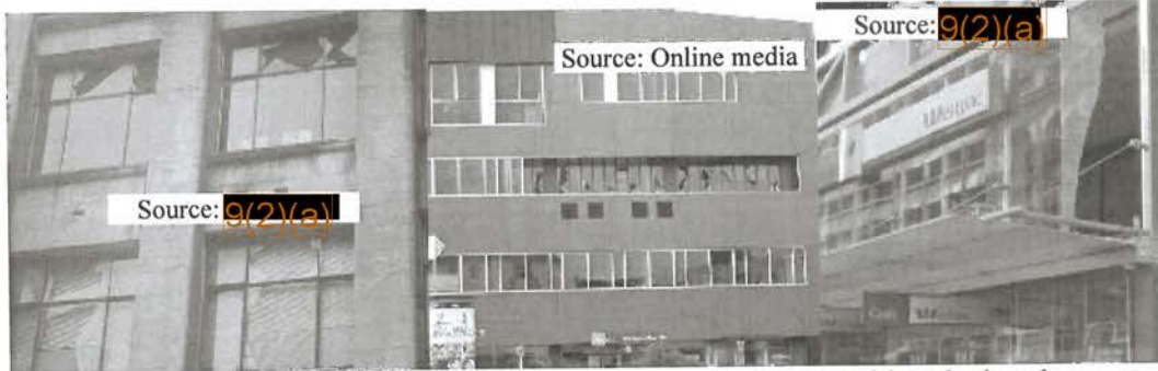
Damage to old glass panels in windows
