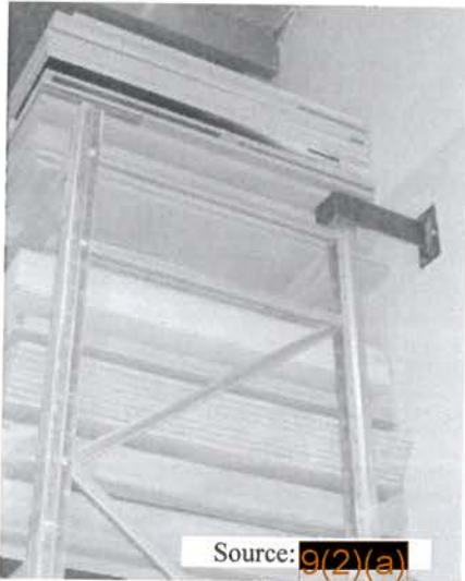
Properly restrained rack with no damage
