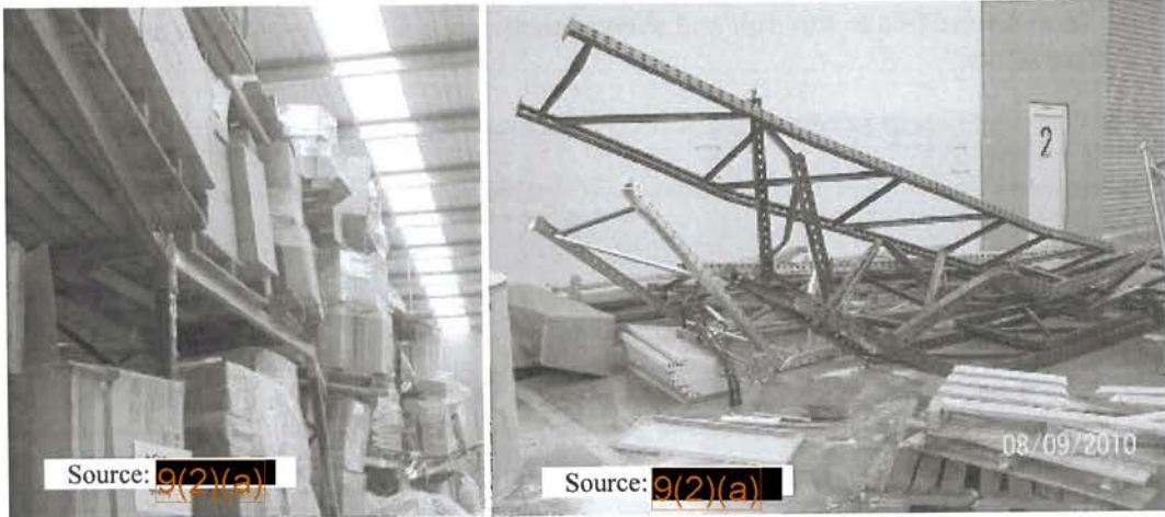
Damaged and collapsed racks at storage facility
