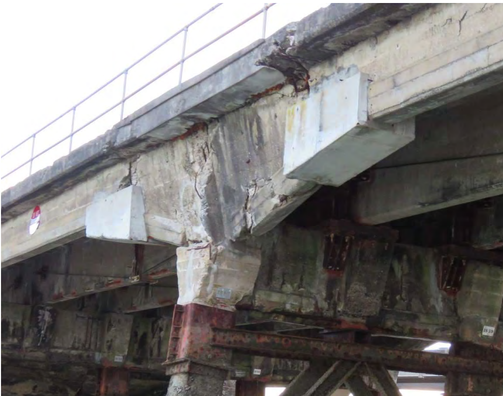
Photo 1 – Pier 15 (Column IS60) impact damage and repairs
