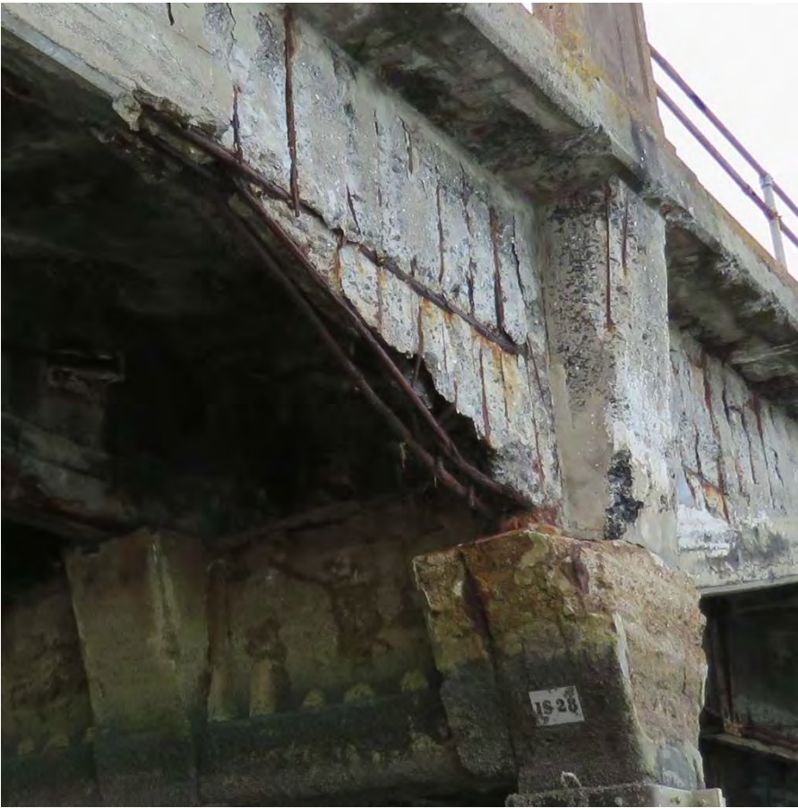
Photo 2 – Pier 7 (Column IS28) loss of concrete and exposed, buckled reinforcing bars
