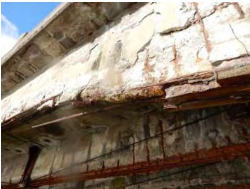
Figure 1: Photo from principal inspection report showing extensive edge girder spalling.
