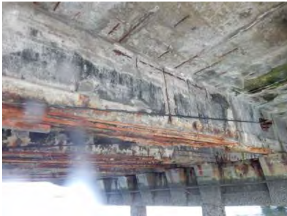
Figure 2: Photo from principal inspection report showing extensive spalling of internal girder.
