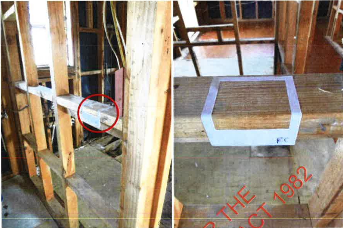
Toilet room framing: methamphetamine was detected on this surface at 0.07 \mu\text{g}/100\text{cm}^2 .
