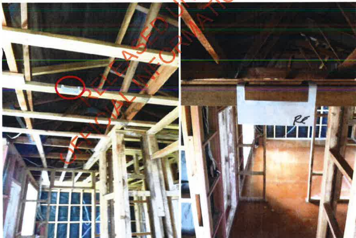
Living room 2 ceiling framing: methamphetamine was detected on this surface at a trace concentration.
