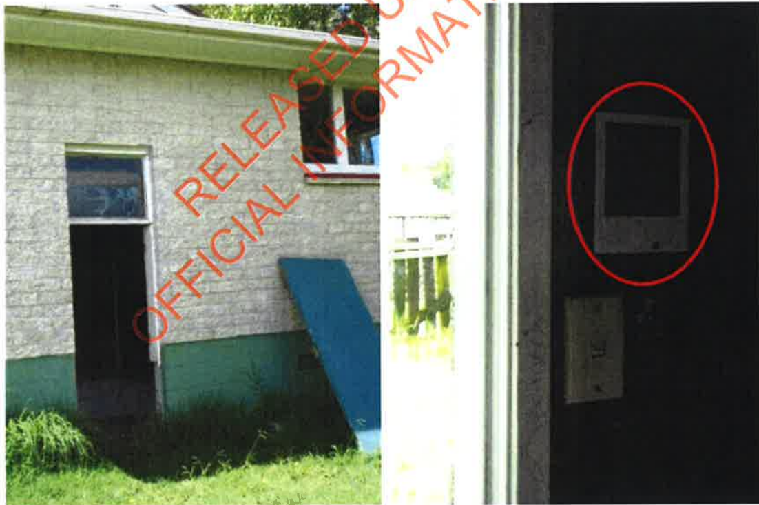
Storage room wall: methamphetamine was detected on this surface at a trace concentration.
