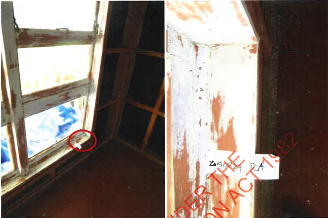
Living room 1 window sill: methamphetamine was detected on this surface at 0.30 \mu\text{g}/100\text{cm}^2 .
