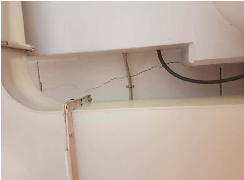
Figure 6 – Transverse crack to hollowcore ground floor unit. CDS A damage.
